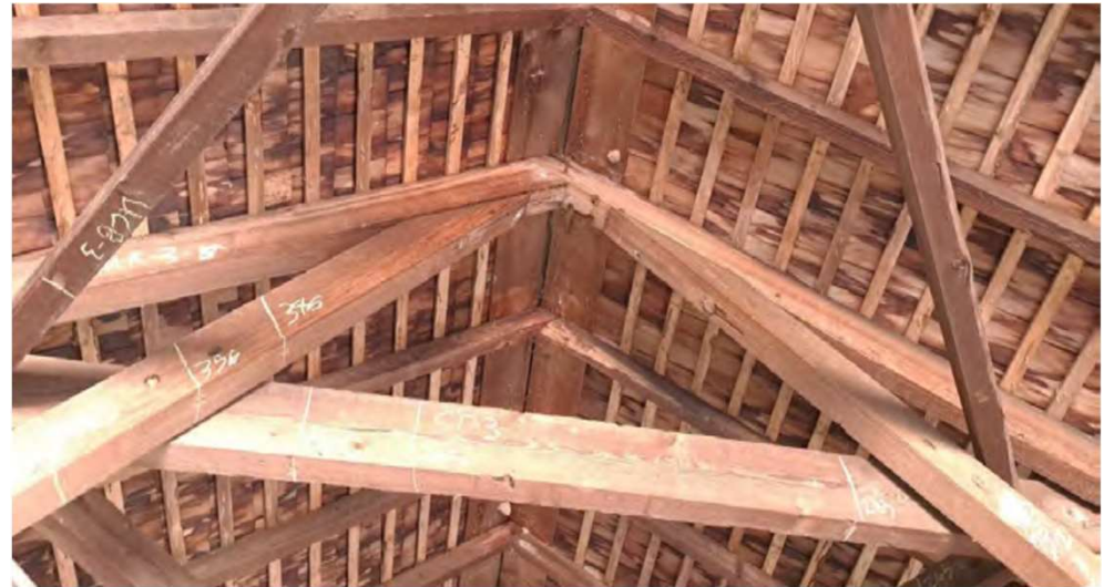
Knee braces KN3-N and KB3-S are out of alignment with CT3. KN3-S has separated from the main rafter R2N-3.
