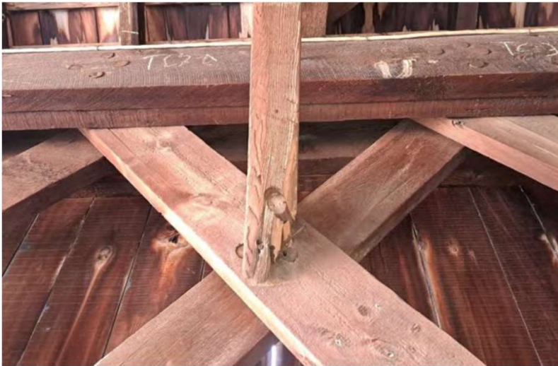
Broken / cleaved dowel connection at knee brace KN2-S.
