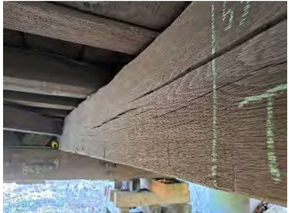
Moderate shrinkage checks in a transverse beam
