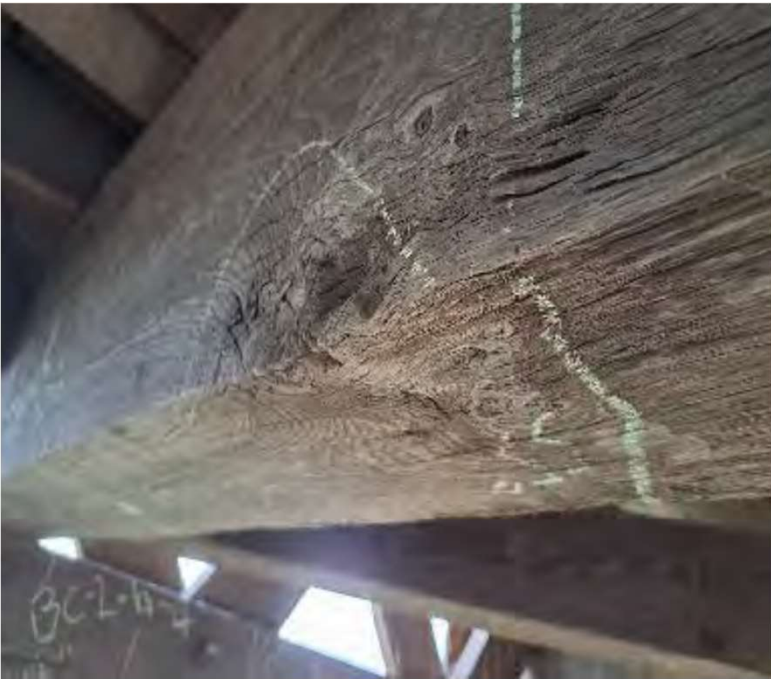
Knot in Transverse Beam
