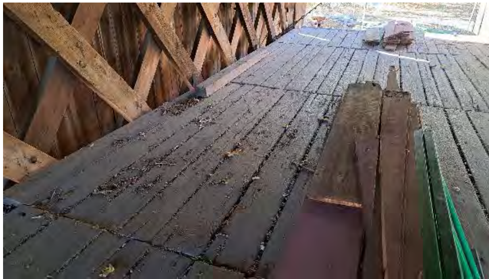
Figure 9-16: Floor decking Span 7, South side.
