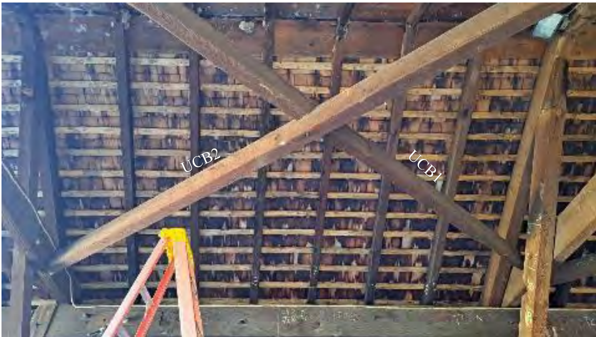
Figure 7-8: Upper cross braces UCB1 and UCB2 are in fair condition.
