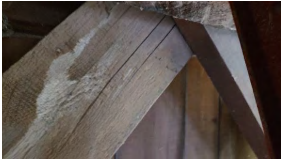
Figure 8-106: L4-20 has split extending from the dowels at the top chord.
