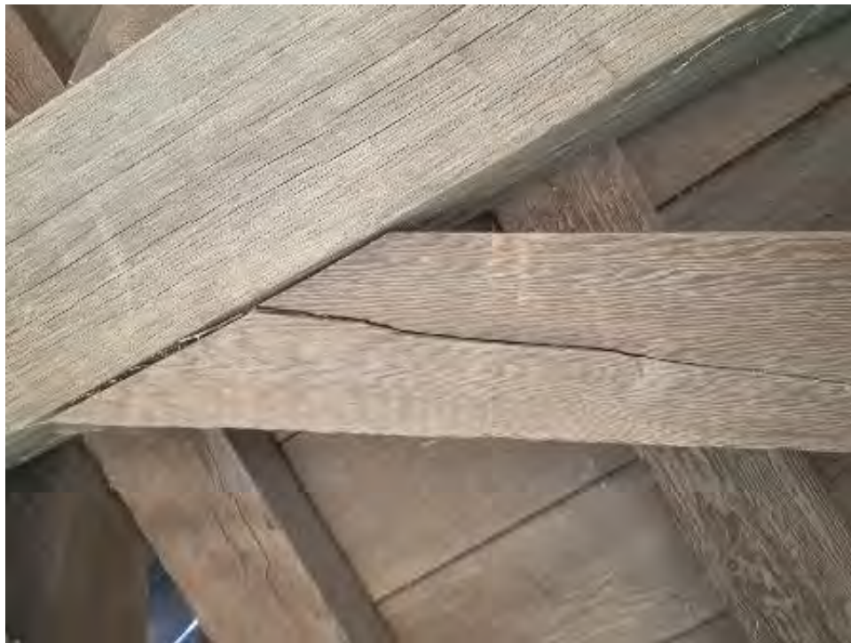
Figure 9-296: LCB-18 major cracking / cleaving of dowel at TB-10. Crack 2-foot long on Abutment 2 face, meets vertical crack on bottom face.
