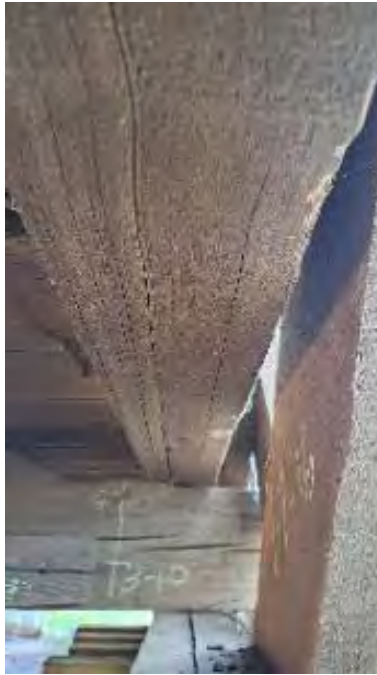
Figure 9-216: J9-1 has a vertical end split from TB10 (24-inches long) and is twisted 4 degrees at the TB10 end, possibly due to the end split and uneven bearing surface. Bearing only on the North edge at TB9.
