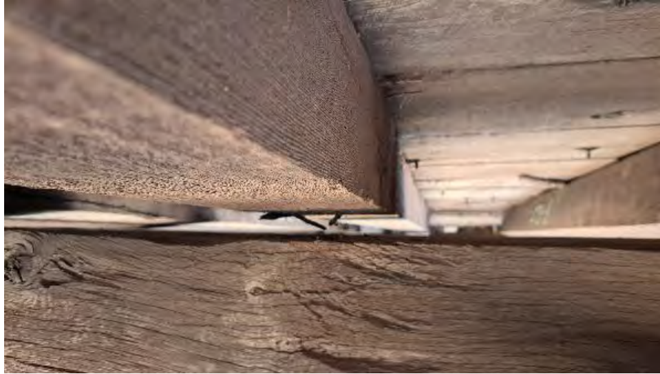
Figure 9-229: J9-7 is not bearing onto TB9.
