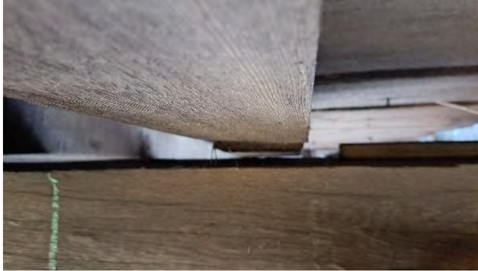
Figure 9-210: J8-7 is not bearing over TB9.
