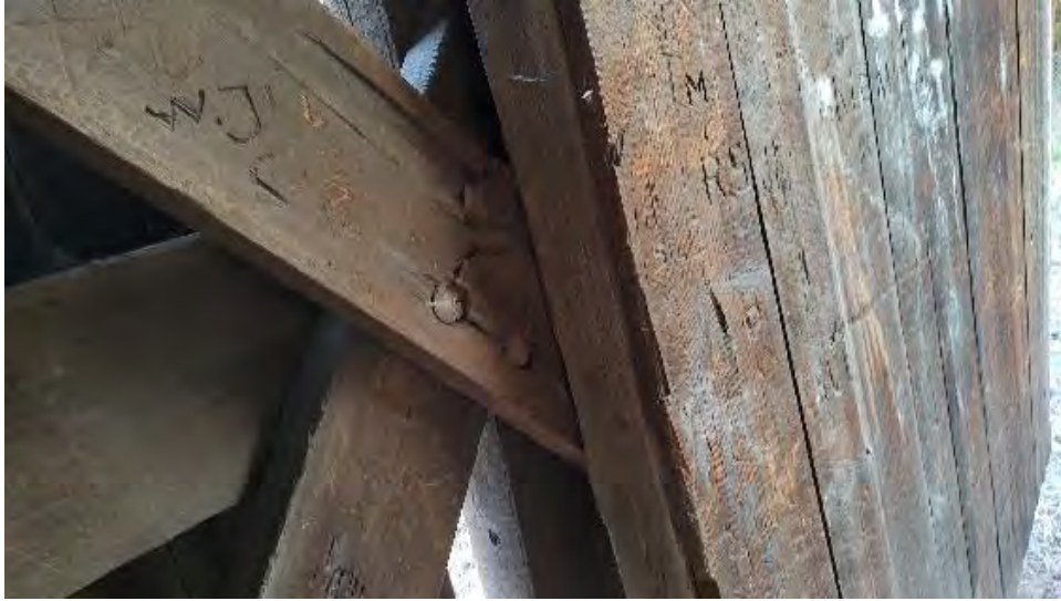
Figure 8-89: L3-21 is broken at the L4-21 connection to P7.
