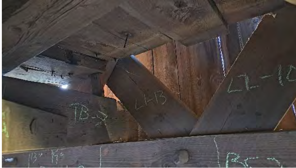
Figure 9-166: J6-1 is missing.
