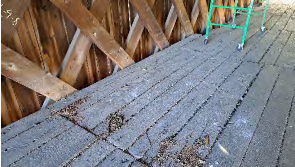
Figure 9-9: Floor decking Span 4, South side.
