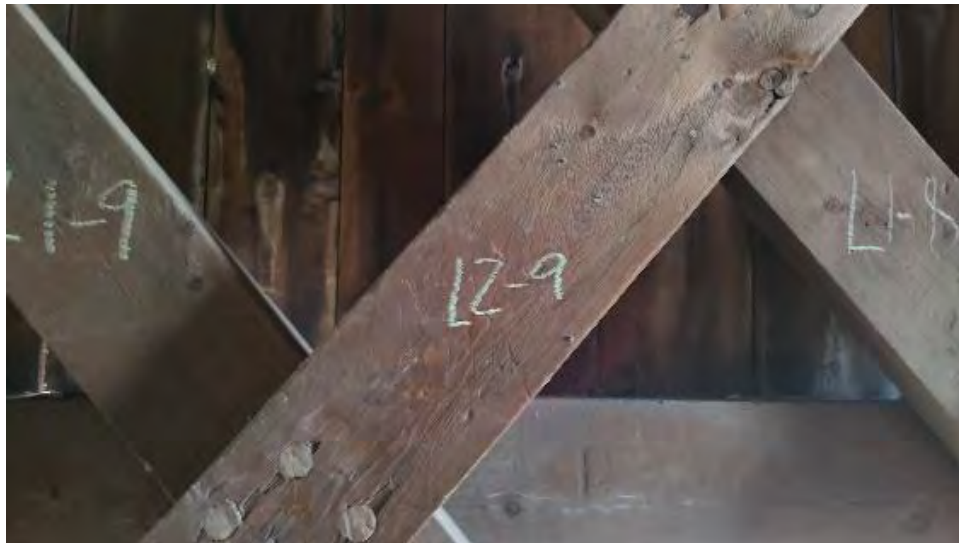
Figure 8-62: L2-9 is cracked at the dowel connection to L1-8.
