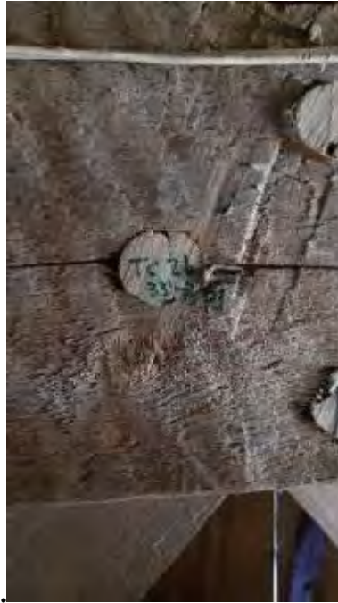
Figure 8-2: TC2B is crack through dowels located 33-feet from post P1.
