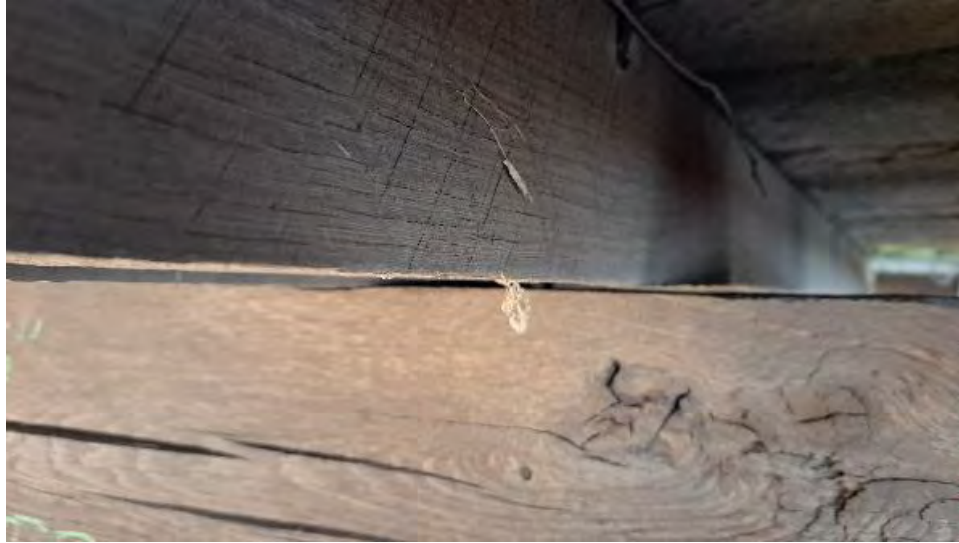
Figure 9-221: J9-3-N minor twisting with no bearing on TB10.
