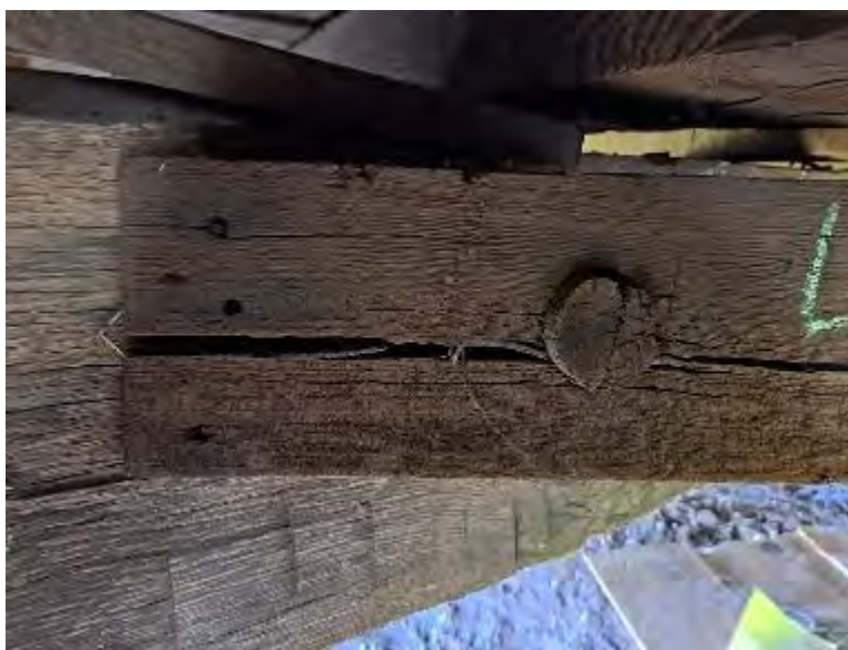
Figure 4-2: End splitting at a lower cross brace at the end connection.
