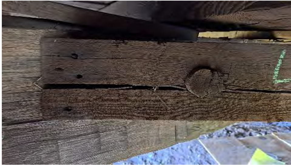
Figure 9-279: LCB-9-A has cleaved on the dowel to TB6.
