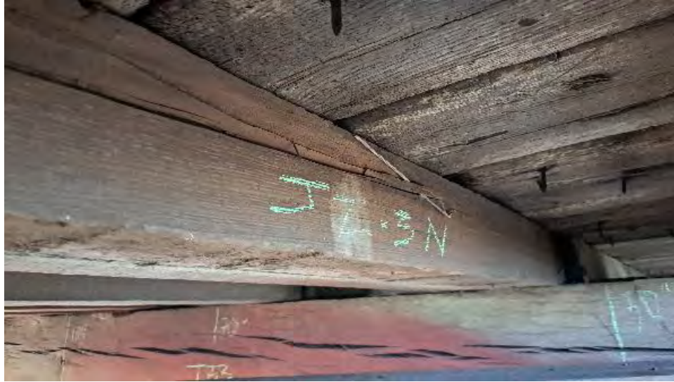
Figure 9-96: J2-3-N has a large split on the North side which extends from the lower corner at TB2 to approximately 12-inches from TB3 at 1/3 from the top edge.
