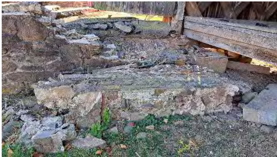
Figure 10-2: The North side of AB1 has approximately 10-foot of stone wall that is dislodged. Backfilling has receded and asphalt surface is damaged.
