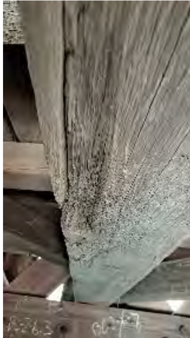
Figure 9-40: TB5 has a slope of grain crack on the AB2 side at 1/3 span from the North end with some section loss in bottom face. Planer skips and chisel scars are on all visible sides.
