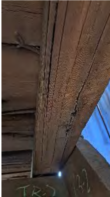
Figure 9-108: J2-8 has vertical cracks to the bottom face, extending to the North side.
