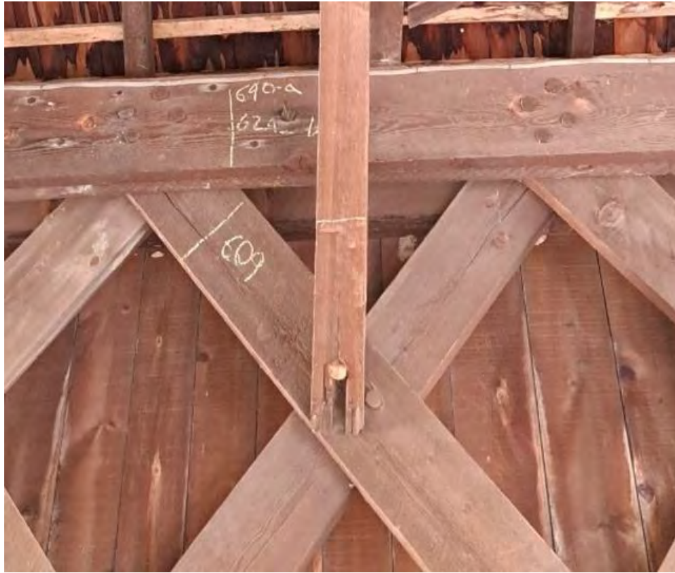
Figure 7-5: KB5-S is cleaved at the lower dowel with section loss below the dowel.
