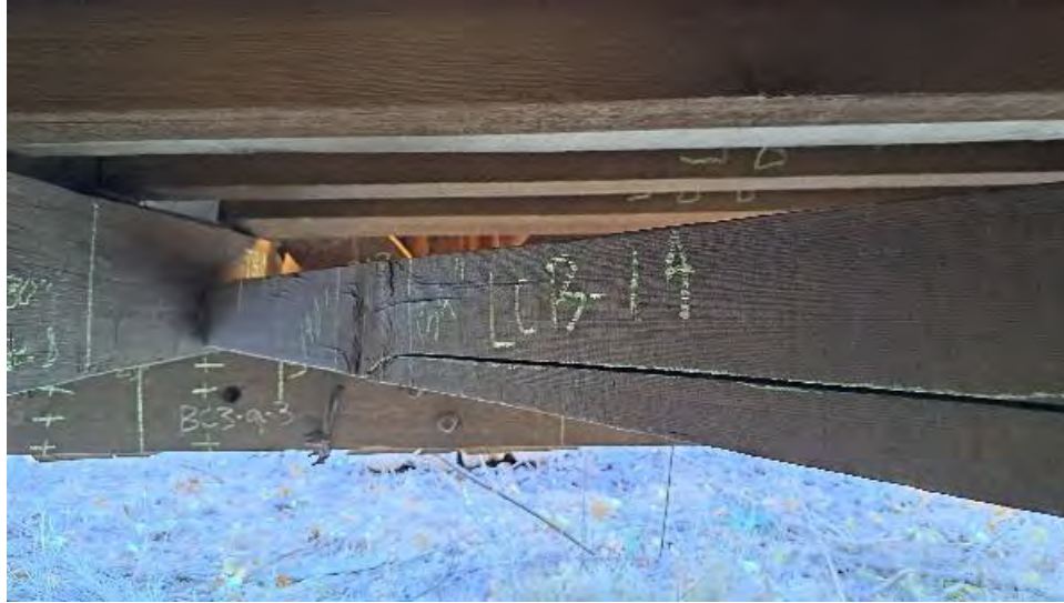
Figure 9-287: LCB-14 has a large knot on the AB1 side that has led to slope of grain cracking.
