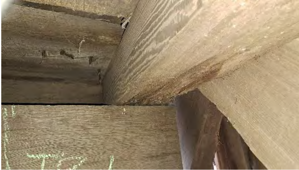
Figure 9-88: J1-8 has decay and section loss to the bottom face for 18-inches from the AB1 end.
