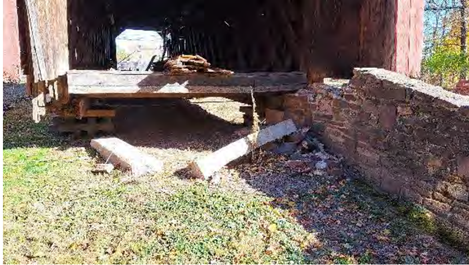
Figure 10-23: Concrete masonry wall segments have been dislodged at AB2. These may have formed the breastwall between the backfill and the timber deck,
