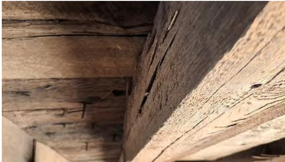
Figure 9-123: J3-6-N has a large end split at TB3 end. The North half is broken.
