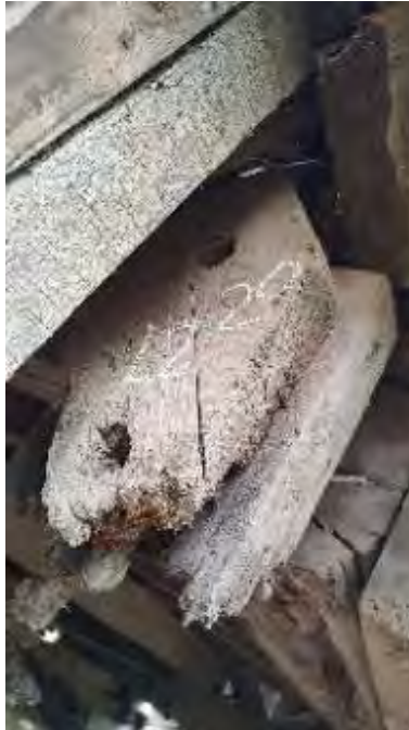
Figure 8-115: The bottom 16-inches of P6 are missing and the next 10-inches are decayed.
