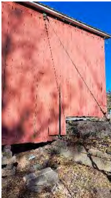
Figure 6-17: South side has some section loss and deterioration on the bottom of the wing wall siding at Abutment 1.
