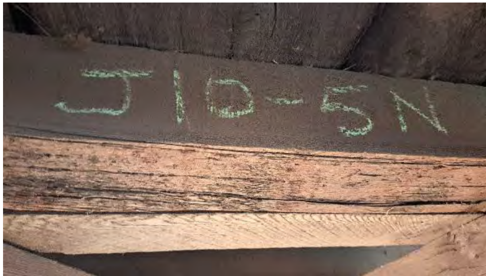
Figure 9-239: J10-5-N has heavy abrasion/section loss to bottom face with significant discontinuity of fiber.
