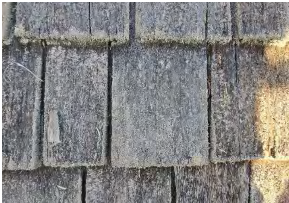
Figure 6-4: Severe weathering, shrinkage and fungal colonies across the roof.
