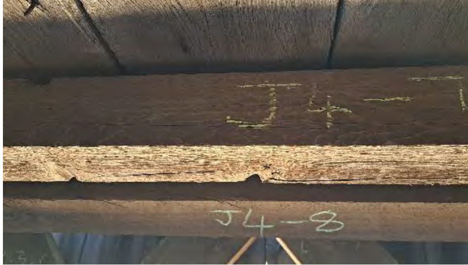
Figure 9-144: J4-7 has two knot holes to the bottom South edge at mid span.
