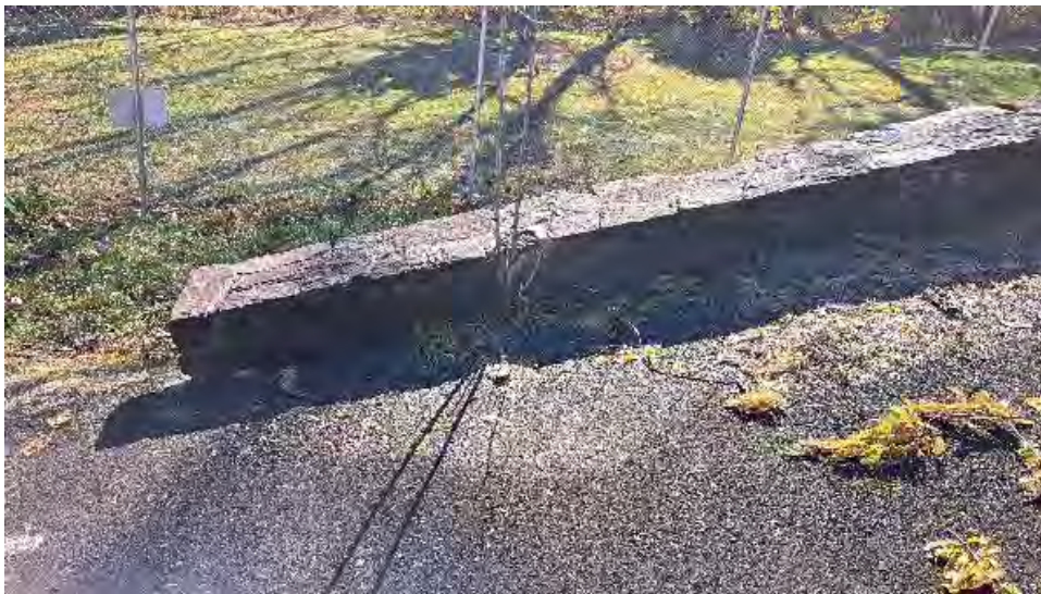
Figure 10-8: Less damage has occurred to the South side stone wall of AB1.
