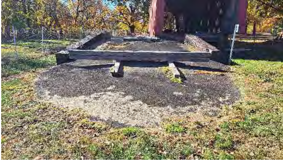
Figure 10-7: A view of the AB1 approach indicates the bridge has moved approximately 10-feet toward the North.
