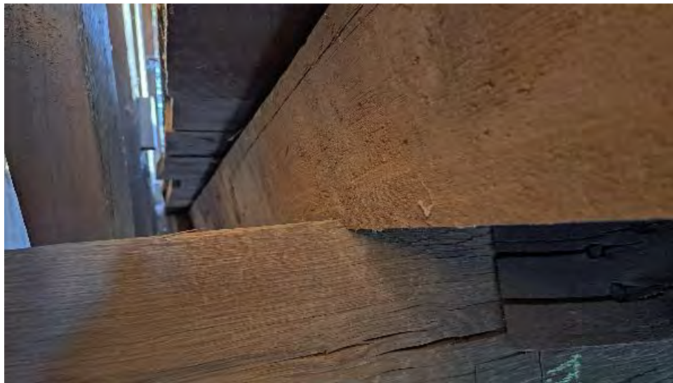
Figure 9-215: J8-8 has twisted about 15 degrees at TB9, resulting in crushing of the TB9 and J8-8 interface.
