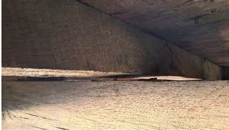
Figure 9-159: J5-6 is twisted 9 degrees over TB5 with no bearing over TB5 or TB6.
