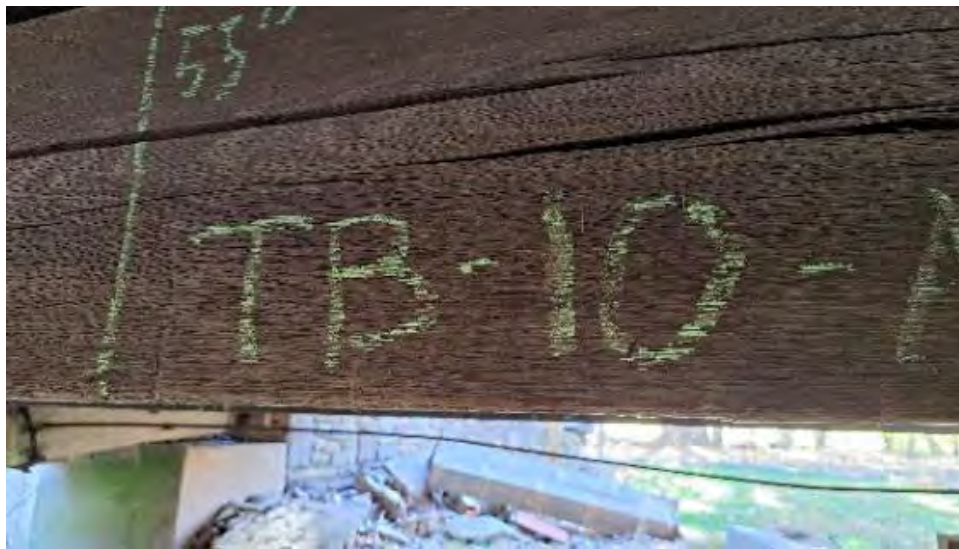
Figure 9-59: TB10 has shrinkage checks 2-inches deep and 3/8-inches wide on the AB1 side, North end.
