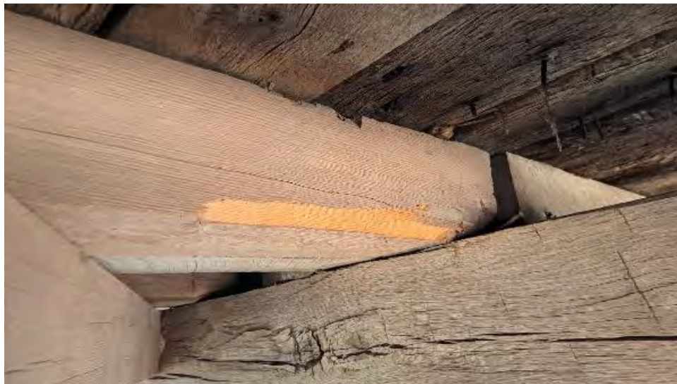
Figure 9-117: J3-3-S has wane and section loss on its South edge at TB3.
