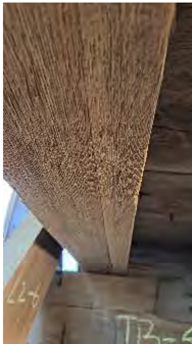
Figure 9-133: J4-1 has a bottom face split extending from TB4.
