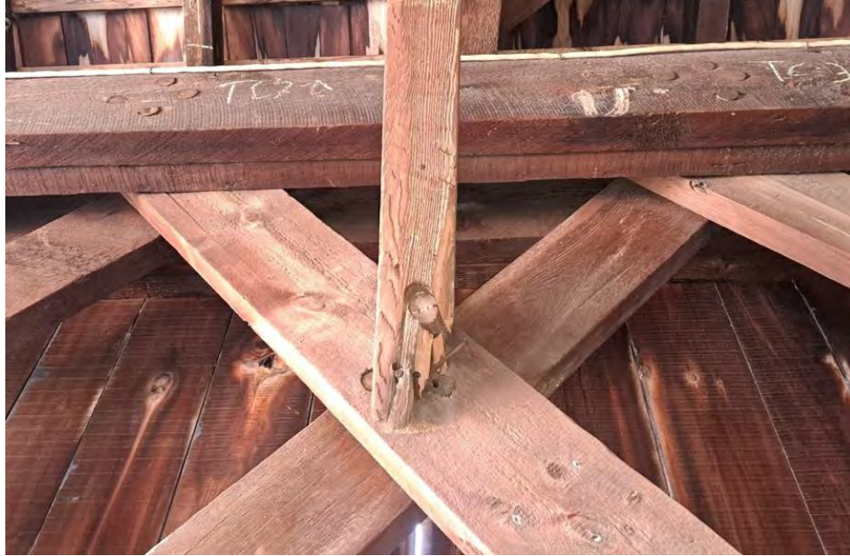
Figure 7-1: Broken / cleaved dowel connection at knee brace KN2-S.
