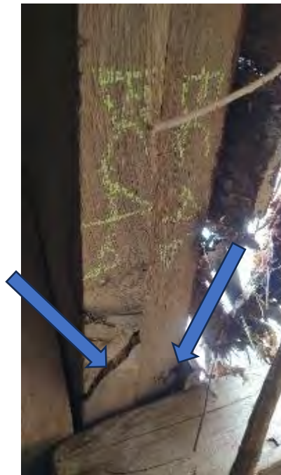
Figure 8-37: BC4A and BC4B are broken at 70-inches from P8.
