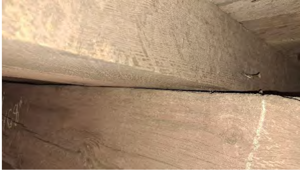
Figure 9-84: J1-6-N is only bearing on the South edge over TB2.
