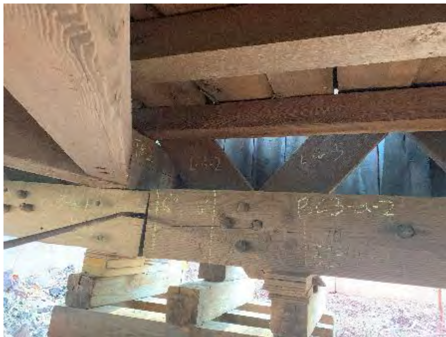
Figure 8-41: Shrinkage checks exist through dowel holes of the BC3A splice.
