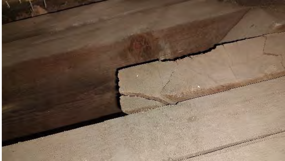
Figure 8-75: L3-6 is split from the dowel connection at the top chord.
