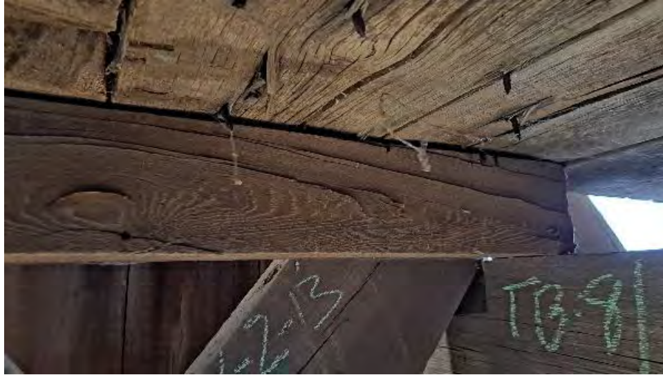
Figure 9-194: J8-1 has a bearing length of 1.5-inches on TB8.
