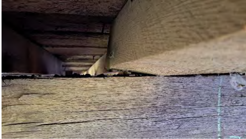
Figure 9-184: J7-4 is only bearing on the South edge at TB7.
