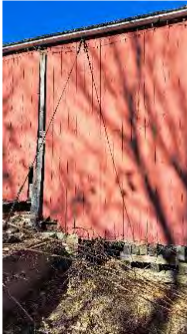
Figure 6-16: Missing boards at Post 8 at Abutment 2 on the South side.
