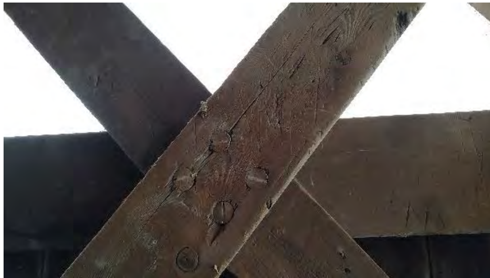
Figure 8-65: L2-17 is cracked at the dowel connection to the middle chord and Lattice 1 member.
