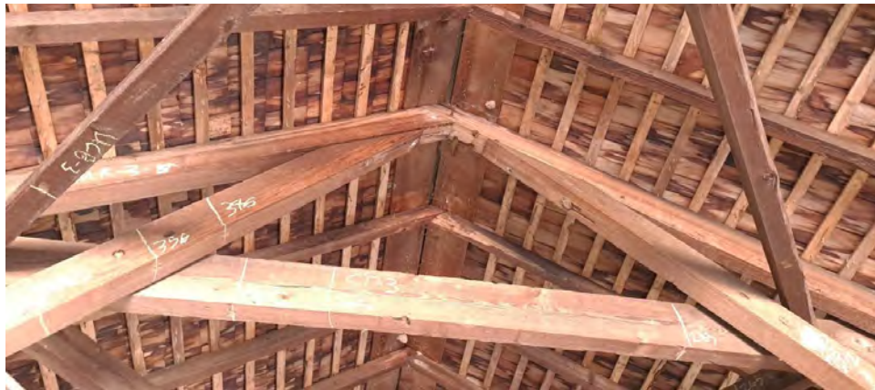
Figure 7-2: Knee braces KN3-N and KB3-S are out of alignment with CT3. KN3-S has separated from the main rafter R2N-3.
