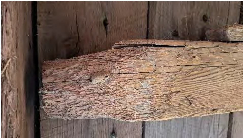
Figure 9-259: J11-7 has termite damage to the bottom and South faces with significant section loss.
