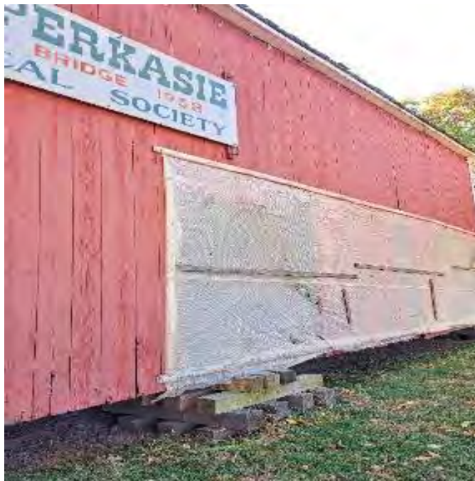
Figure 6-11: Siding on Northwest side showing missing boards in multiple locations behind the temporary plastic wrapping.
