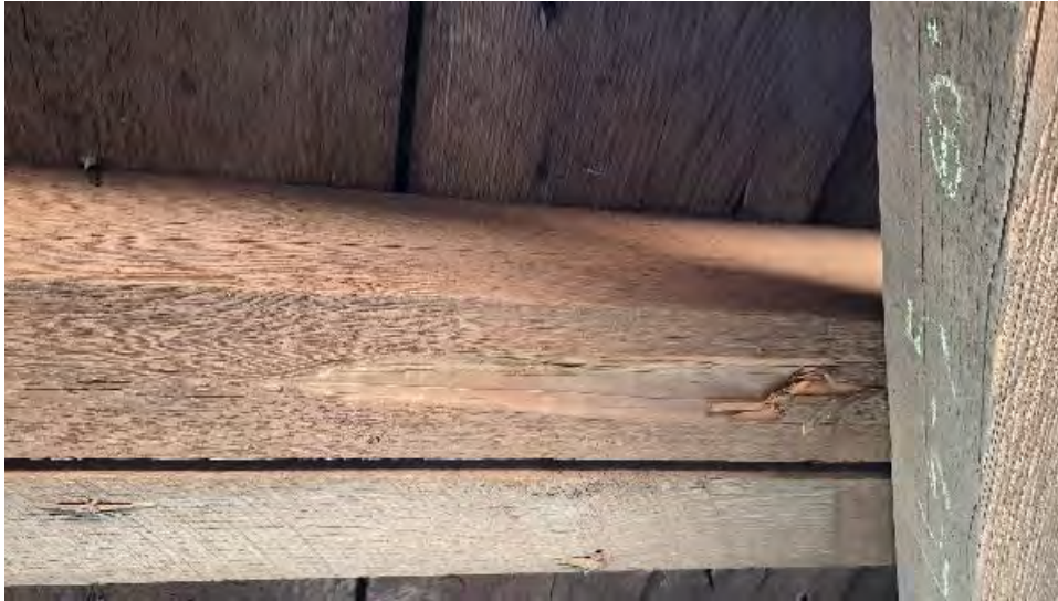
Figure 9-139: J4-3-S has a vertical crack on the bottom face extending from TB4 for 3-feet.
