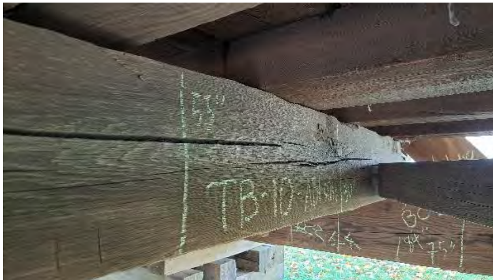
Figure 9-61: TB10 has shrinkage checks 2-inches deep and 3/8-inches wide on the AB1 side, North end.
