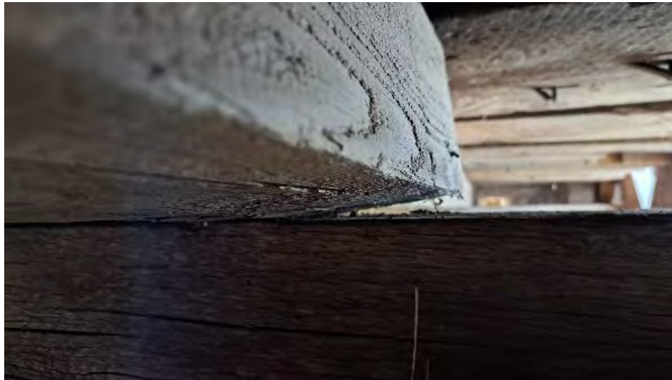
Figure 9-167: J6-2 is partial bearing on its South edge at TB7. J6-2 is twisted by 8 degrees.
