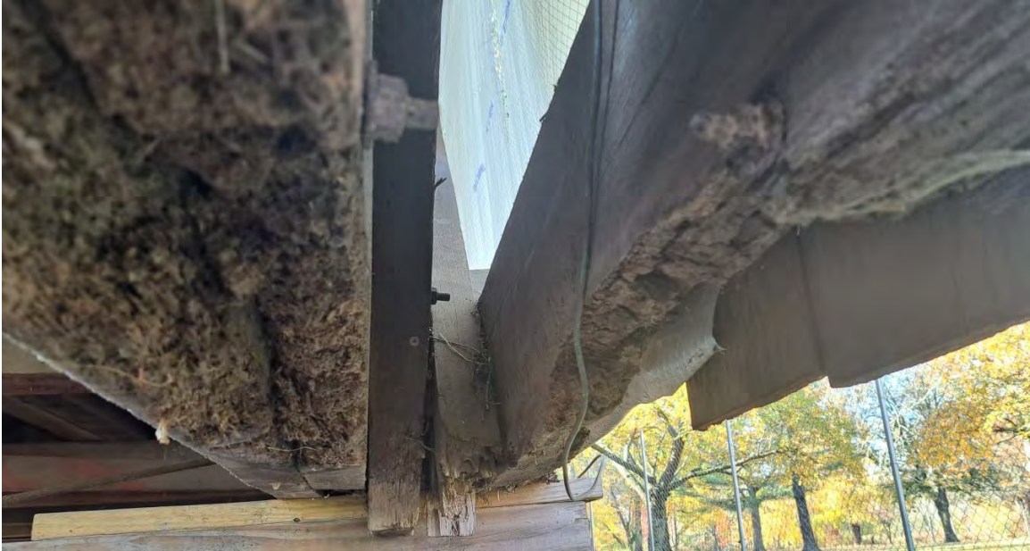
Figure 8-24: The first 40-inches of bottom chord BC1A and BC1B from Post P1 has significant decay and 2-inches section loss on bottom faces. The bottom half of BC1B is decayed/crushed for the first 3-feet from P1. The next 5-feet of the bottom face is decayed/crushed. The bottom third of BC2A is decayed with significant section loss for the first 39-inches from P2. The next 40-inches is crushed on the bottom face for a depth of 1-inch and extends over the cribbing. BC2A is spliced 49-inches from the end. Significant section loss exists for the first 6-inches of BC2B from P2. The next 3-feet is decayed for the bottom third. BC2B is spliced at 6-feet from P2.
