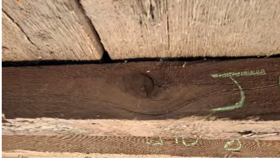
Figure 9-244: J10-7 has a large knot on its North side face near midspan which has led to slope of grain cracking.
