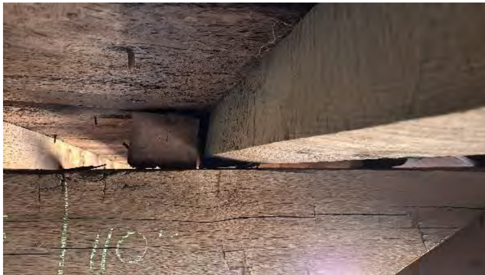
Figure 9-160: J5-6 is twisted 9 degrees over TB5 with no bearing over TB5 or TB6.
