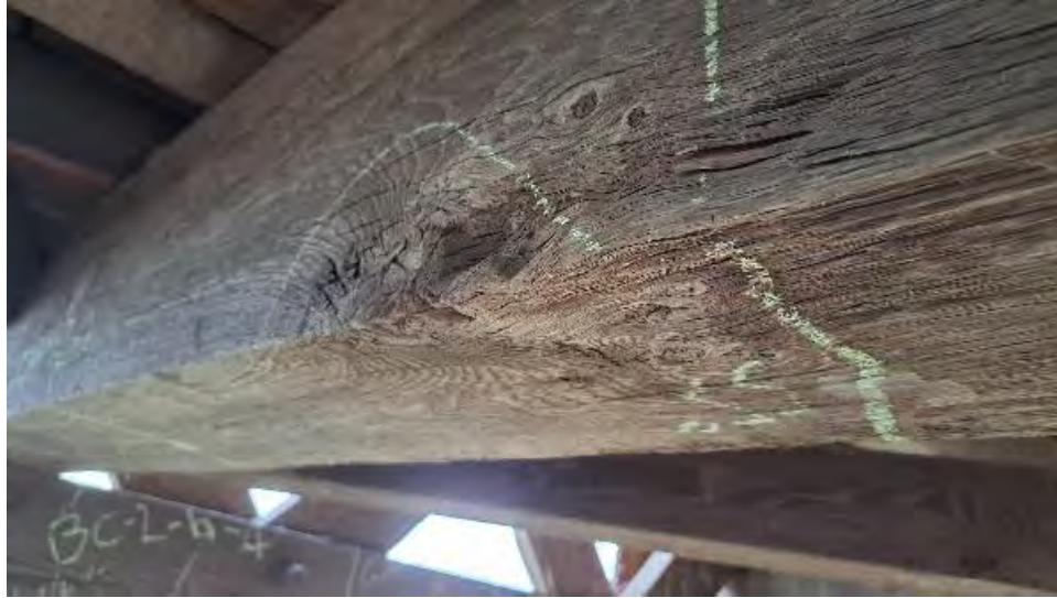
Figure 9-62: TB10 has a large knot to the bottom AB2 edge at 1/3 span location from the North end.
