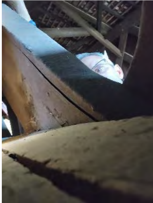
Figure 8-93: L4-2 is cracked either side of the connection to L3-2 and with shrinkage checks through 1 row of dowels.
