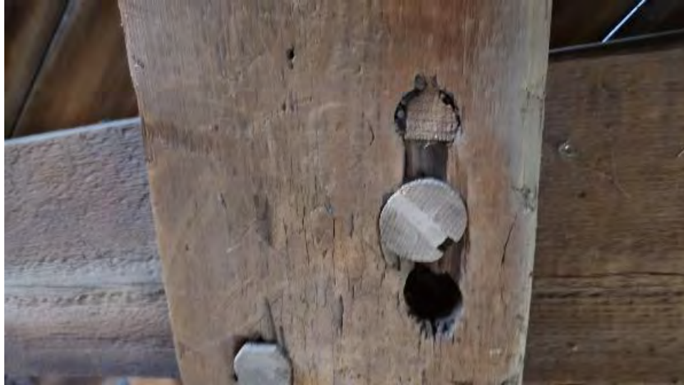
Figure 8-81: Dowel on L3-14 at L4-15 has insufficient distance to adjacent dowel and hole to be effective.
