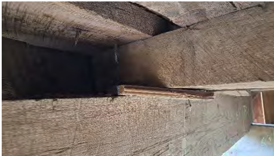
Figure 9-83: J1-6-N is packed above TB1 but is resting on its South edge only over TB2.
