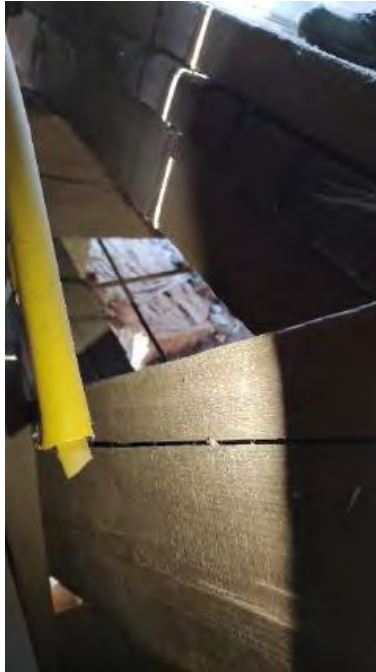
Figure 8-109: L4-22 is broken at the deck level.
