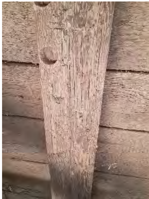
Figure 9-243: J10-7 bottom face with several knots, significant discontinuity of fibers.
