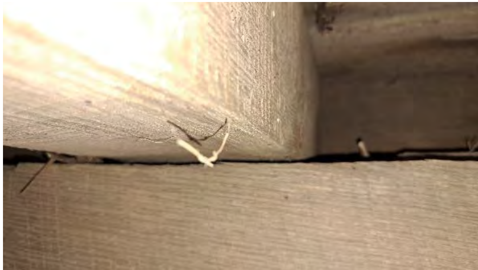
Figure 9-73: J1-2 is not bearing on TB1.
