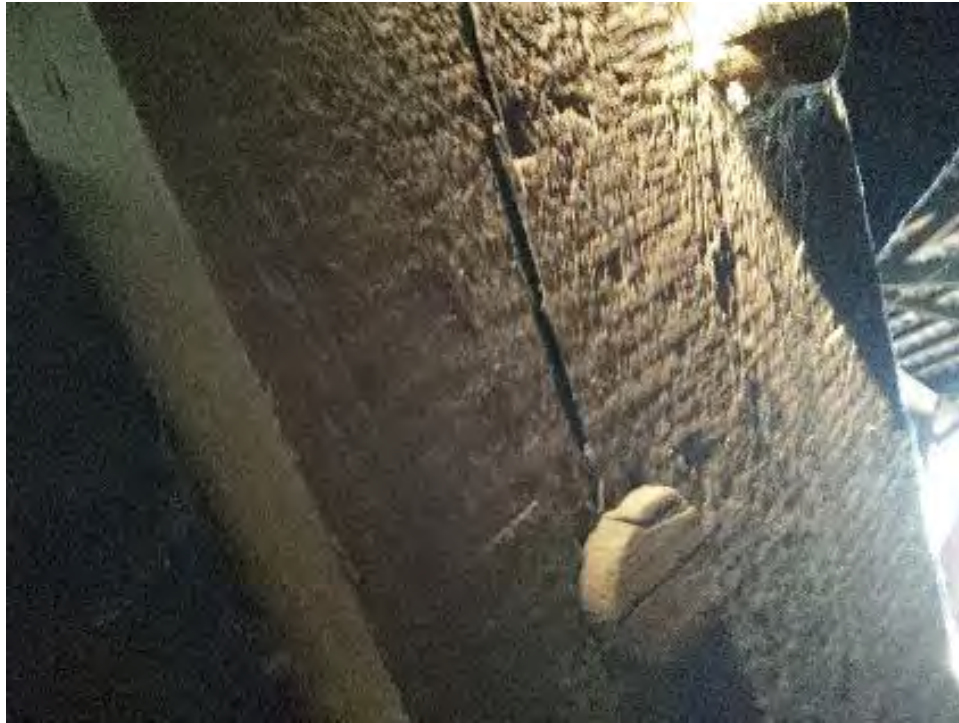
Figure 8-101: L4-12 is cracked through the bottom dowel at L3-11.
