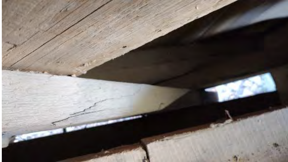
Figure 8-83: L3-16 is cracked below L4-18 towards the bottom.
