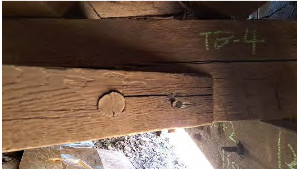
Figure 9-275: LCB-6 has cleaved on the dowel to TB4.
