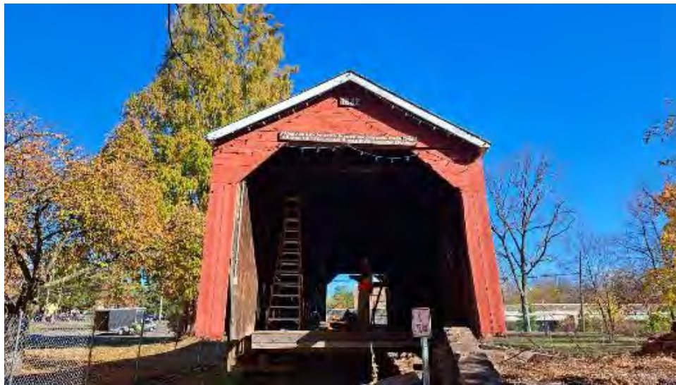
Figure 6-21: Abutment 2 front view of siding.
