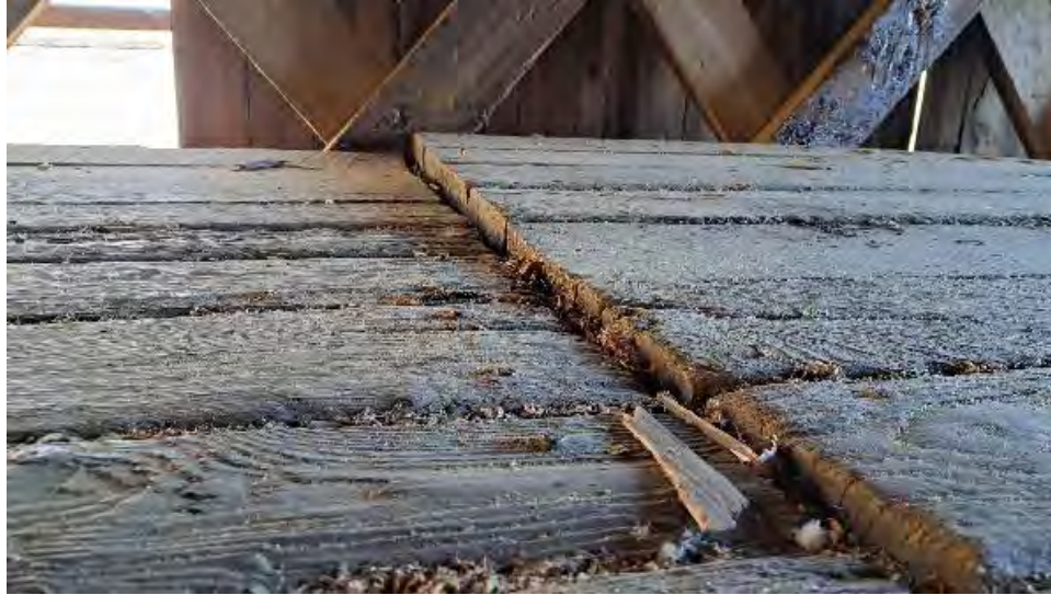
Figure 9-13: The Northwest corner of floor decking Span 5 is raised above Span 4 by 2.5-inches.
