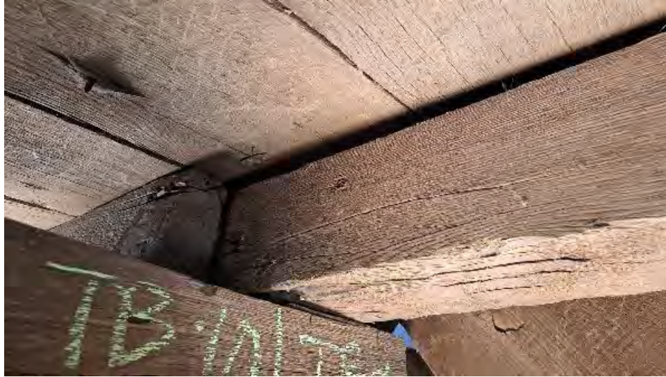
Figure 9-246: J10-8 has section loss at its bearing surface over TB10 and at the top South edge over TB10.
