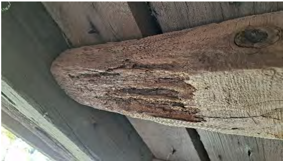
Figure 9-253: J11-4 has some termite damage with major section loss at the bottom face at the AB2 end.
