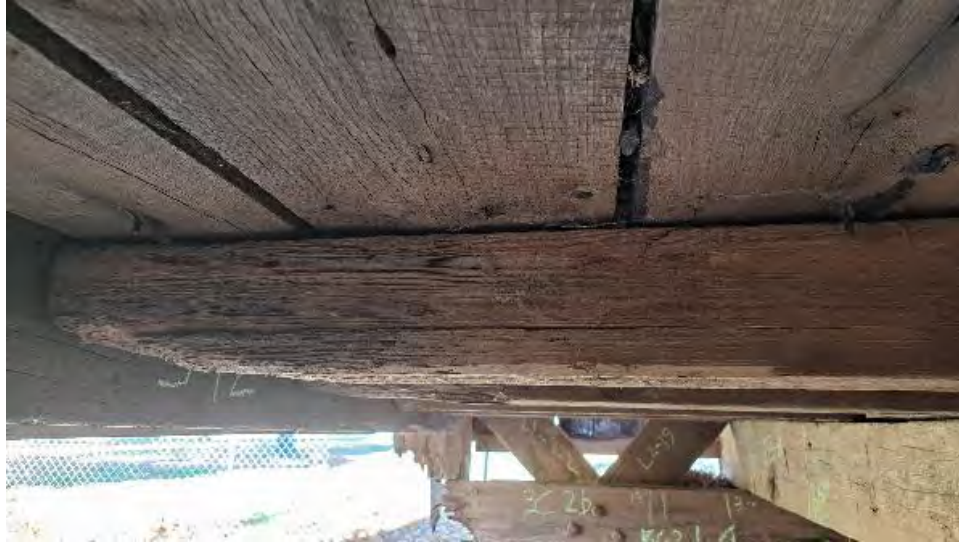
Figure 9-256: J11-5 has an end split on the South face that is 20-inches long.
