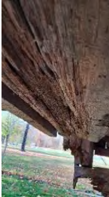
Figure 9-68: JT2 is severely decayed and with section loss on bottom face. A 3-inch-deep cavity exists on the bottom face. JT2 is not currently supported at either end.
