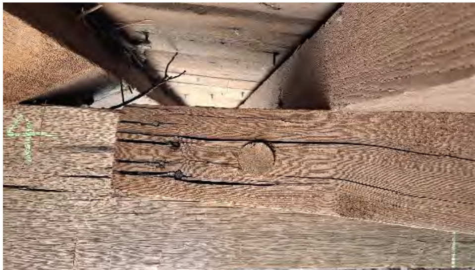
Figure 9-272: The LCB-3 dowel and spikes at TB4 have cleaved.
