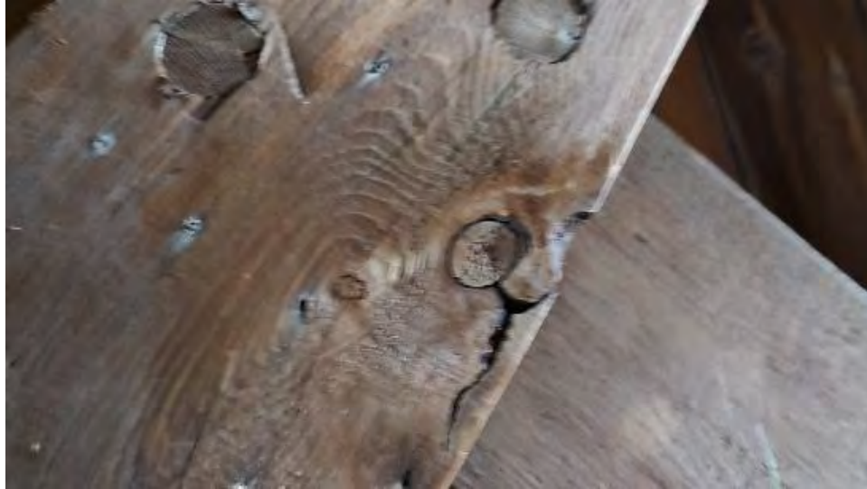
Figure 8-61: L2-9 is cracked at the dowel connection to L1-8.
