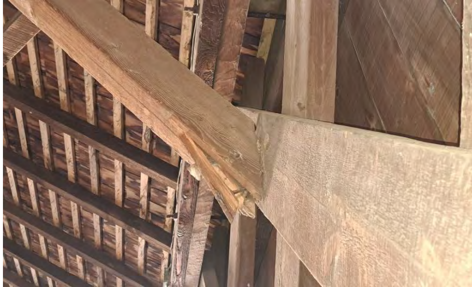
Figure 7-3: Cleaved and broken lower end of knee brace KN4-S.
