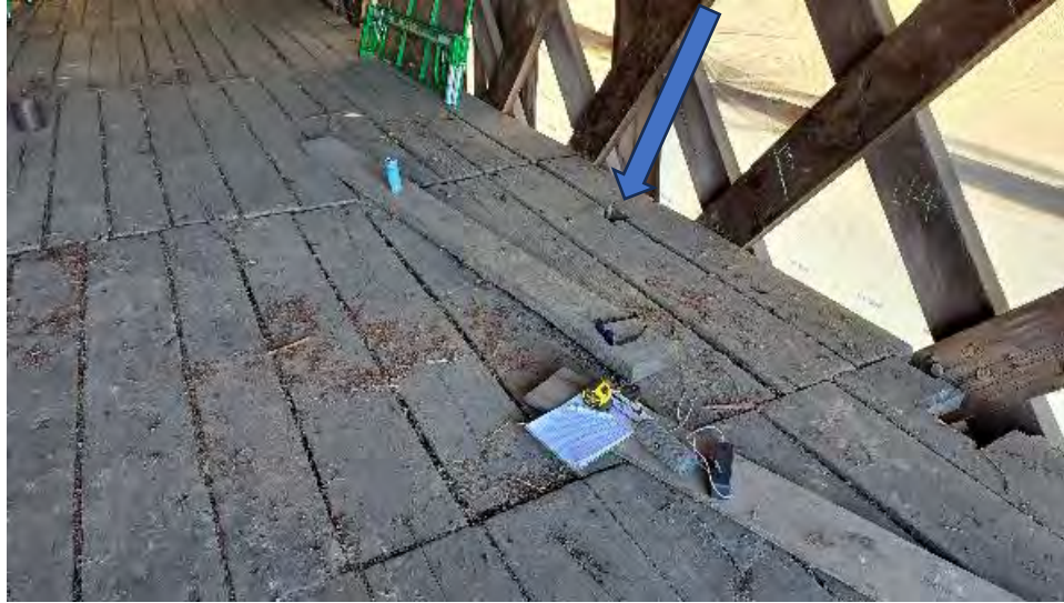
Figure 9-5: Floor decking Span 2 North side, with common hole in Plank 1 and 2.
