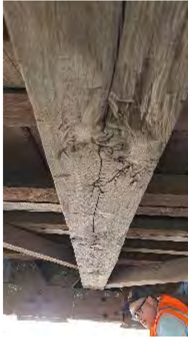
Figure 9-57: TB9 has large knots on the bottom face at 1/3, 1/2, and 2/3 span locations. Planer skips and chisel scars exist on all visible sides. Shrinkage checks exist on the bottom face.
