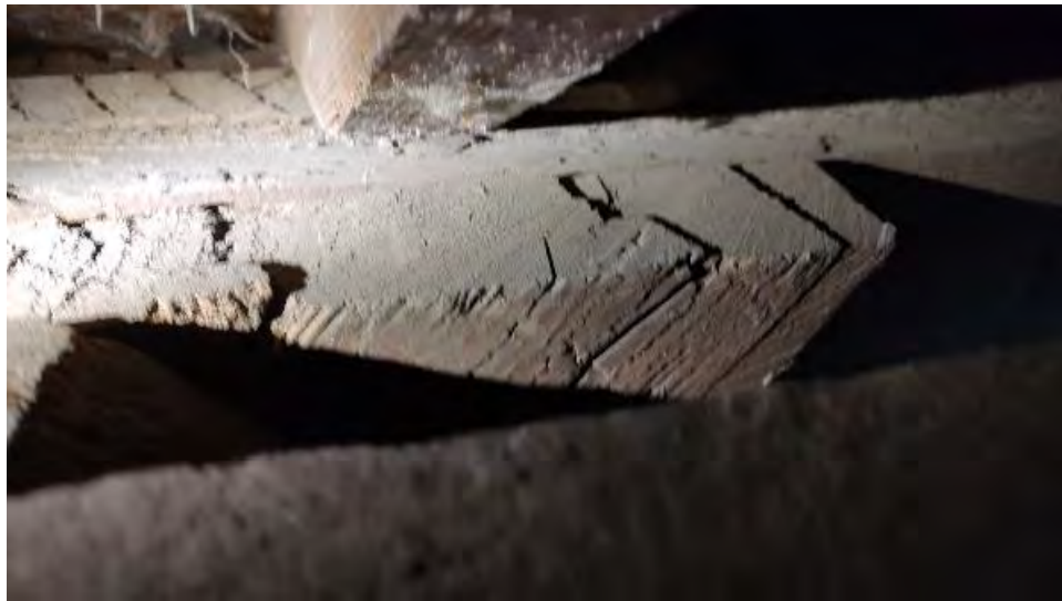
Figure 8-104: L4-16 has split extending from the dowels at the top chord.
