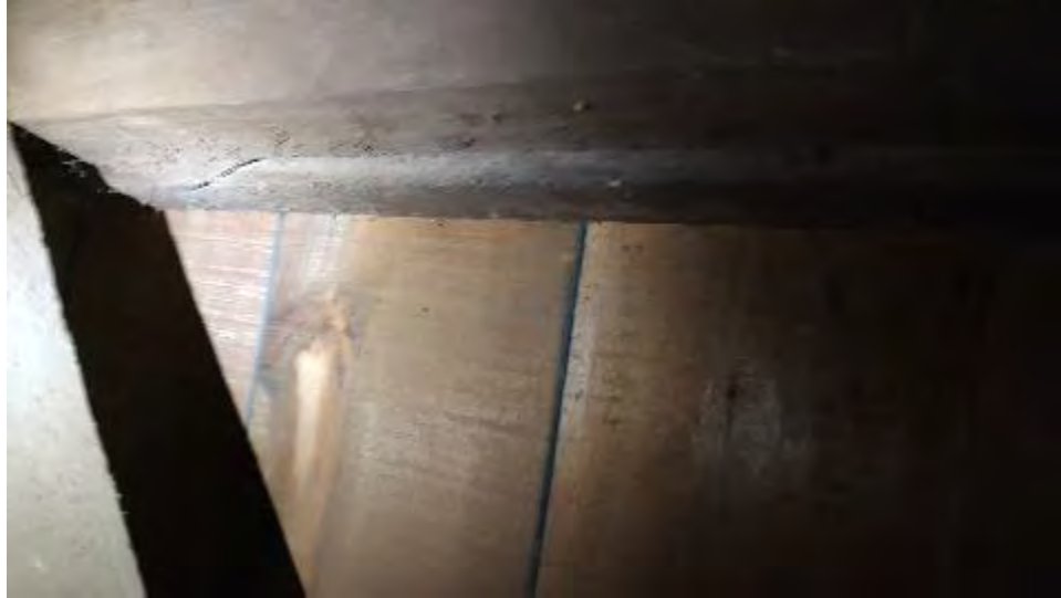
Figure 8-6: The crack in a small section on the bottom face of TC1B does not appear to extend to the top or through the member.
