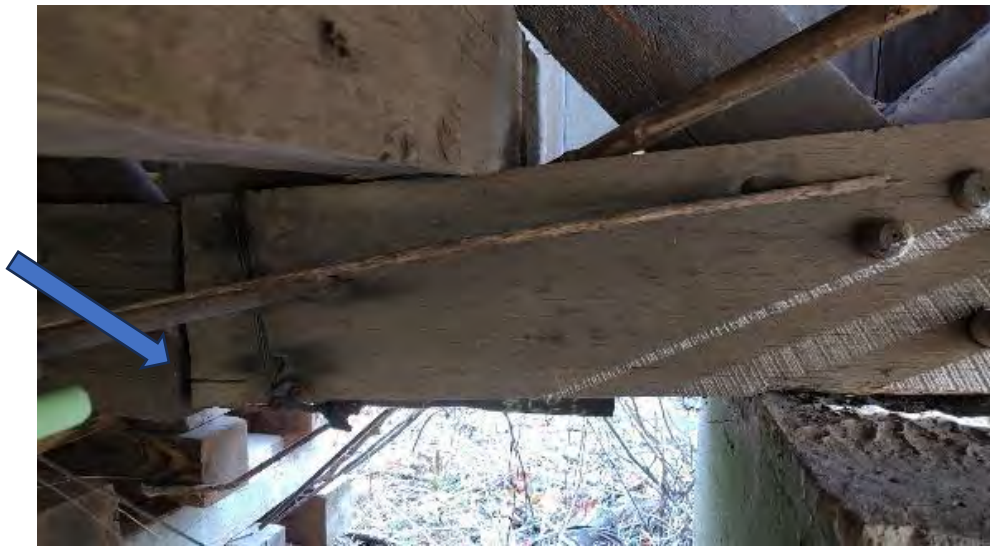
Figure 8-34: The splice of BC3B is broken at 64-inches from P7.
