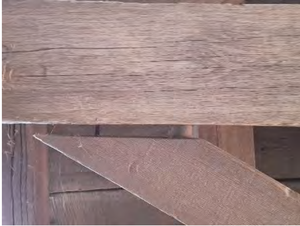
Figure 9-291: LCB-16 is separated from TB 10 by approximately 1-inch.
