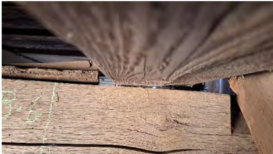
Figure 9-148: J5-1 is not bearing on TB5.
