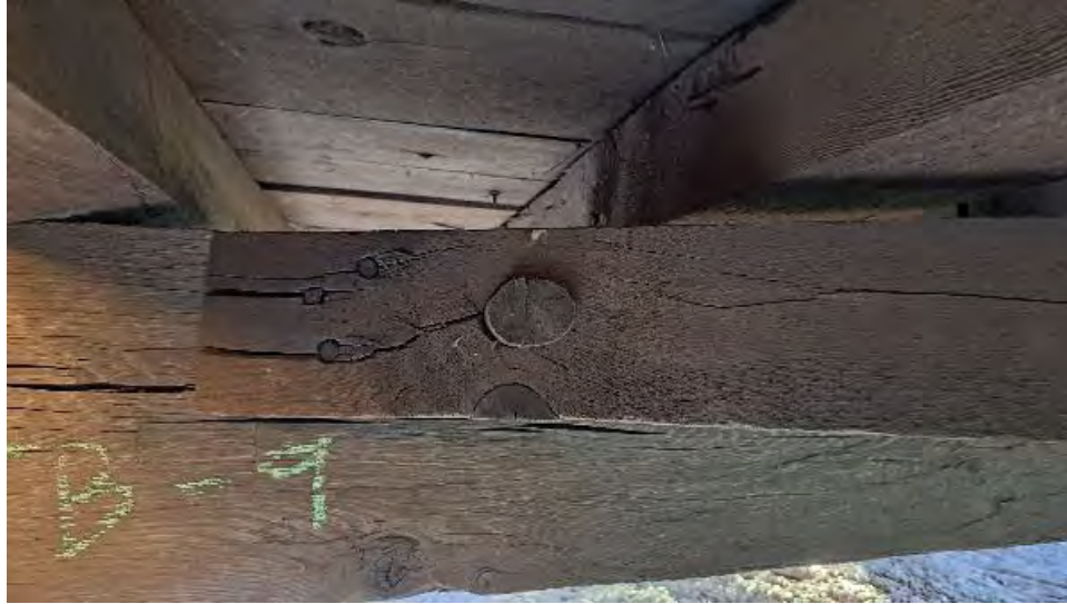
Figure 9-285: LCB-13 has cleaved on the dowel and spikes to TB9.
