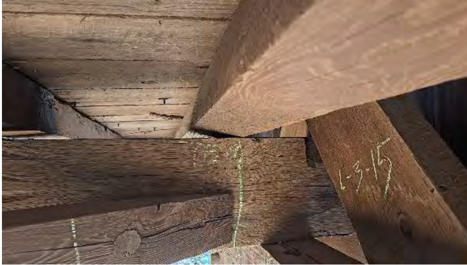
Figure 9-231: J9-8 twisted 12 degrees at TB9 end.
