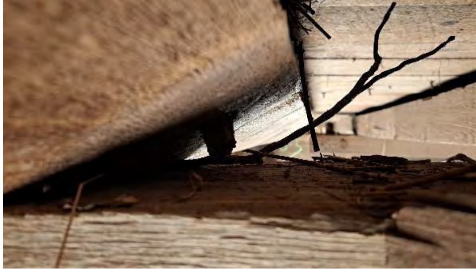
Figure 9-130: J3-8 is penetrated by a vertical broken dowel over TB4.
