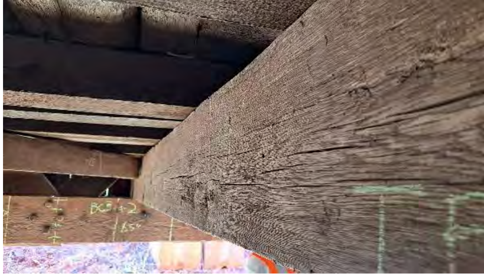
Figure 9-37: All visible sides of TB4 have planer skips or chisel scars.
