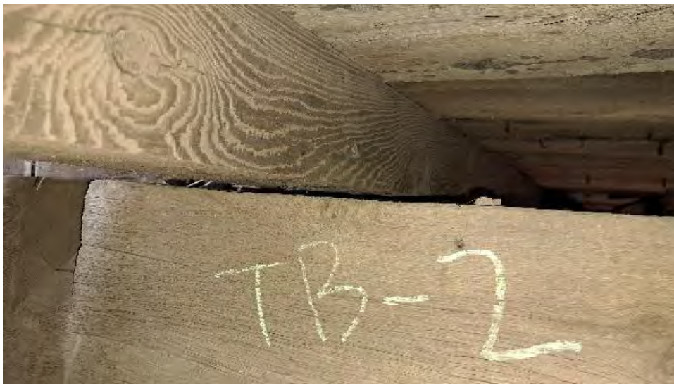
Figure 9-89: J1-8 is continuous with J2-8 but is not bearing on TB2.
