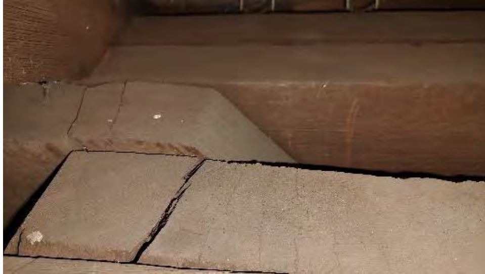
Figure 8-49: L1-4 top split on outer edge, nail is going through member on top.
