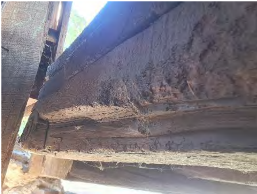
Figure 9-263: termite damage to bottom and South faces for most of the length with some minor cracking and damage.
