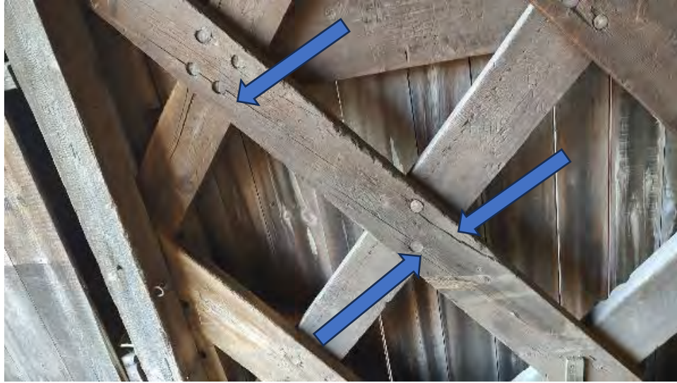
Figure 8-69: L3-2 has several cracks propagating from the dowelled connections to L4-2 & L4-3.
