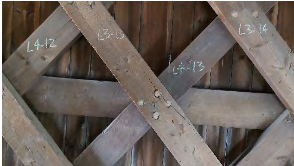
Figure 8-80: L3-13 is cracked through 1 row of dowels at the middle chord and L4-13.
