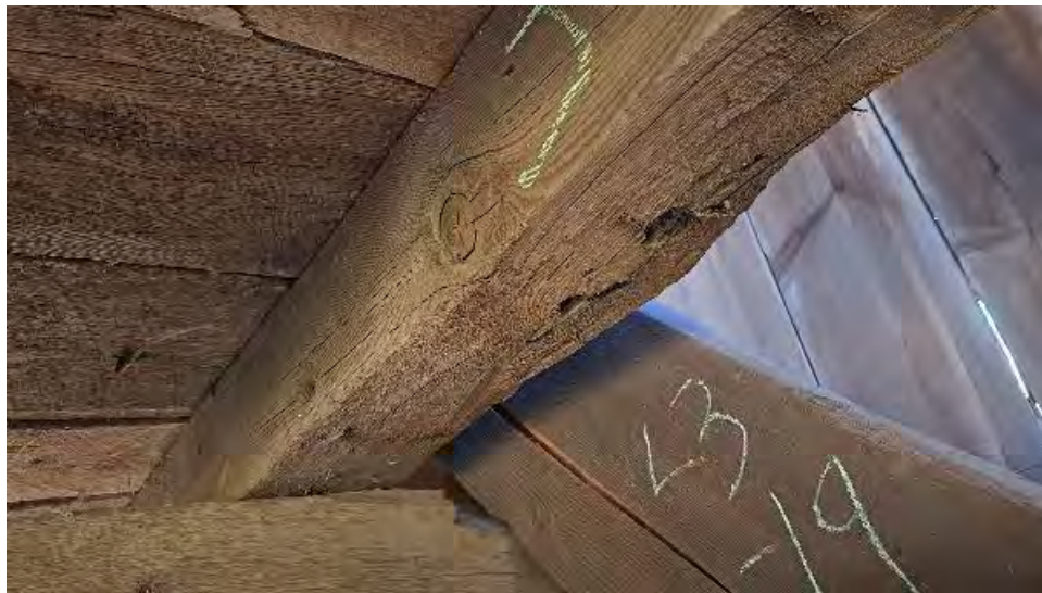
Figure 9-261: Joist J11-8 termite damage to bottom and South faces for most of the length with some minor cracking and damage.
