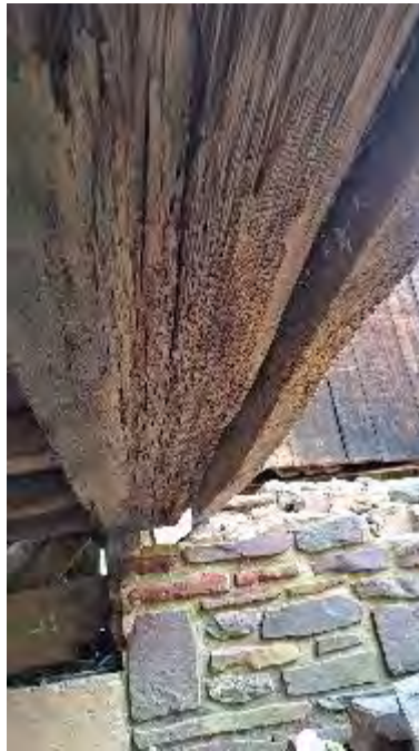
Figure 9-67: JT2 is severely decayed and with section loss on bottom face. A 3-inch-deep cavity exists on the bottom face. JT2 is not currently supported at either end.
