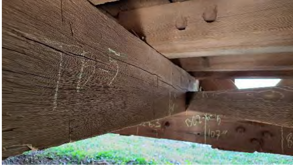
Figure 9-42: TB5 has planer skips and chisel scars on all visible sides. The North end is twisted 4 degrees and is lifting on the AB1 side from BC2.
