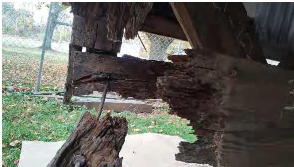
Figure 8-29: Significant decay and section loss to the AB2 ends of BC1 and BC2.
