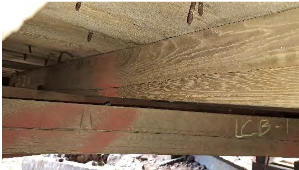
Figure 9-95: J2-3-N has a large split on the North side which extends from the lower corner at TB2 to approximately 12-inches from TB3 at 1/3 from the top edge.
