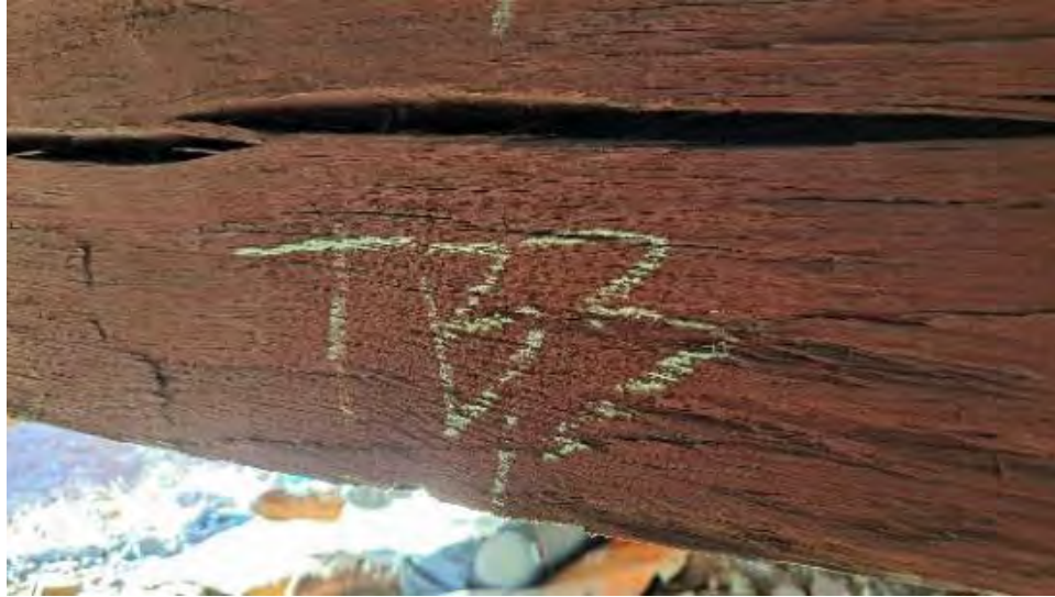
Figure 9-32: TB3 has large shrinkage checks on AB1 side that are up to 5/8-inches wide, for its full length.
