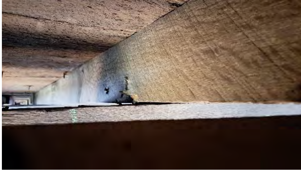
Figure 9-198: J8-3S has decay and section loss at its bearing over TB8.
