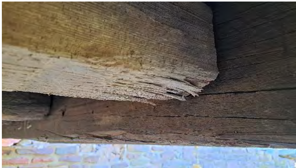
Figure 9-251: J11-3 has feathering at the bottom face at AB2 end.
