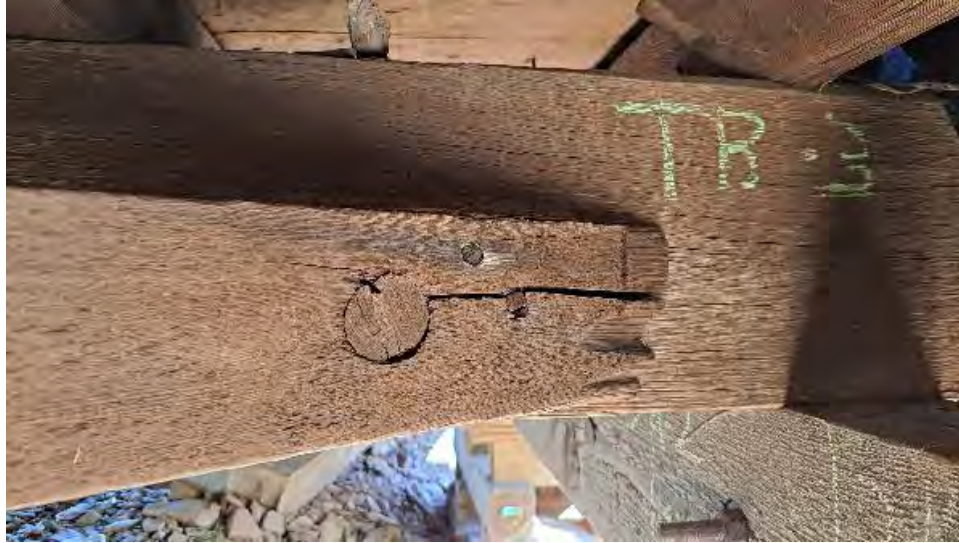
Figure 9-271: The LCB-4 dowel and spikes to TB3 have cleaved.
