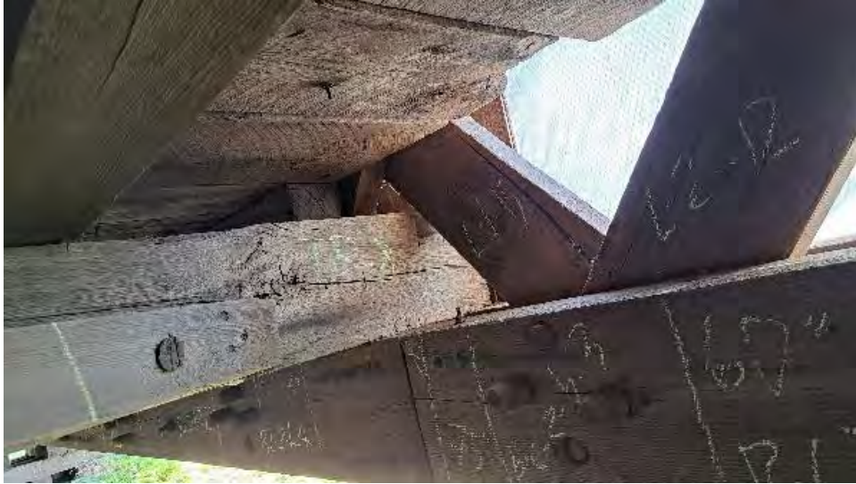
Figure 9-178: J7-1 is missing.
