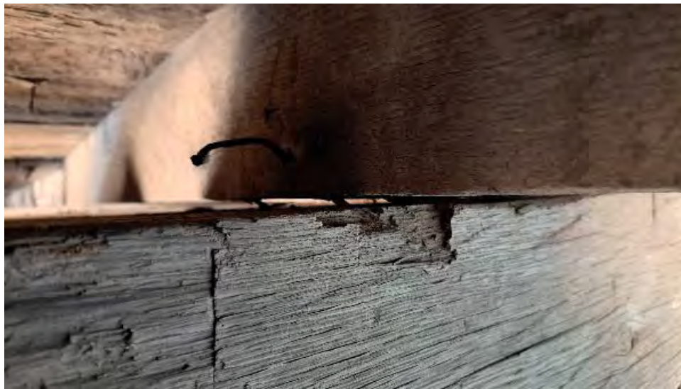
Figure 9-158: J5-5 is not bearing over TB6.
