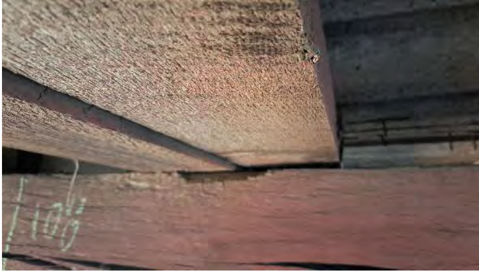
Figure 9-100: J2-5-N is not bearing over TB1.
