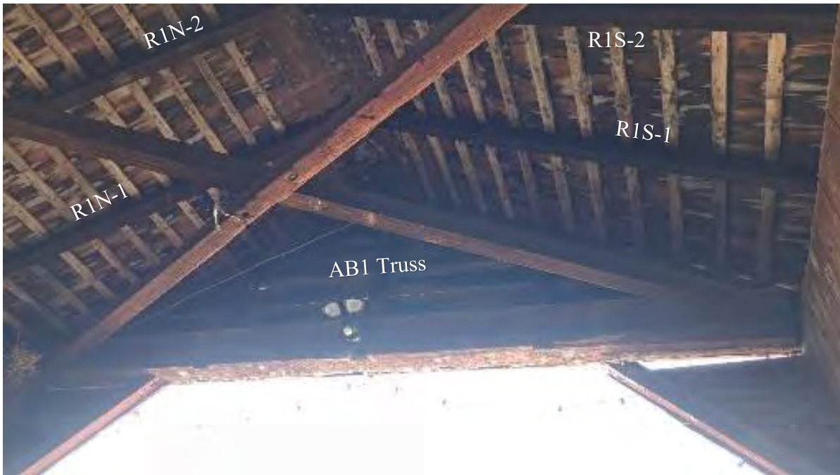
Figure 7-15: No access to Abutment 1 truss main rafters with limited visual accessibility. R1N & R1S appear to be in fair condition.
