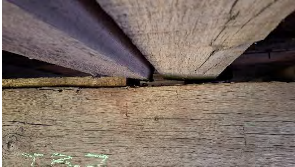
Figure 9-188: J7-5-N partial bearing on packer at TB7 & TB8. J7-5-S is not supported at TB7 or TB8. Old termite damage exists with pockets that have led to cracking at mid span.
