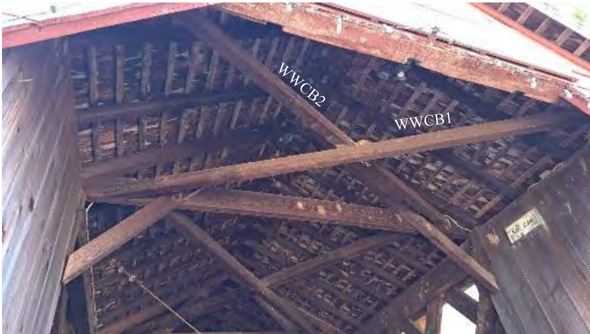
Figure 7-7: Wing wall upper cross braces WWCB1 and WWCB2 are in fair condition.
