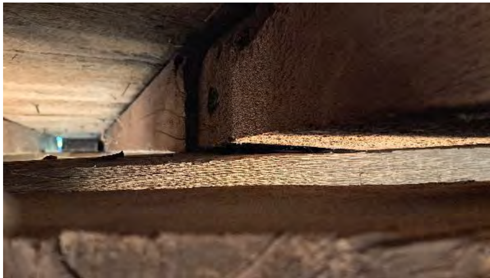
Figure 9-230: J9-7 is bearing on its North edge onto TB10 due to twisting of 6 degrees.
