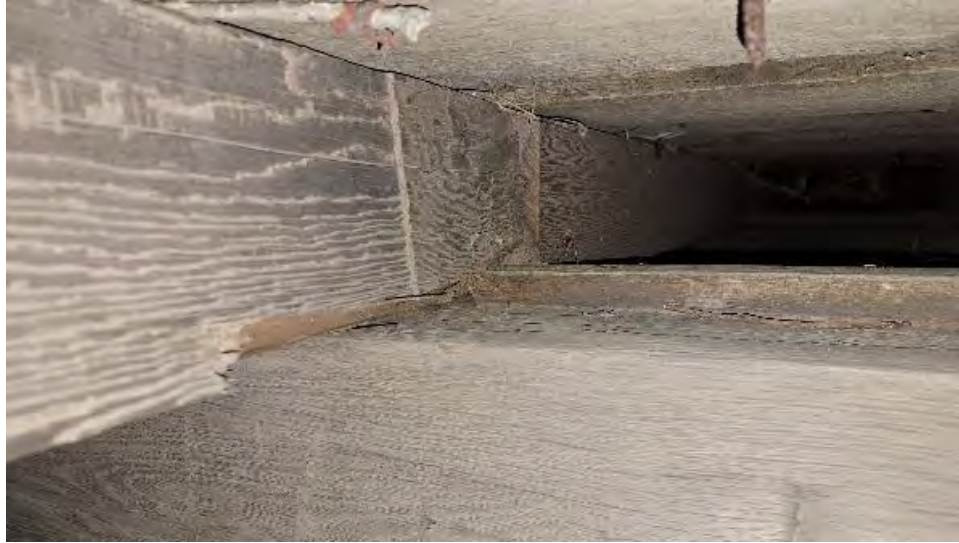
Figure 9-206: J8-5-N was partially packed over TB9 but now with section loss and only partially bearing on TB9.
