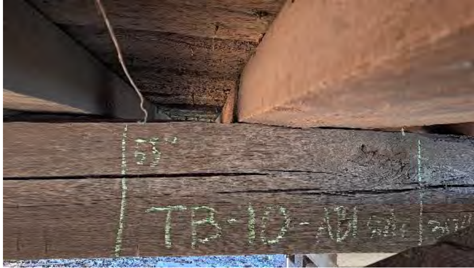
Figure 9-223: J9-3-S has minor twisting over TB10 due to sloped bearing surface of TB10.
