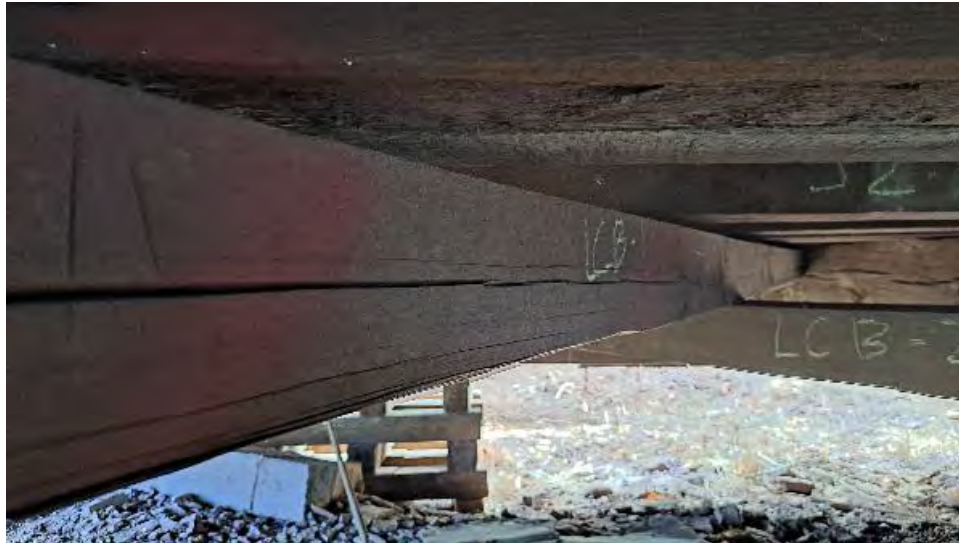
Figure 9-267: LCB-1 has end split extending to mid span.
