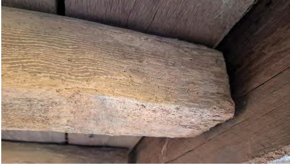
Figure 9-258: J11-6 has abrasion wear at the AB2 end.
