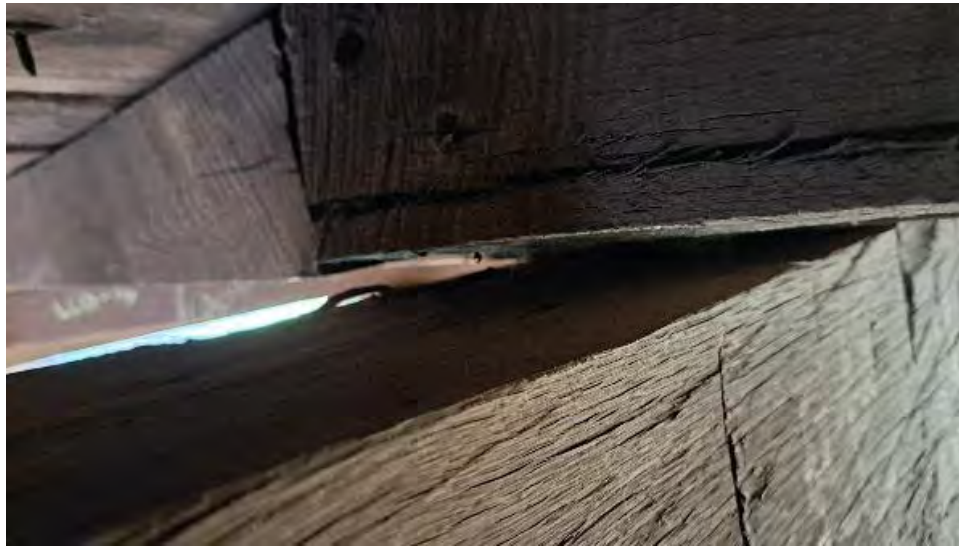
Figure 9-211: J8-7 has section loss on the top North end corner.
