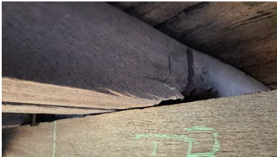
Figure 9-199: J8-3S has decay and section loss at its bearing over TB8.
