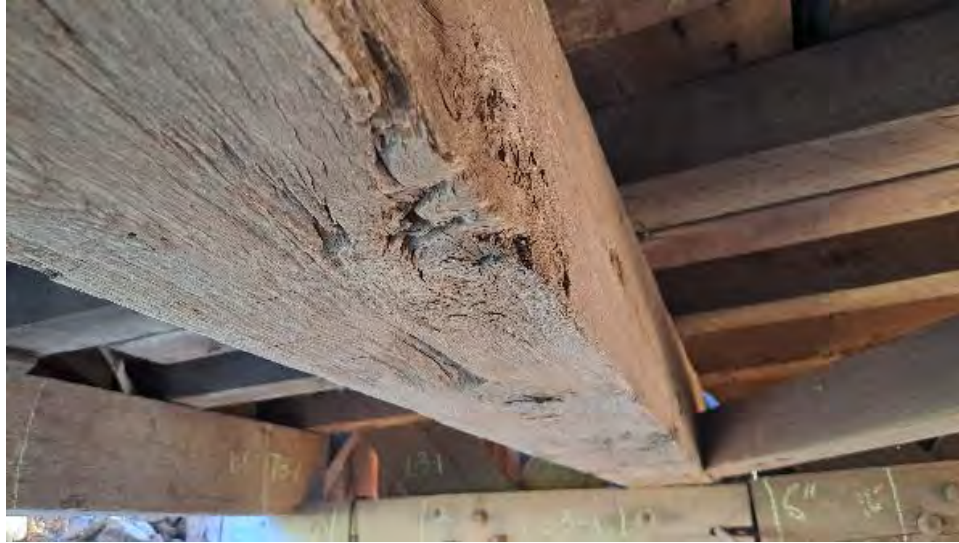
Figure 9-31: TB2 has another large knot on the bottom AB2 edge near the northern end.
