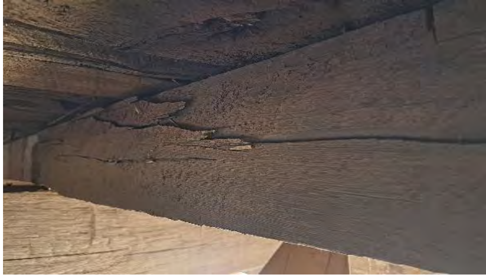
Figure 9-124: J3-6-N has a large end split at TB3 end. The North half is broken.
