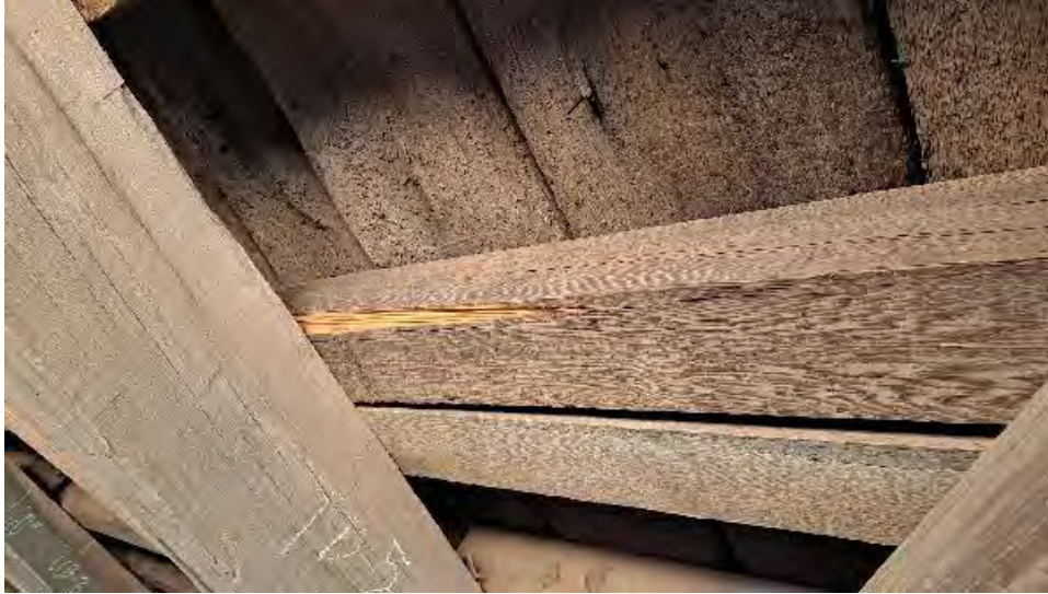
Figure 9-140: J4-4-S has section loss on the bottom edge and does not bear onto TB5.
