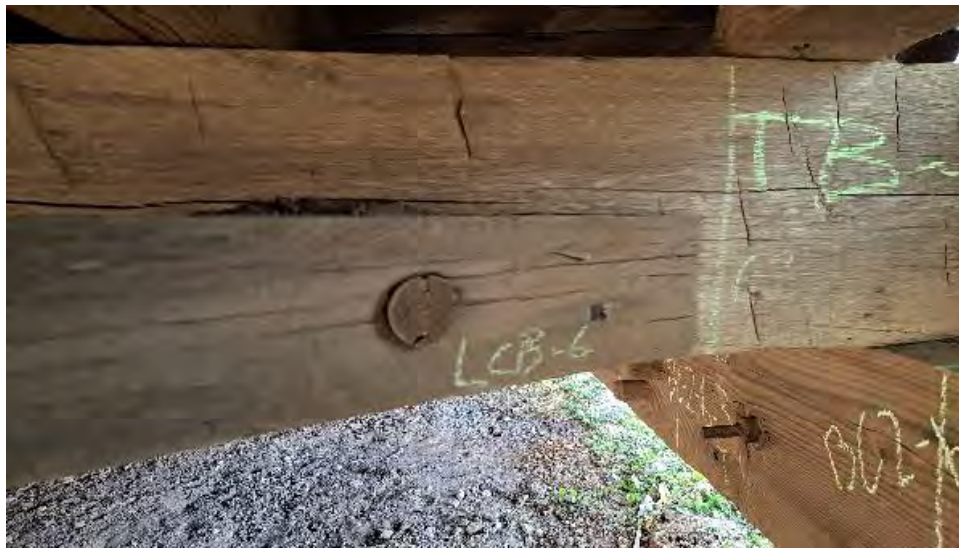
Figure 9-276: LCB-6 has some minor end splits through the dowelled connection to TB4.
