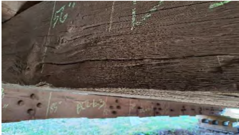
Figure 9-39: TB5 has a slope of grain crack on the AB2 side at 1/3 span from the North end with some section loss in bottom face.
