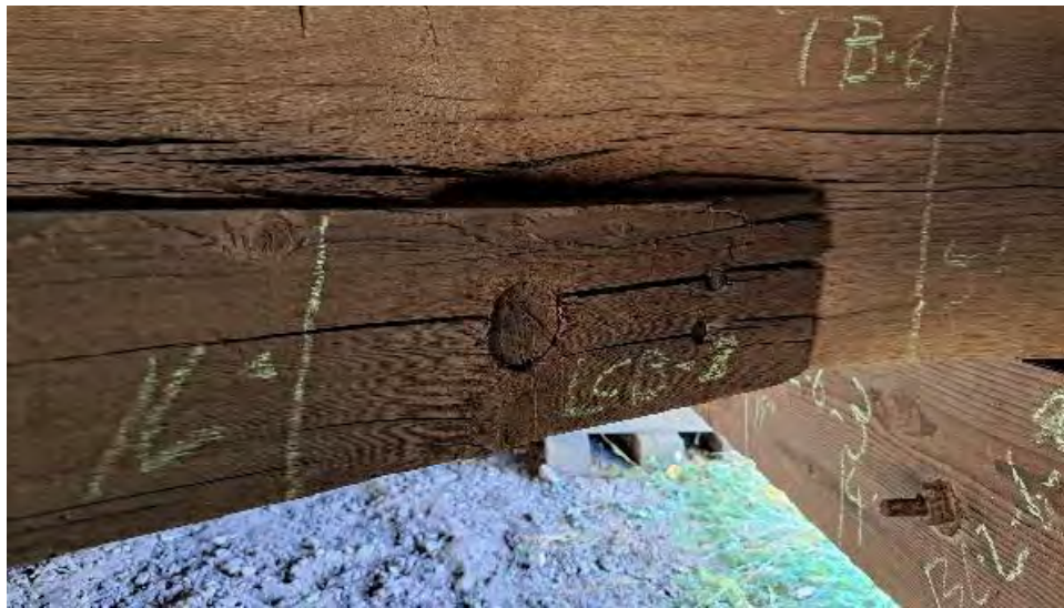
Figure 9-278: LCB-8 has cleaved on the dowel to TB6.
