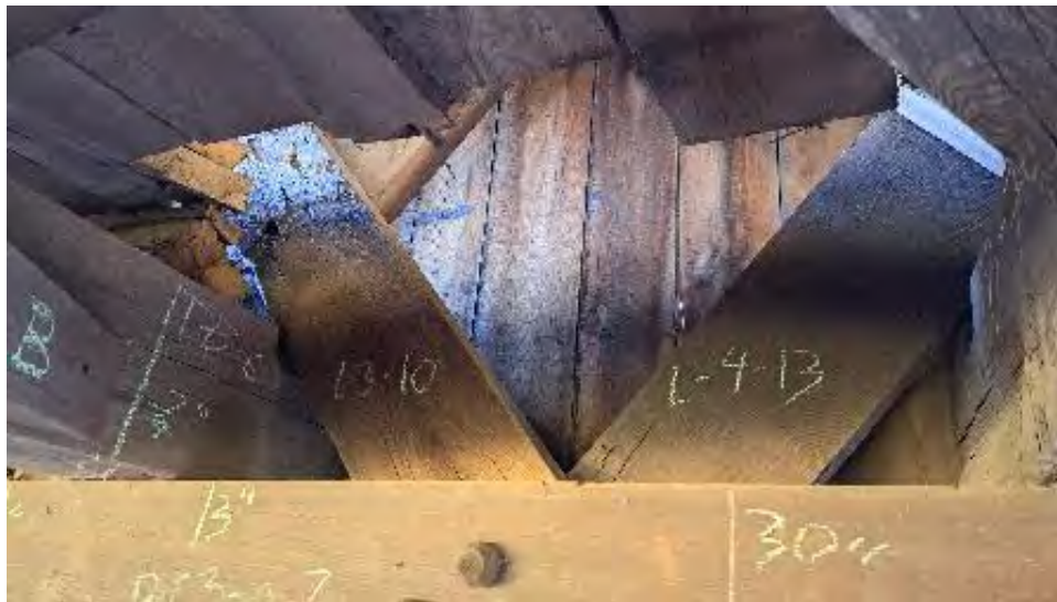
Figure 9-177: J6-8 is missing.
