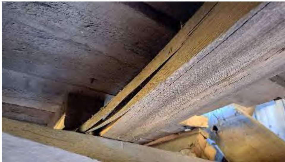
Figure 9-175: J6-7 has up to 1/2 cross section loss over TB6 and with several end splits at TB7.
