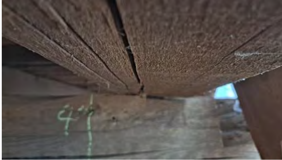
Figure 9-217: J9-1 has a vertical end split from TB10 (24-inches long) and is twisted 4 degrees at the TB10 end, possibly due to the end split and uneven bearing surface. Bearing on the North edge at TB9 only.
