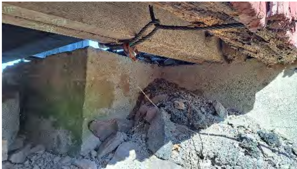
Figure 10-12: The receded backfill and segments of the asphalt surface are scattered against the mass concrete foundation of AB1.
