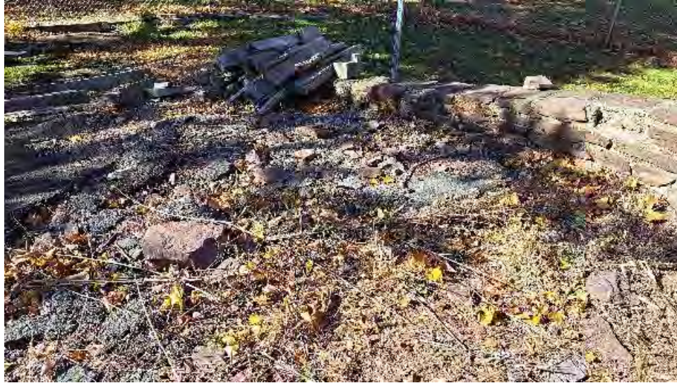
Figure 10-15: The backfilling at AB2 has receded and the asphalt surface is damaged for the full width of AB2. Significant debris exists over the approach. Loose timber elements are stockpiled at AB2.
