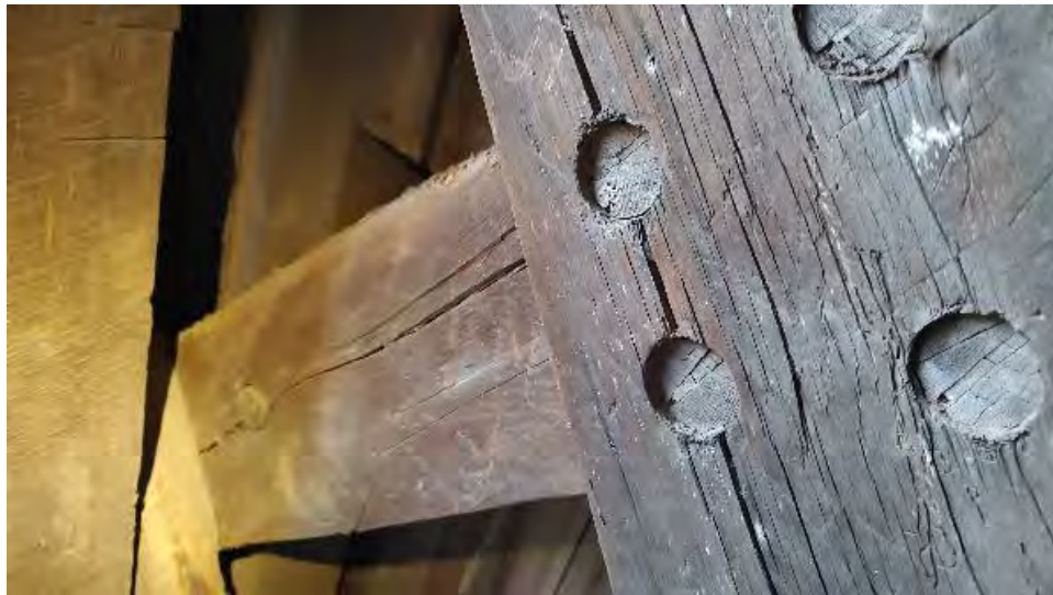
Figure 8-92: L4-2 is cracked either side of the connection to L3-2 and with shrinkage checks through 1 row of dowels.
