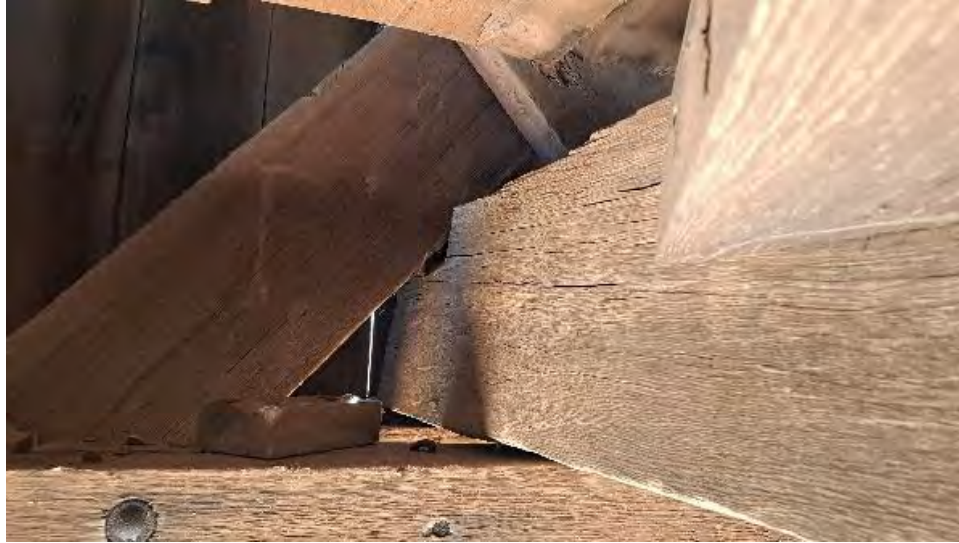
Figure 9-53: TB8 is twisted at the North end by 2-inches and has lifted off BC2 on the AB2 side.
