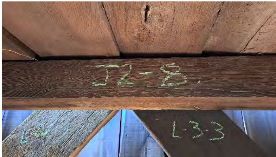
Figure 9-107: J2-8 has vertical cracks to the bottom face, extending to the North side.
