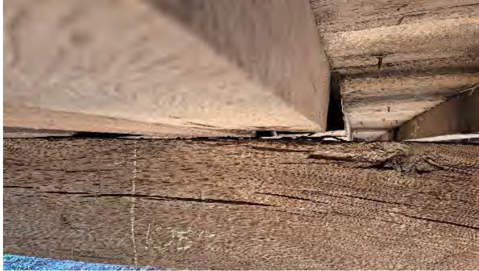
Figure 9-227: J9-6-N and J9-6-S are not bearing onto TB9.
