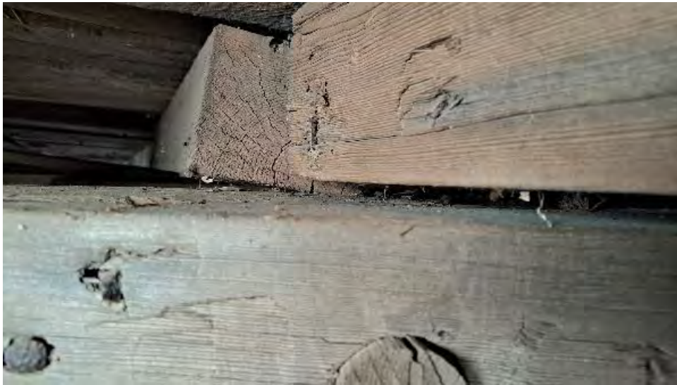
Figure 9-179: J7-2 is not bearing on TB7.
