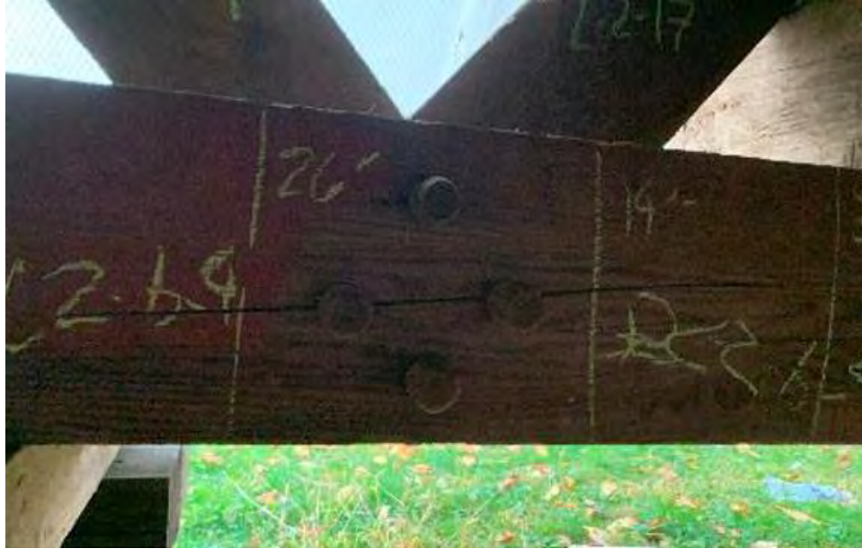
Figure 8-43: Shrinkage checks exist through BC2B splices.
