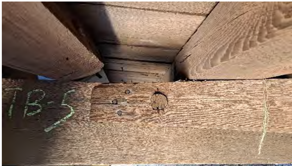
Figure 9-274: LCB-5 has cleaved on the dowel to TB5.
