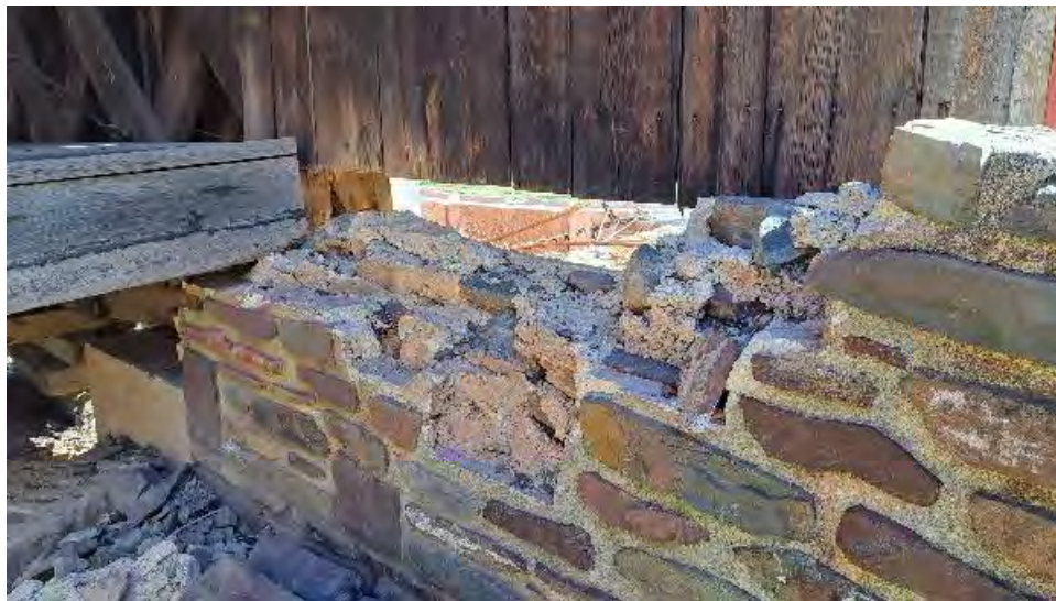
Figure 10-22: The North side of AB2 has approximate 10-foot length of stone wall destroyed for approximately half of its height.
