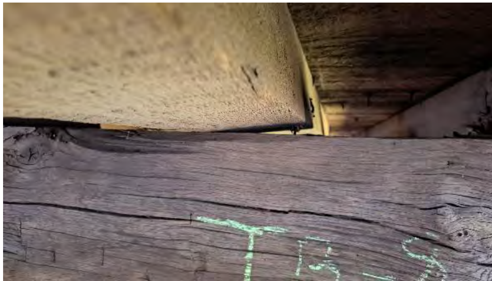
Figure 9-185: J7-4 is only bearing on the South edge at TB8
