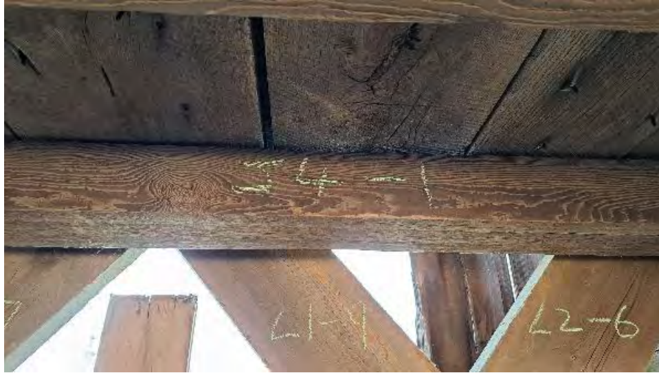
Figure 9-132: J4-1 has a bottom face split extending from TB4.
