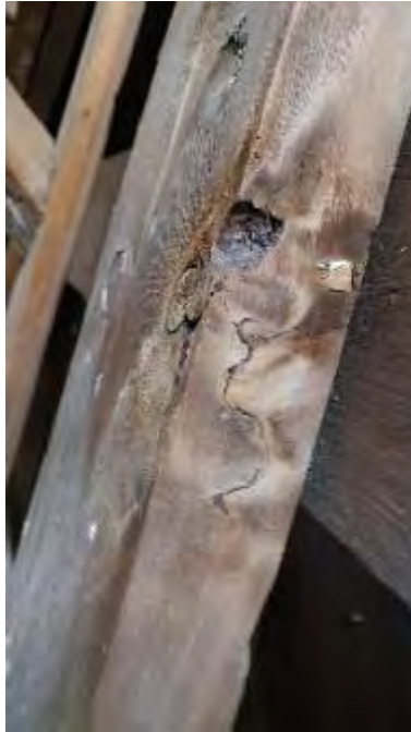
Figure 8-63: L2-9 is cracked at the dowel connection to L1-8.
