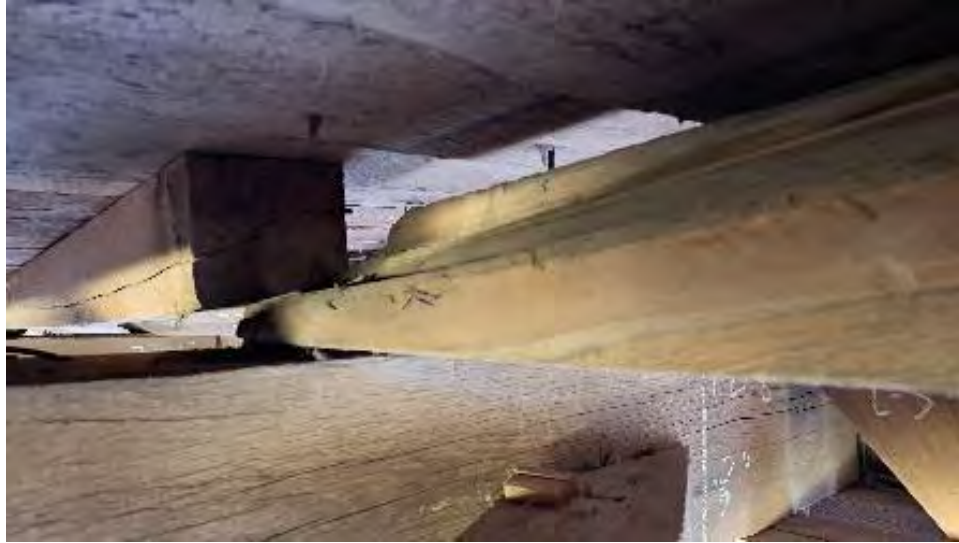
Figure 9-174: J6-7 has up to 1/2 cross section loss over TB6 and with several end splits at TB7.
