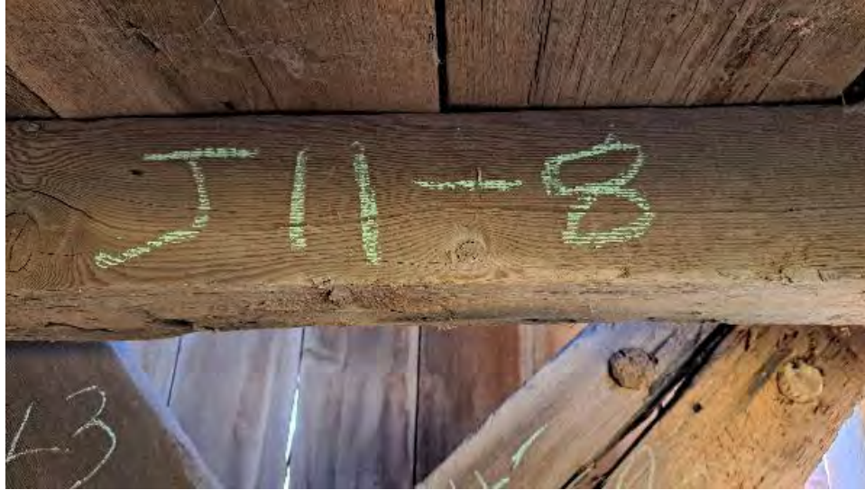
Figure 9-260: J11-8 termite damage to bottom and South faces for most of the length with some minor cracking and damage.
