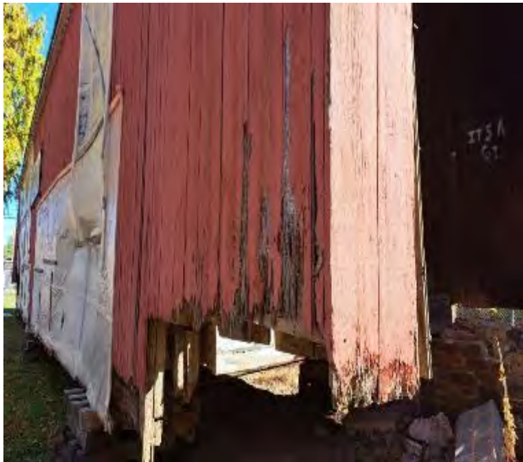
Figure 6-13: Siding on Northwest side end wing wall at Abutment 2 showing section loss and decay on bottom of boards.
