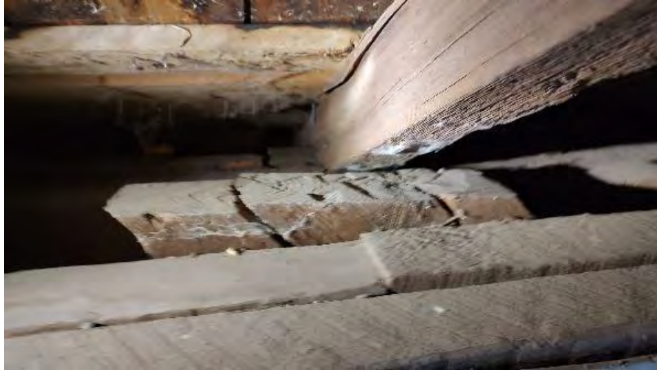
Figure 8-85: L3-18 has end splits originating at both rows of dowels at the top chord.
