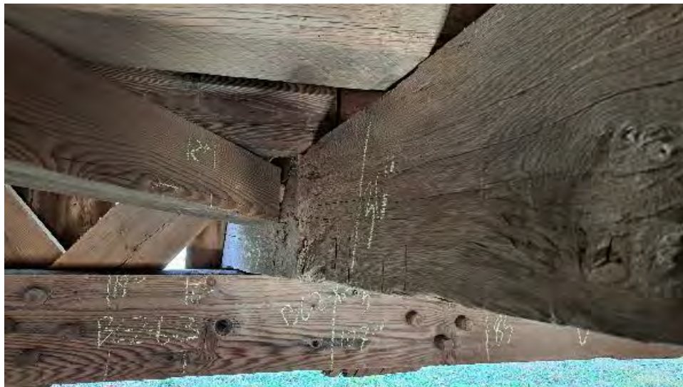
Figure 9-41: TB5 has planer skips and chisel scars on all visible sides. The North end is twisted 4 degrees and is lifting on the AB1 side from BC2.
