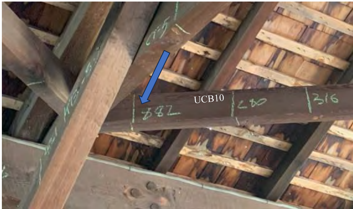
Figure 7-13: Upper cross brace UCB10 has a split 6-inches from CT-5 on the South side.
