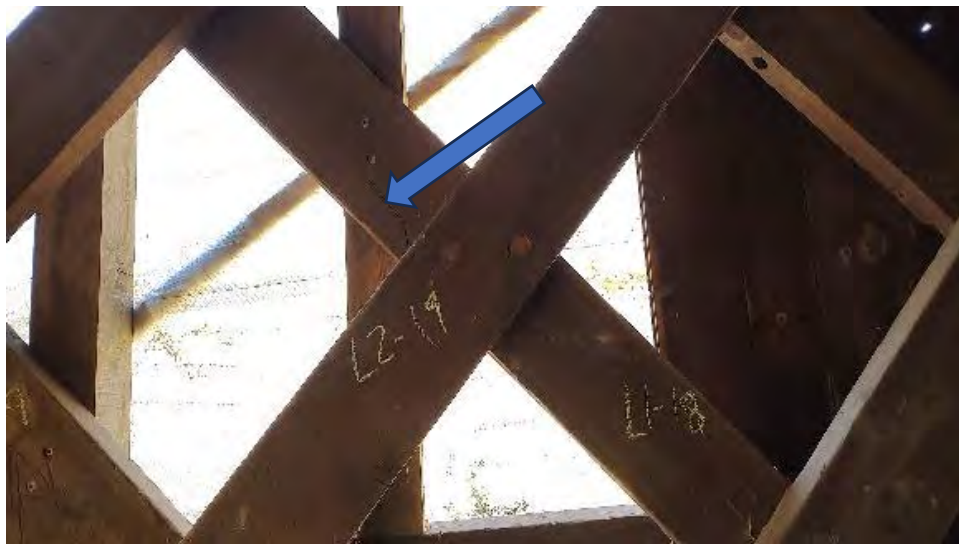
Figure 8-54: L1-18 is cracked on its side and lower edge above the intersection with L2-19.
