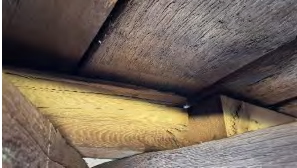
Figure 9-176: J6-7 has up to 1/2 cross section loss over TB6 and with several end splits at TB7.
