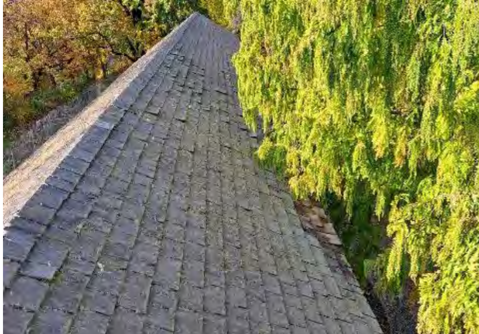
Figure 6-3: North side roof top of the Bridge with areas of cupping under the area shaded by the redwood tree. This area is likely to hold more water, but the upper layer of shakes is exposed and able to dry, resulting in cupping of the upper layer.
