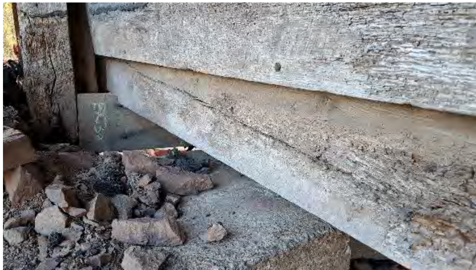
Figure 9-25: TB1 has a large shrinkage check originating from the South end, on Abutment 1 side which extends for 5 to 6 feet.
