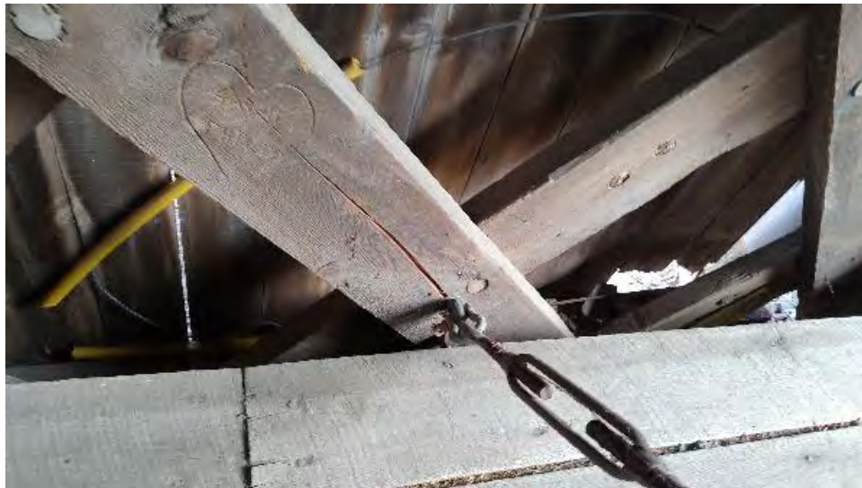
Figure 8-86: L3-19 is split by the temporary brace anchor, located approximately 6-feet from the bottom chord.
