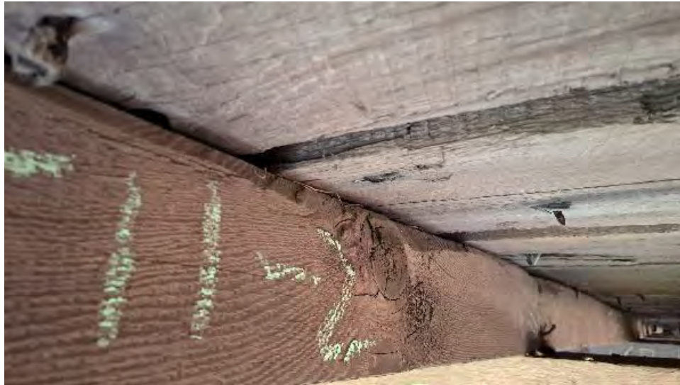
Figure 9-249: J11-2 has a large knot on the South face at mid span, likely extending to the top face with some section loss from slope of grain cracking and wane.
