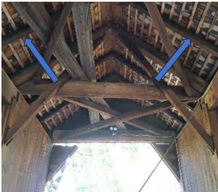
Figure 1-3: Roof rafters that were inaccessible for ladder use while doing the inspection.
