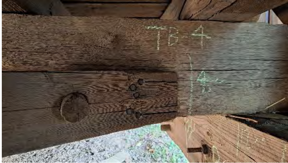
Figure 9-273: The doweled connection of LCB-4 to TB4 has been reinforced with 5 spikes, with cleaving on 3 spikes.
