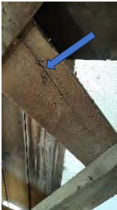
Figure 8-56: Shrinkage checks exist to L1-20 which extend from the dowelled connection with the top chord.
