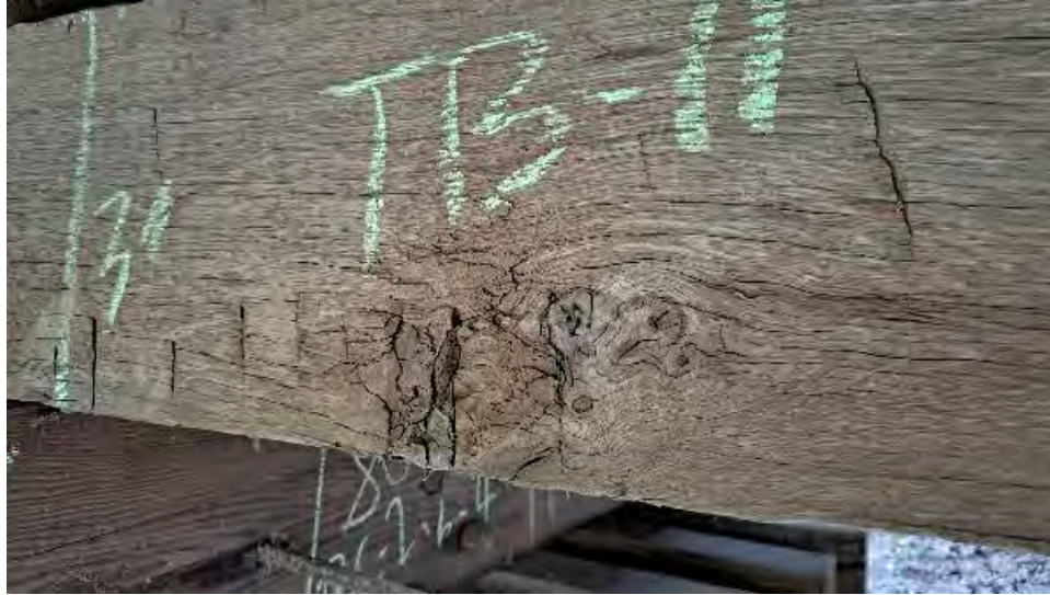
Figure 9-65: TB11 has a large knot on the bottom AB2 edge, approximately 12-inches from the North end.
