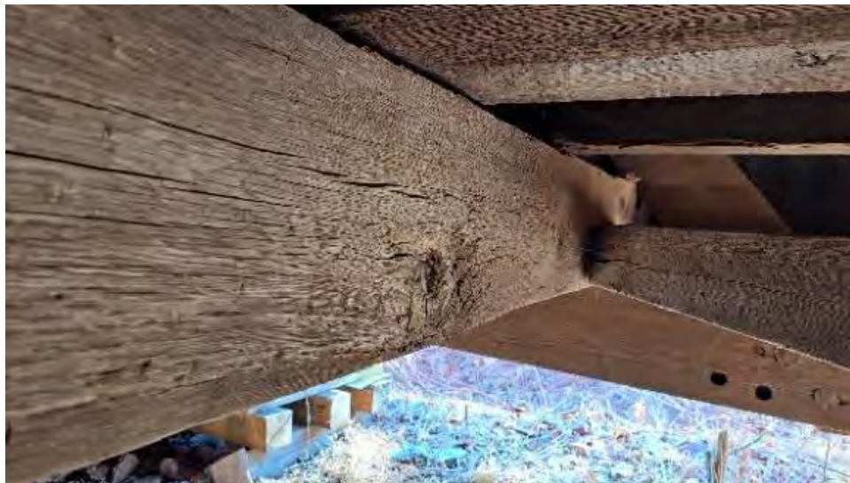
Figure 9-47: TB7 has a large knot on the AB1 side. Section loss exists above BC3A resulting from the old slope of grain cracks.
