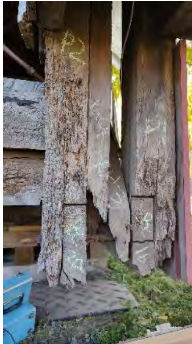
Figure 8-110: Post P1 is decayed and with termite damage for bottom 2-feet. P2 is decayed and with insect damage and section loss for bottom 3-feet. The packer between P2 and the lattice member has decayed and section loss.
