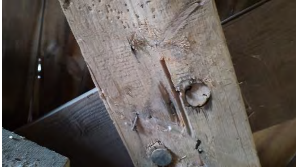
Figure 8-79: L3-11 is cupping on longitudinal alignment on the inside face where pith is evident (note the short pith segment that is missing).
