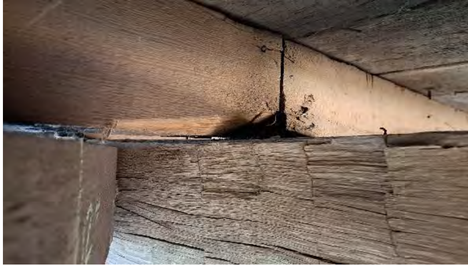
Figure 9-236: J10-2 has wane on South corner over TB10, reducing bearing width to 4.75-inches.
