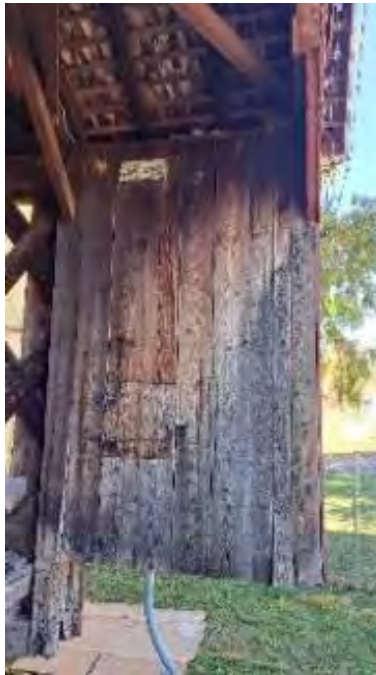
Figure 6-24: Abutment 1 North side wing wall view of internal siding.
