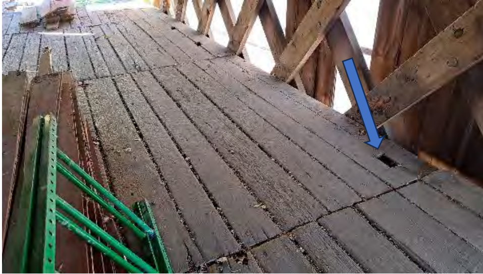
Figure 9-17: Floor decking Span 7, North side, with common hole in Planks 1 and 2.
