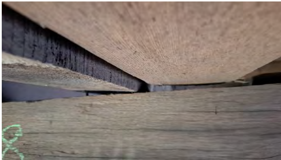
Figure 9-201: J8-4-S is not bearing over TB8.
