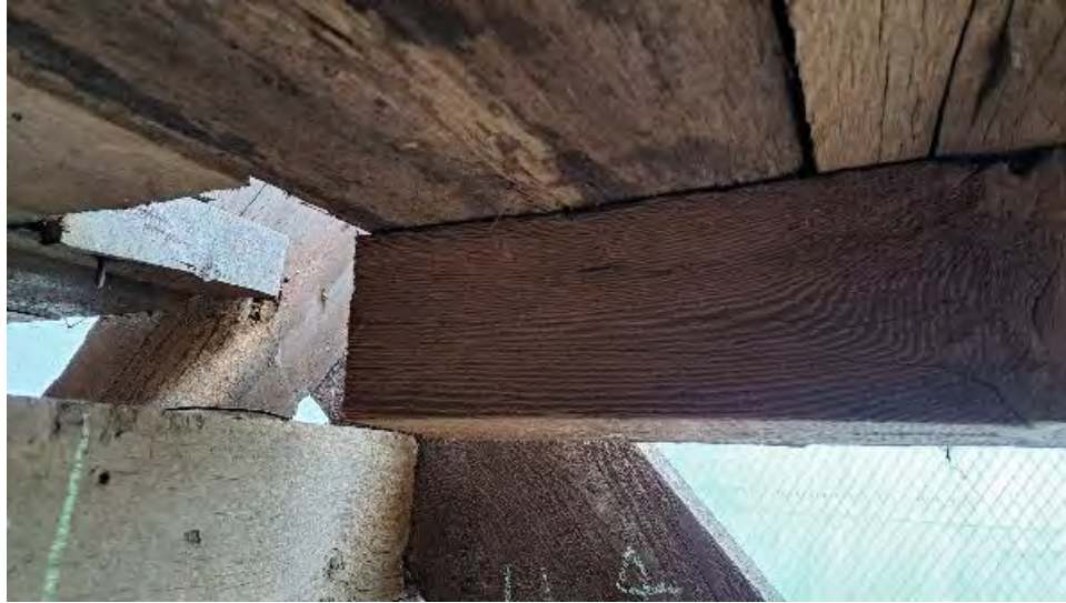
Figure 9-72: J1-1 has reduced bearing over TB2.
