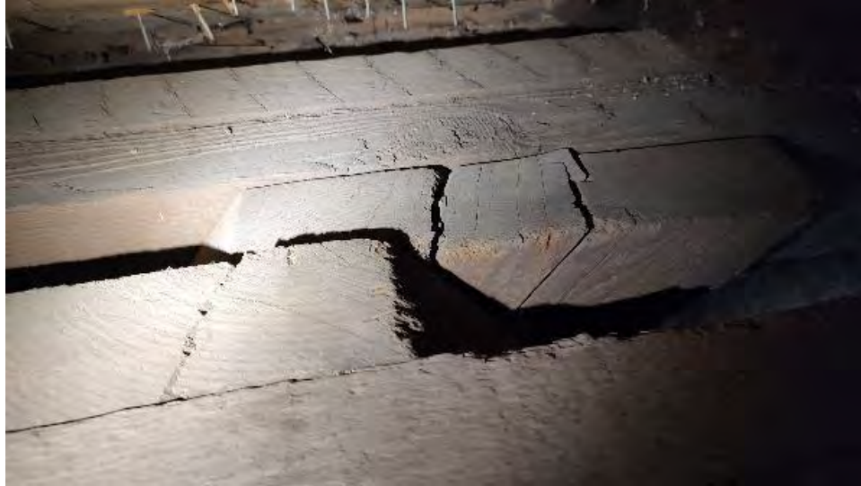
Figure 8-107: L4-20 has split extending from the dowels at the top chord.
