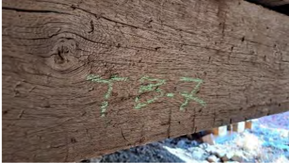
Figure 9-46: TB7 has planer skips and chisel scars on the AB1 side.
