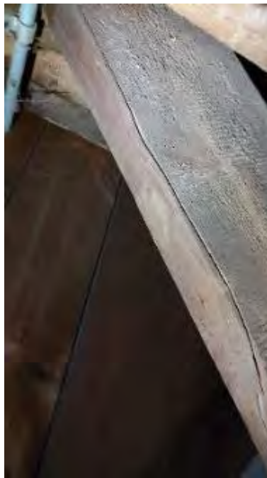
Figure 8-82: The bottom face of L4-11 is cracked.
