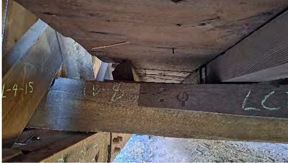
Figure 9-192: J7-8 is missing.
