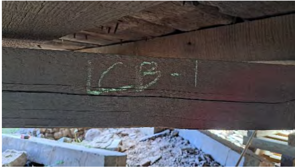
Figure 9-265: LCB-1 has some large shrinkage checks on the side face.
