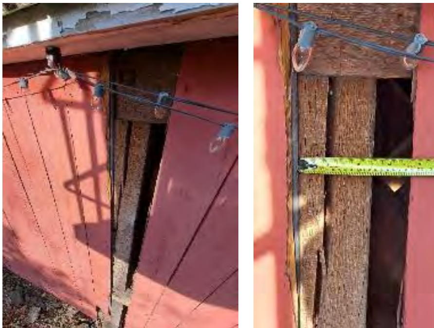
Figure 6-15: Missing boards at Post 8 at Abutment 2 on the South side.
