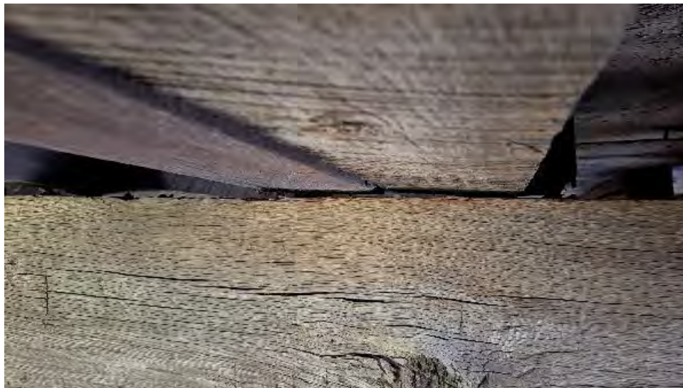
Figure 9-189: J7-6-S is not bearing over TB7.
