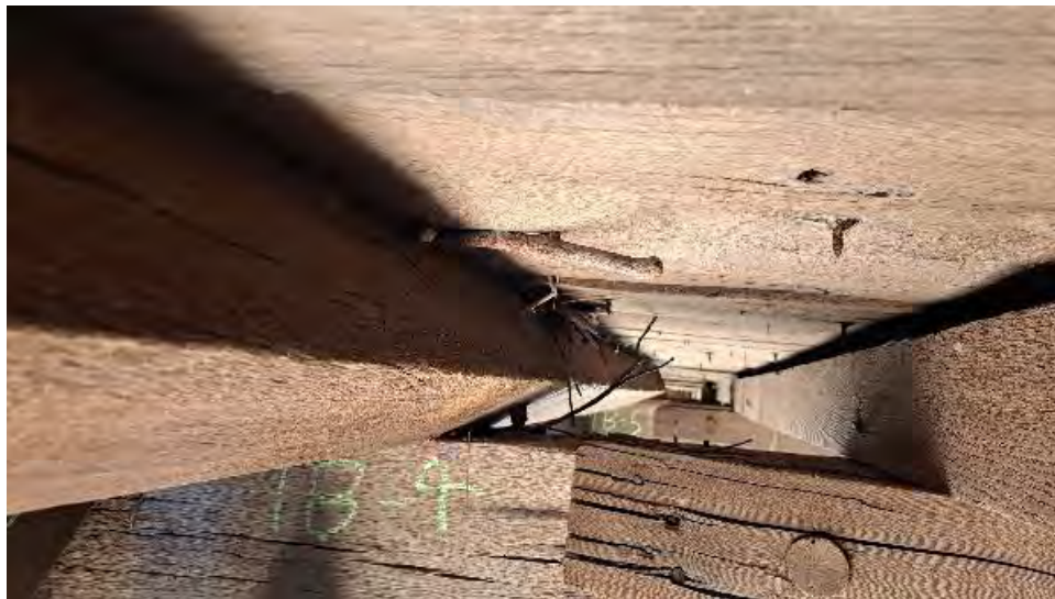
Figure 9-129: J3-8 is penetrated by a vertical broken dowel over TB4.
