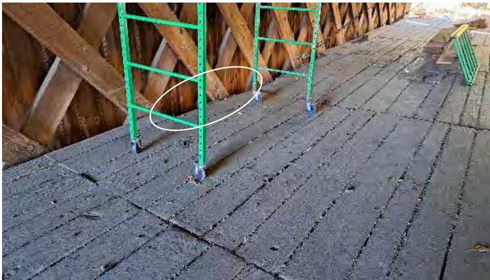
Figure 9-10: Floor decking Span 5, South side. Half of Plank is 18 missing.
