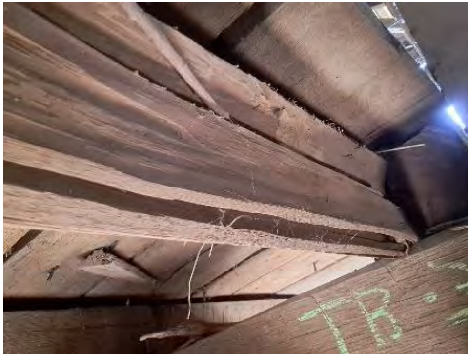
Figure 9-131: J3-8 has major cracking on the South side at TB3 for 2-foot length.
