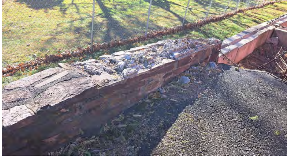
Figure 10-9: The top course of stone is missing from the South side of AB1 for the length of the wing wall.
