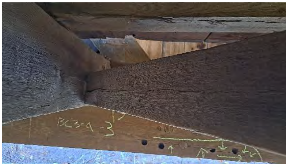
Figure 9-284: LCB-12 has an end split on its AB1 side face at TB7 end.
