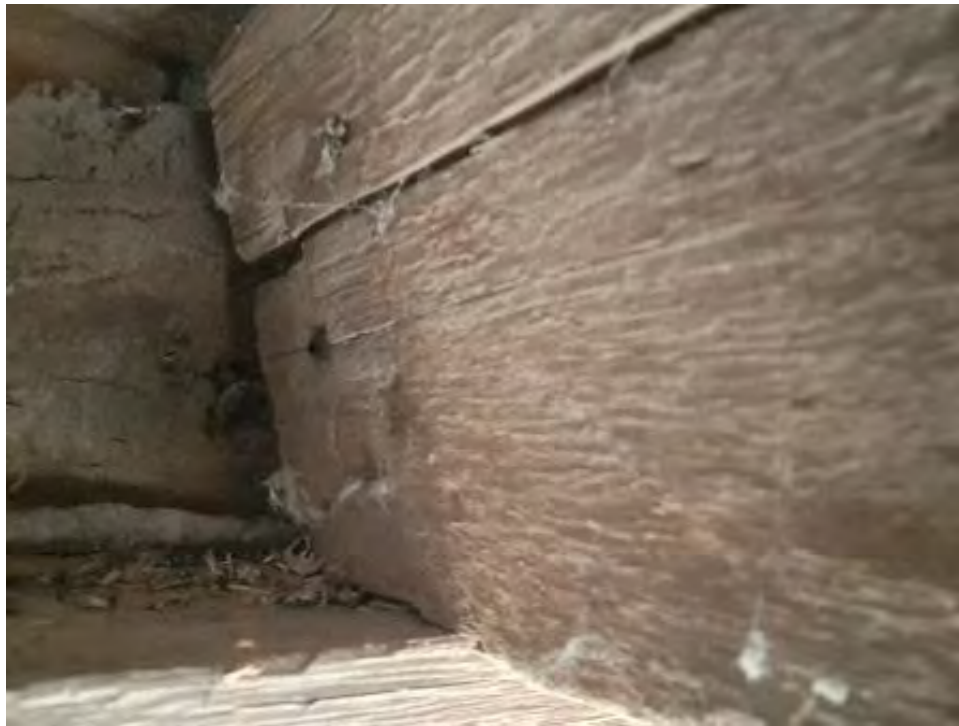
Figure 9-233: J9-8 has end splitting showing its South side only at TB10 end that is 4-feet long. J9-8 is likely cracked on its top surface. There is an end split 8-inches long on its North face from TB10.
