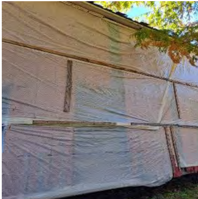
Figure 6-9: Siding on Northeast side showing missing boards in multiple locations behind the temporary plastic wrapping.
