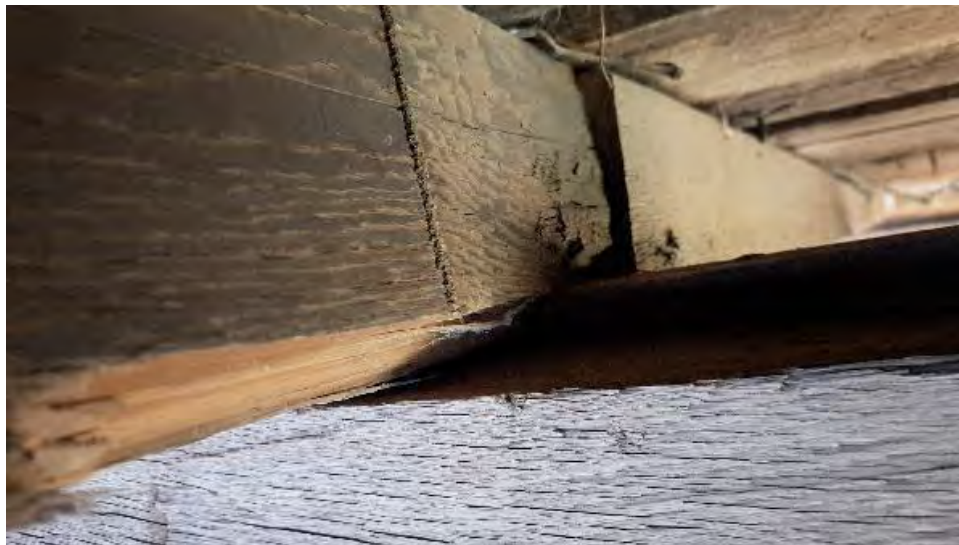
Figure 9-205: J8-5-N was partially packed over TB9 but now with section loss and only partially bearing on TB9.
