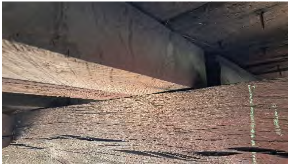
Figure 9-103: J2-6-N is bearing on TB3 on its South edge only. It is not twisted but is not a square section.
