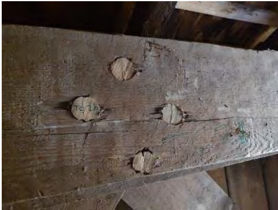
Figure 8-1: Shrinkage checks on dowels to TC2B connection with lattice.
