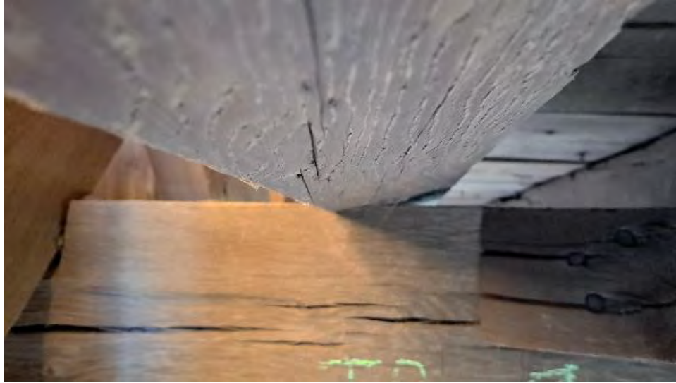
Figure 9-214: J8-8 has twisted about 15 degrees at TB9, resulting in crushing of the TB9 and J8-8 interface.
