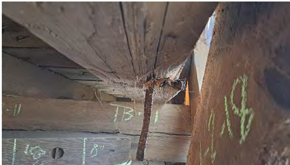
Figure 9-235: Wane exists on the North bottom edge of J10-1 for 3-feet from TB11 with approximately 1x1-inch section loss.
