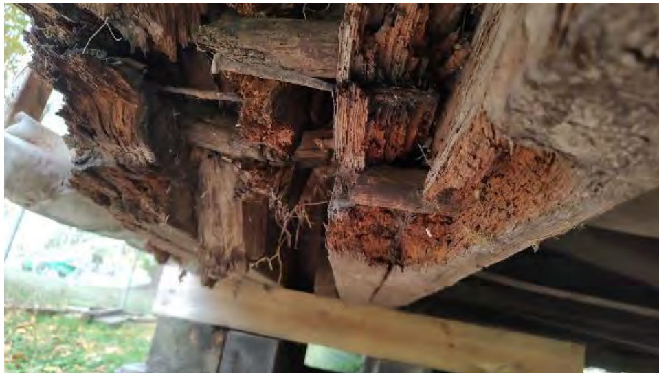
Figure 8-31: Significant decay and section loss to the AB2 ends of BC1 and BC2.
