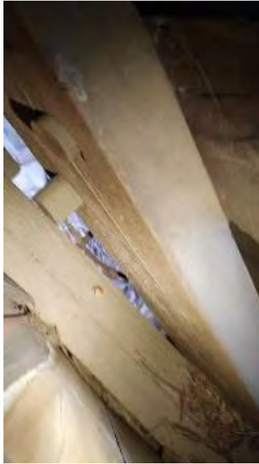
Figure 8-95: L4-5 is cracked through a dowel at the connection to L3-3.
