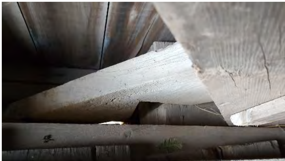
Figure 8-94: L4-4 has a notch 2/3 of its depth over a transverse beam.
