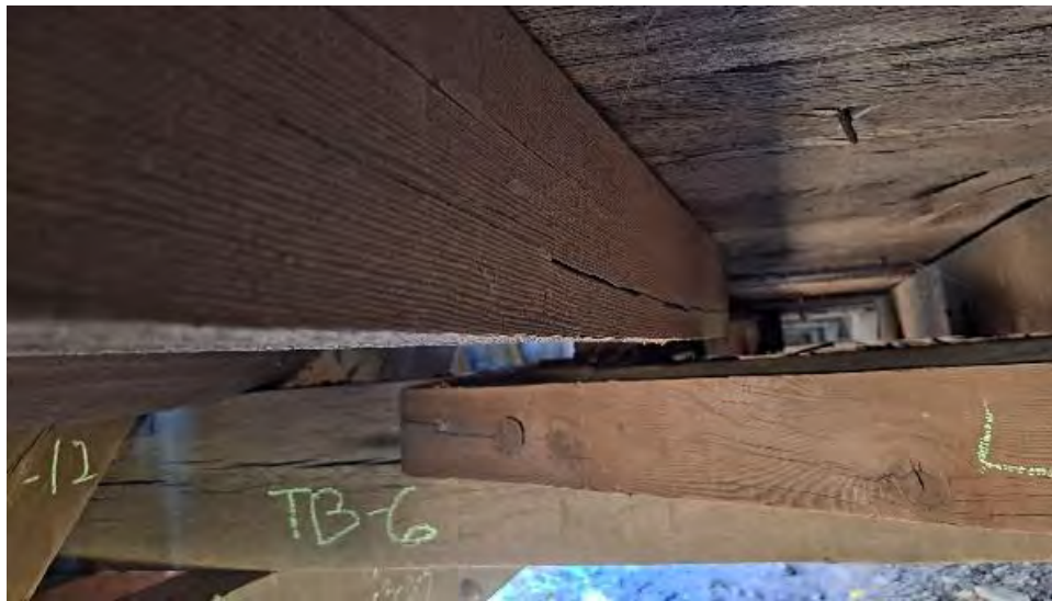
Figure 9-162: J5-7 is cracked for 3-feet length on the North side from TB6. J5-7 is not bearing on TB6.
