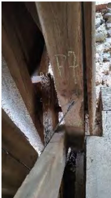
Figure 8-116: The bottom 16-inches of P7 are in very poor condition with decay.
