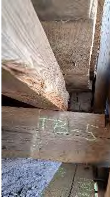
Figure 9-134: J4-1 has 1.25-inch bearing on TB5. Some impact damage and section loss exist above TB5.
