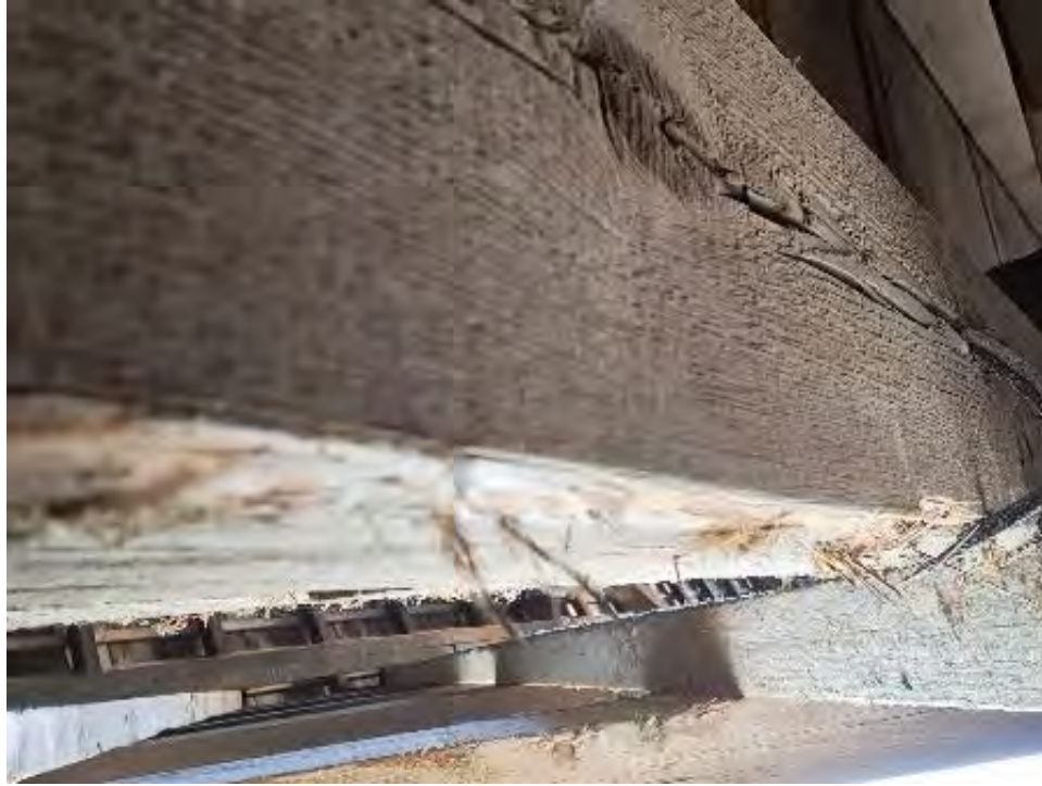
Figure 9-149: J5-1 has abrasion damage to its North edge.
