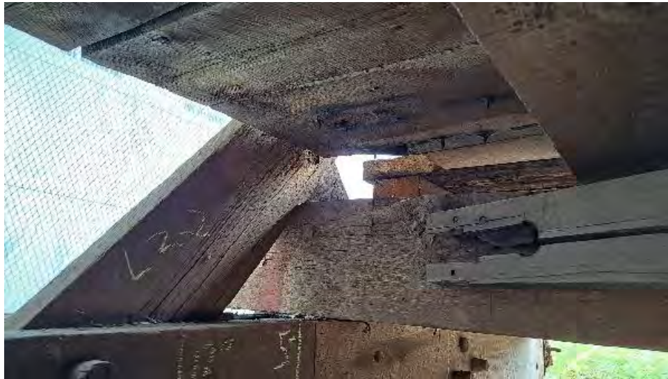
Figure 9-91: J2-1 is missing.
