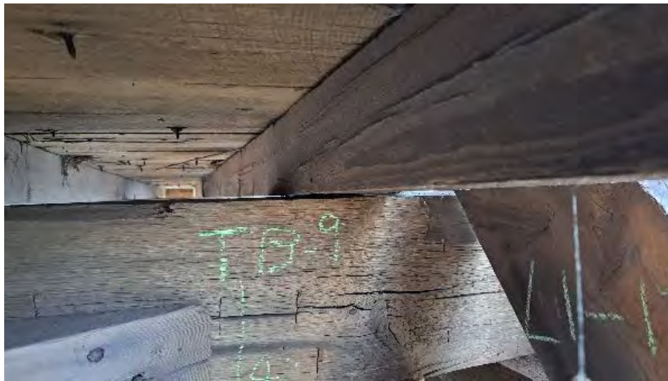
Figure 9-195: J8-1 is not bearing on TB9.
