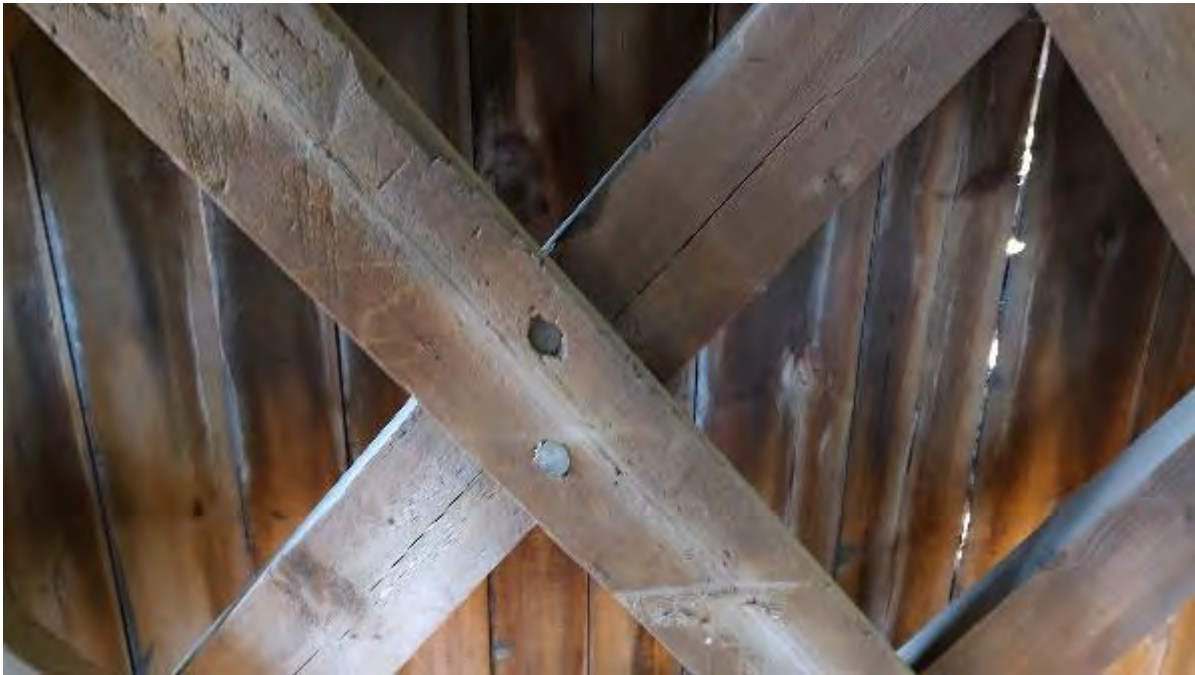
Figure 8-100: L4-12 is cracked through the bottom dowel at L3-11.
