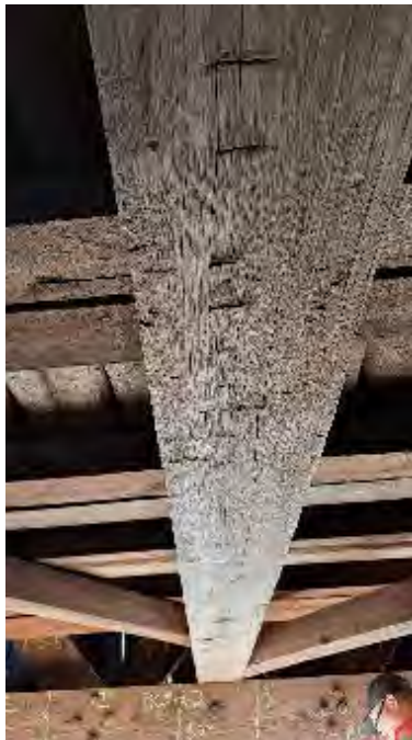
Figure 9-36: All visible sides of TB4 have planer skips or chisel scars.
