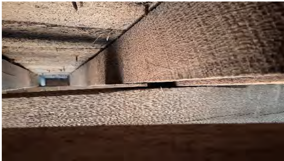
Figure 9-228: J9-6-S is not bearing onto TB9.
