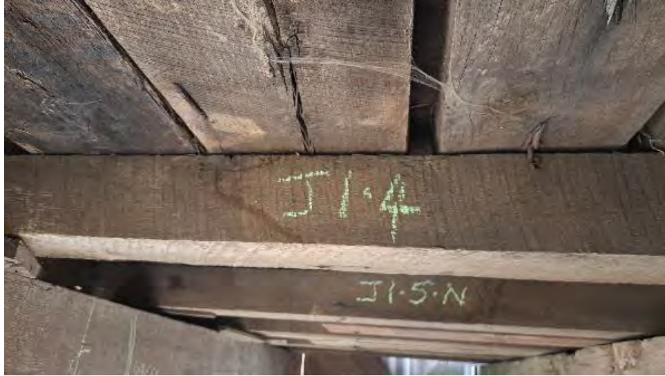
Figure 9-76: J1-4 is in fair condition.
