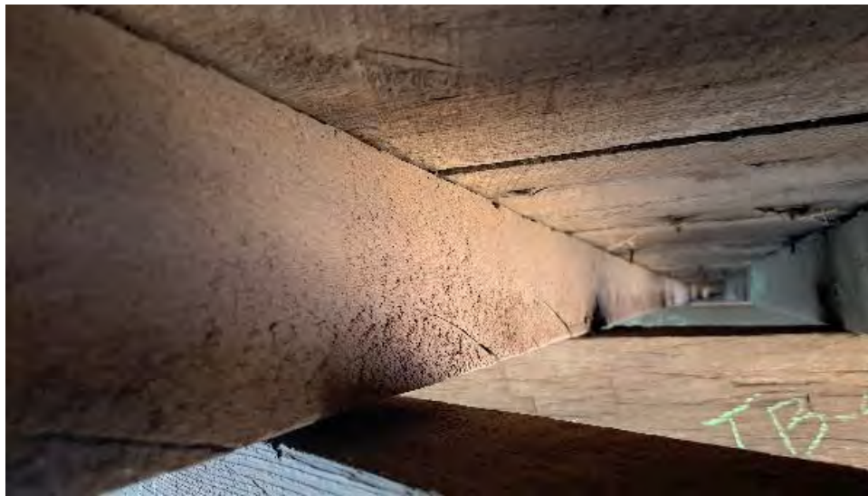
Figure 9-222: J9-3-S is cracked from the bearing over TB9 to 1/3 span.
