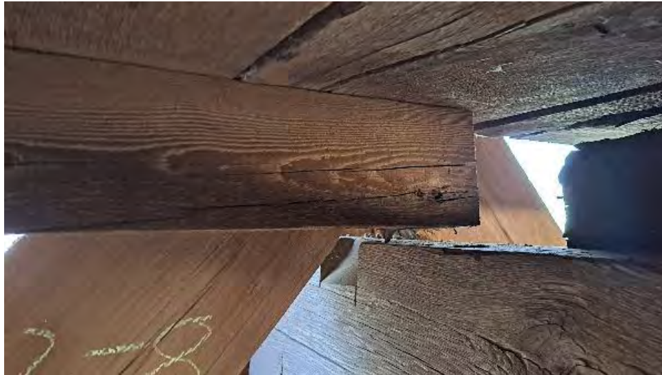
Figure 9-147: J5-1 is not bearing on TB4.
