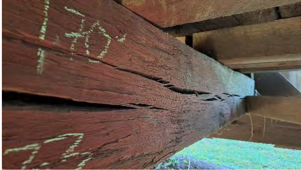
Figure 9-34: TB3 has large shrinkage checks on AB1 side that are up to 5/8-inches wide, for its full length.
