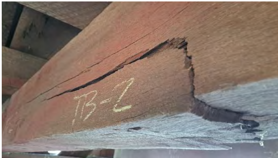
Figure 9-30: TB2 is broken, extending from the bottom face at mid span and caused by extreme slope of grain around a large knot on the side face.
