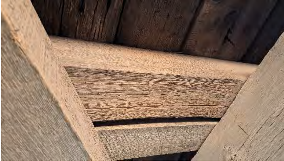
Figure 9-138: J4-3-N has section loss of pith from bottom face at mid span.
