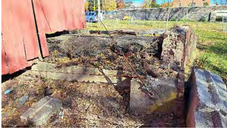
Figure 10-11: The backfilling at AB1 has receded and the asphalt surface is damaged for the full width of AB1.
