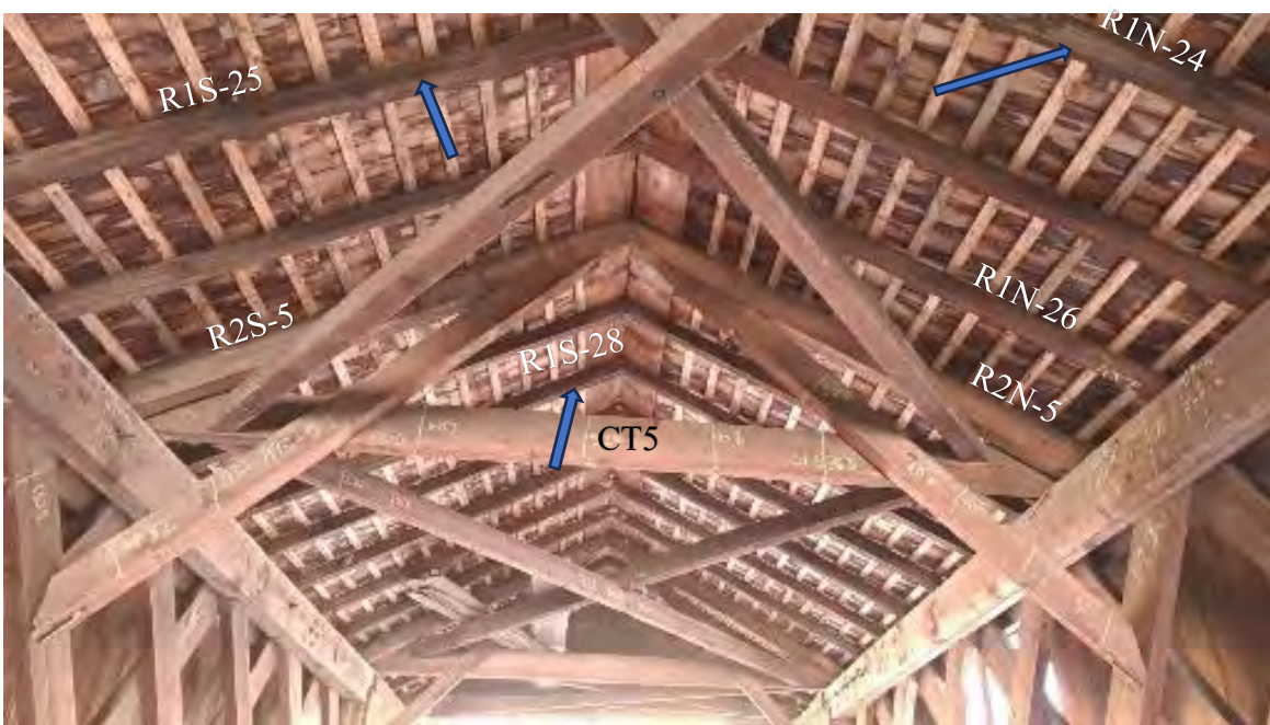
Figure 7-20: R1S-25 has severe shrinkage checks. R1N-24 has cracks, splits and deterioration at the bottom face. R1S-28 has shrinkage checks, cracks and splits.
