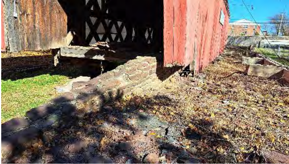
Figure 10-19: The stone wall on the North side of AB2 is in generally good condition away from the original wing wall position.
