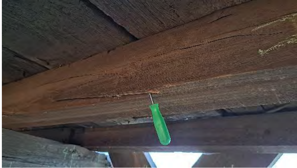
Figure 9-219: J9-2 is decayed on the South side face resulting in splits and section loss with possible internal termite damage for approximately 1/3 width, in very poor condition.
