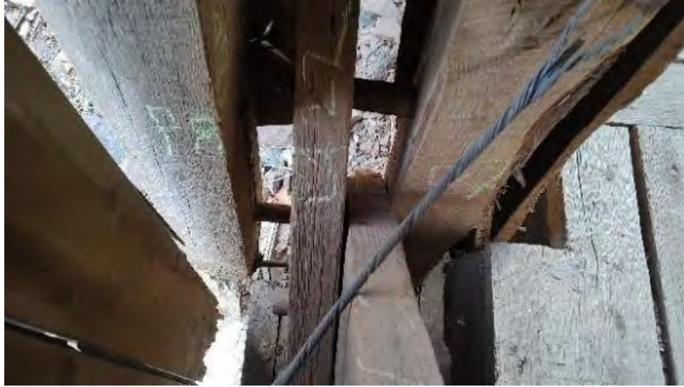
Figure 8-117: The bottom 12-inches of P8 are broken. There is a split up to 3-feet from the bottom and has disconnected from 2 dowels. The dowels are broken.
