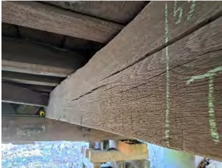
Figure 4-1: Example of moderate shrinkage checks in a transverse beam on the Bridge.
