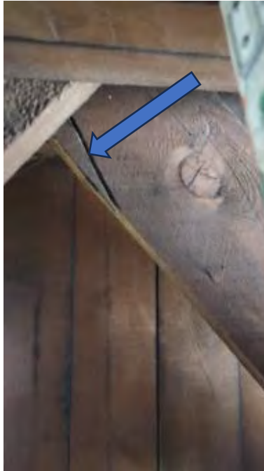
Figure 8-47: L1-4 is broken at the bottom on the outer edge.
