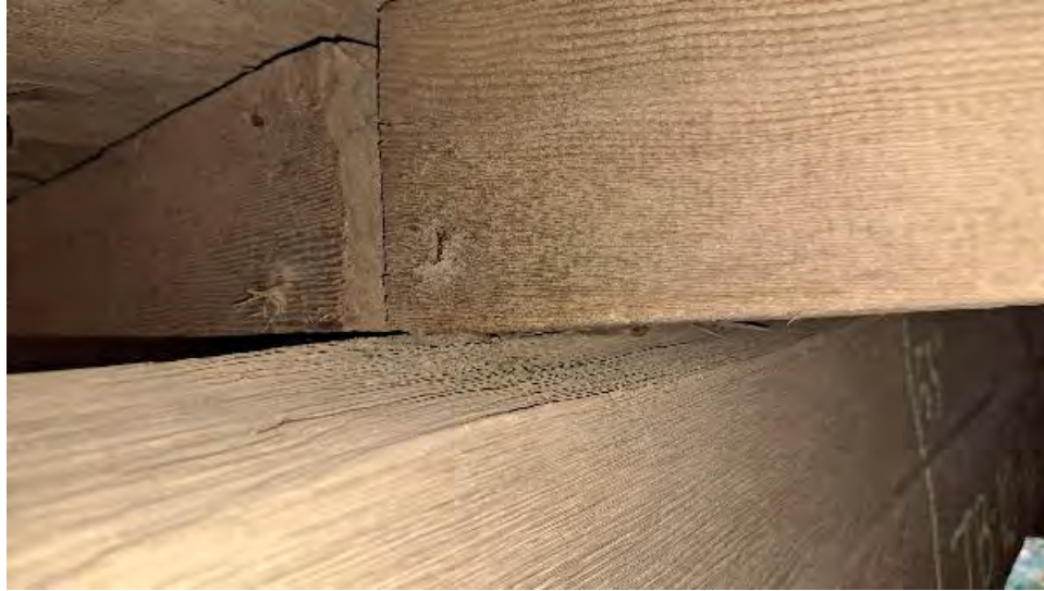
Figure 9-225: J9-4-S is bearing on TB10 for a length of 1/2-inches due to wane on AB1 edge of TB10.
