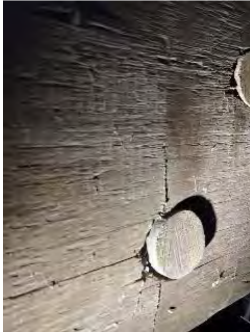
Figure 8-105: L4-17 is cleaved on both rows of dowels at the top chord.
