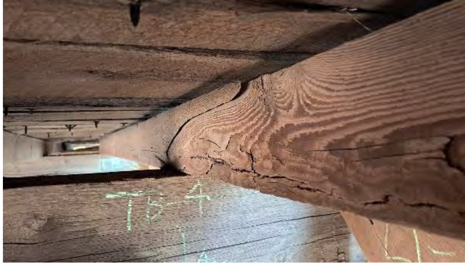
Figure 9-112: J3-1 has large cracks on the South side over TB4 and is continuous with J4-1.
