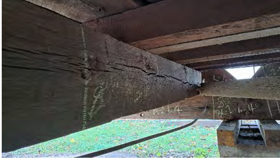
Figure 9-63: TB11 has full length shrinkage checks on the AB1 side that are 1 inch deep.
