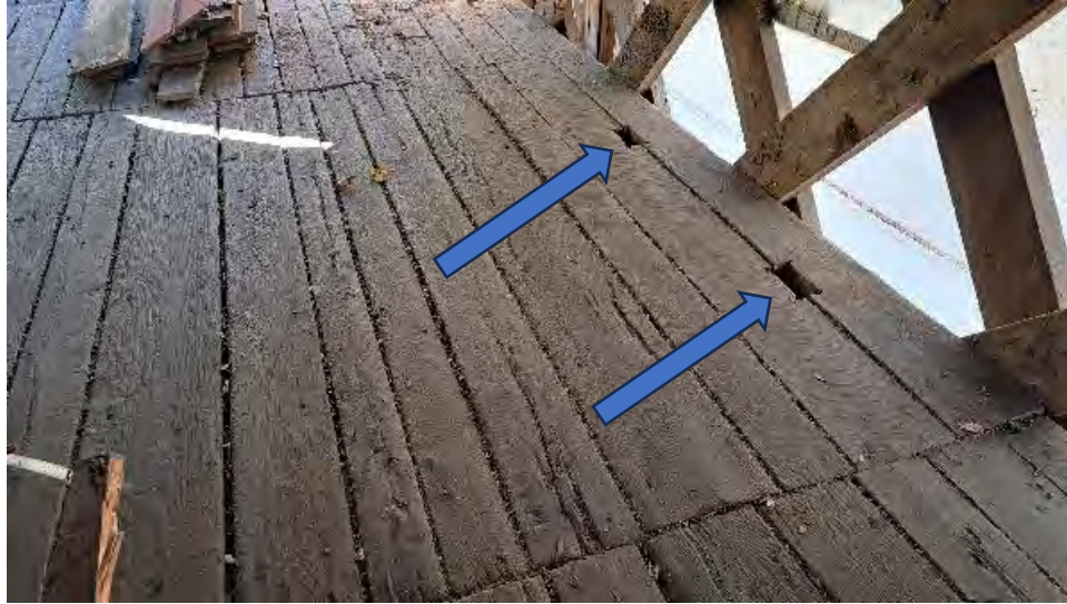
Figure 9-19: Floor decking Span 8, North side, with two common holes in Planks 1 and 2.
