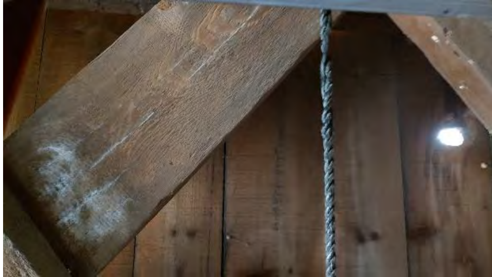
Figure 8-99: L4-7 is cracked through a row of dowels at the connection to L3-7. White surface fungi is seen on L3-7 above this connection. The top dowel does not penetrate through L4-7.
