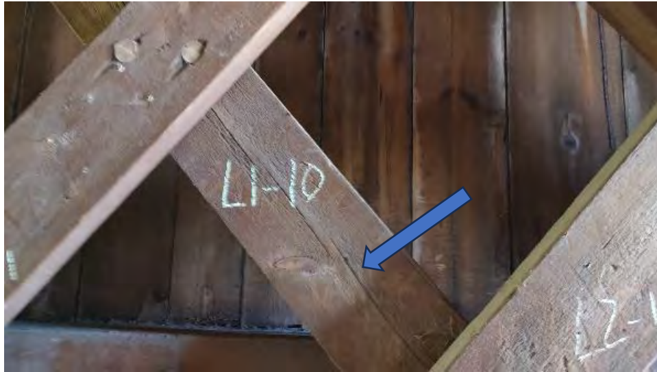
Figure 8-51: Large shrinkage checks exist through L1-10 just above the middle chord.
