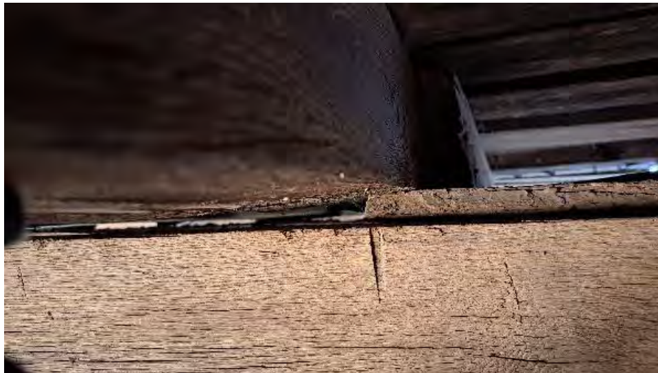
Figure 9-150: J5-2 has partial bearing on a packer over TB6.
