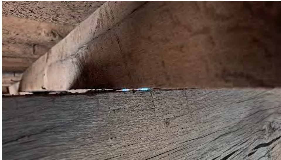
Figure 9-154: J5-4 is not bearing on TB5.
