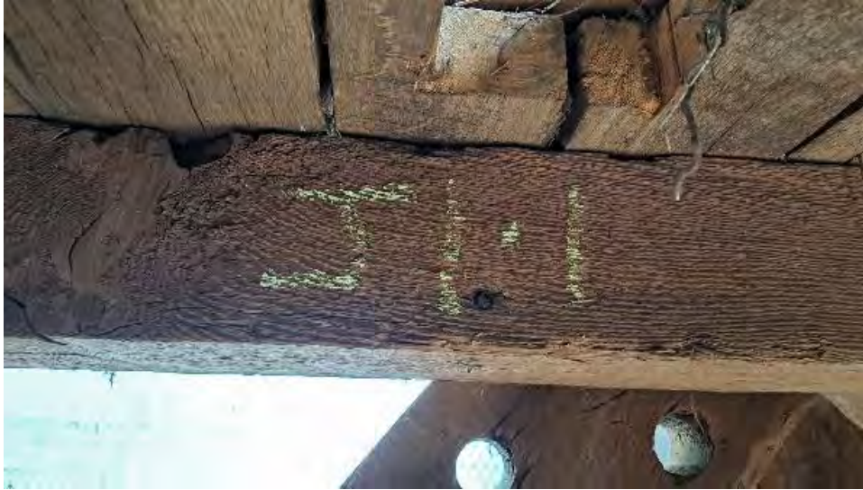
Figure 9-70: Joist J1-1 has some large knots.
