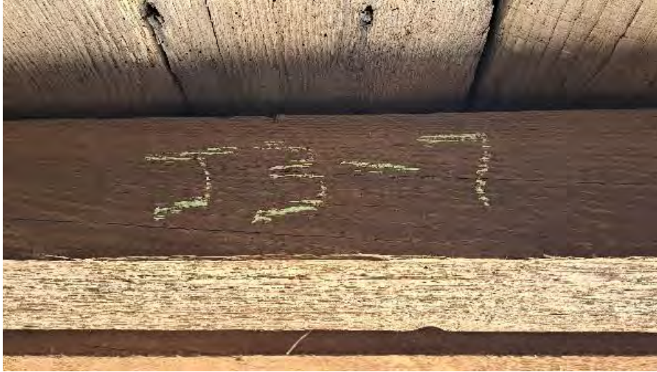
Figure 9-126: J3-7 is in fair condition.
