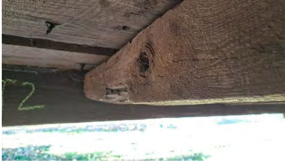
Figure 9-254: J11-4 has some termite damage with major section loss at the bottom face at the AB2 end.
