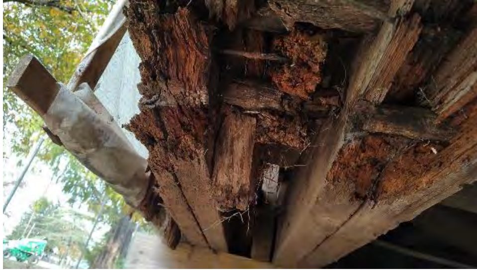
Figure 8-30: Significant decay and section loss to the AB2 ends of BC1 and BC2.
