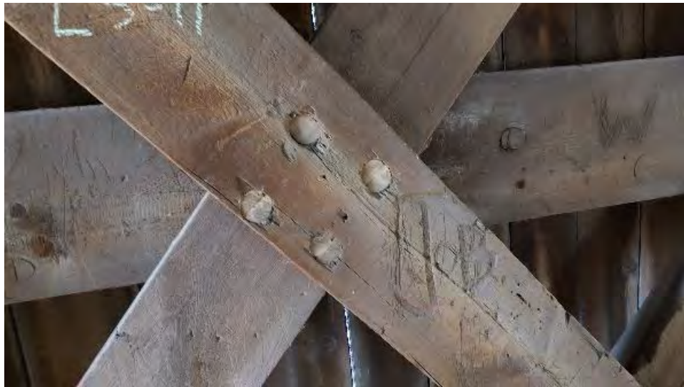
Figure 8-78: L3-11 is cupping on longitudinal alignment on the inside face where pith is evident.
