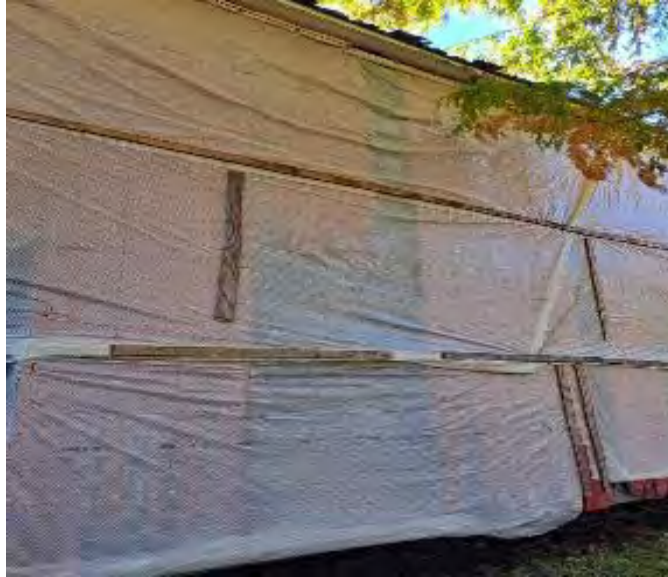
Figure 6-10: Siding on the North side showing missing boards in multiple locations behind the temporary plastic wrapping.
