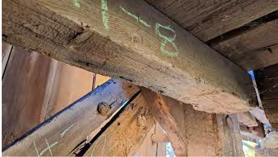
Figure 9-262: Joist J11-8 termite damage to bottom and South faces for most of the length with some minor cracking and damage.
