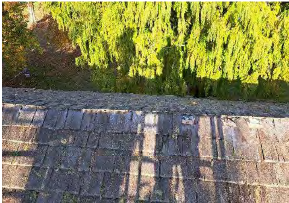
Figure 6-6: A 4x4-inch light-gauge steel cap exists for full length of ridge and located under the upper layer of shakes.
