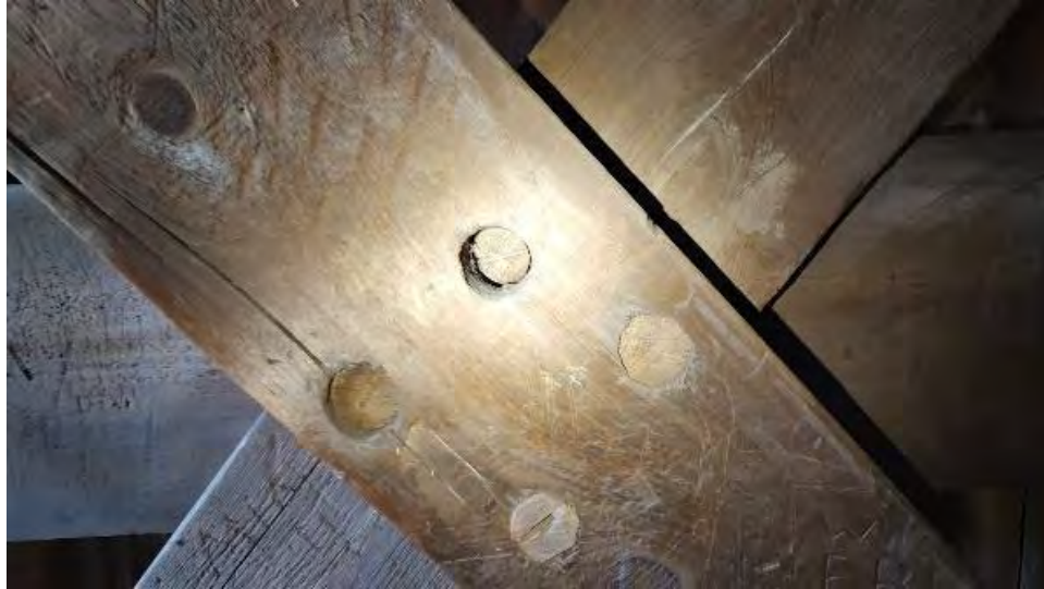
Figure 8-97: L4-7 is cracked through a row of dowels at the connection to L3-7. White surface fungi is seen on L3-7 above this connection. The top dowel does not penetrate through L4-7.
