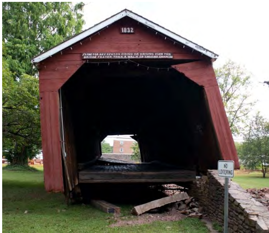
Figure 1-2: A view from Abutment 1 (top) and Abutment 2 (bottom) of the Bridge after the flood event.
