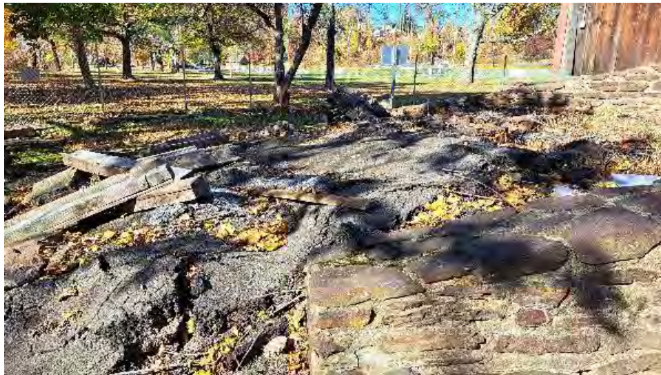
Figure 10-16: The remaining asphalt at AB2 is in poor condition. Loose timber elements are stockpiled at AB2.
