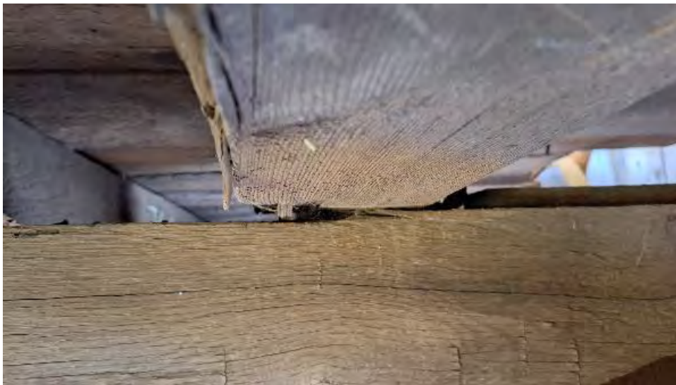
Figure 9-191: J7-7 does not bear onto transverse beams at either end.
