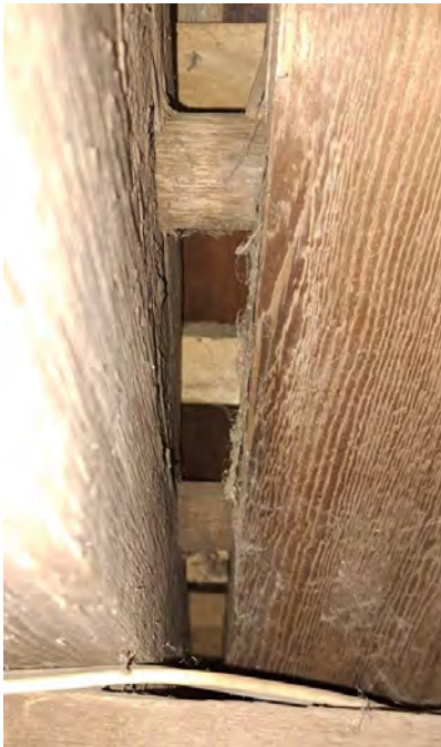
Figure 7-4: Separation of CT4 from the main rafter on the south side.
