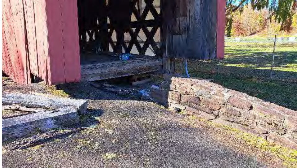
Figure 10-3: The North side of AB1 has approximately 10-foot of stone wall that is dislodged. Backfilling has receded and asphalt surface is damaged.
