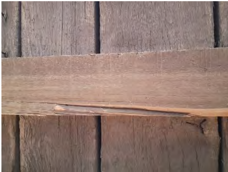
Figure 9-220: J9-2 is decayed on the South face resulting in splits and section loss with possible internal termite damage for approximately 1/3 width, in very poor condition.
