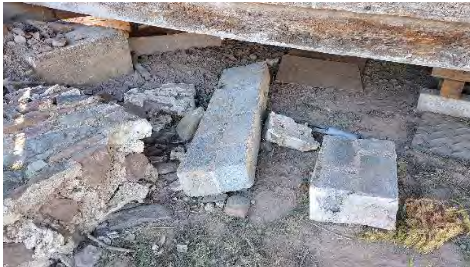
Figure 10-4: Concrete masonry wall segments have been dislodged at AB1. These may have formed the breastwall between the backfill and the timber deck.
