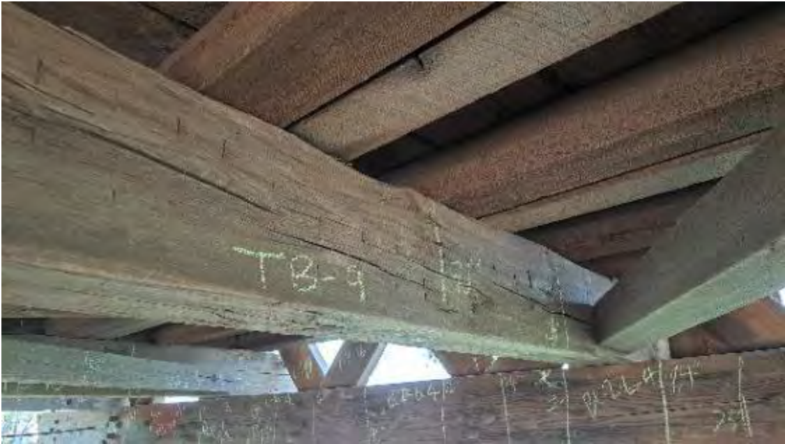
Figure 9-55: TB9 has shrinkage checks 2-inches deep and 3/8-inches wide on the AB1 side at the North end.
