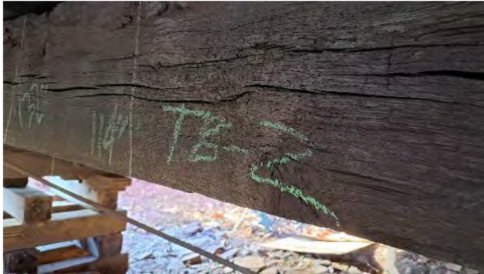
Figure 9-27: Significant shrinkage checking exists to TB2.
