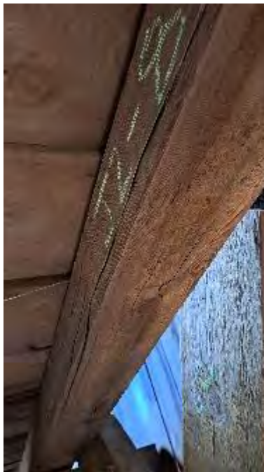
Figure 9-109: J2-8 has vertical cracks to the bottom face, extending to the North side.
