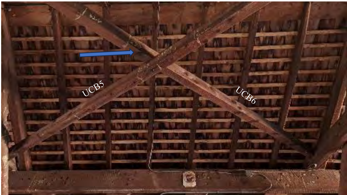
Figure 7-10: Upper cross braces UCB5 and UCB6 with a split 2-inches from middle of UCB6.
