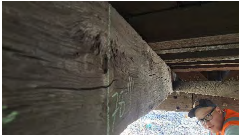
Figure 9-58: TB9 has large knots on the bottom face at 1/3, 1/2, and 2/3 span locations. Planer skips and chisel scars exist on all visible sides. Shrinkage checks exist on the bottom face.
