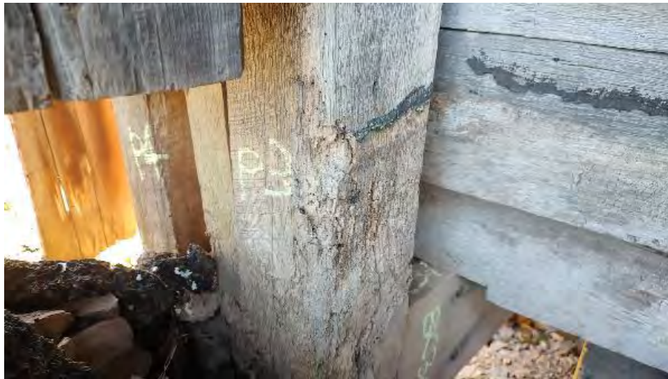
Figure 8-112: P3 is in very poor condition with decay extending 30-inches from the bottom.
