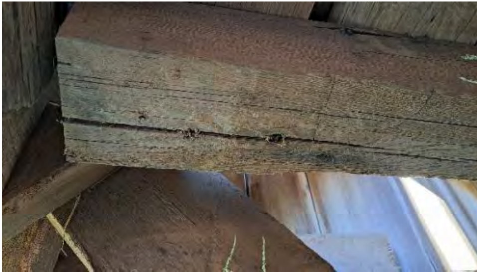
Figure 9-247: J11-1 has a vertical split 16-inches long at the AB2 end, with some additional minor splitting at its top South edge.
