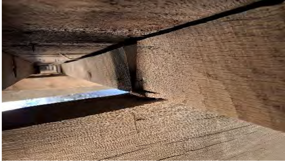
Figure 9-142: J4-6-S has a short end split due to cleaving of skew nail to TB5.
