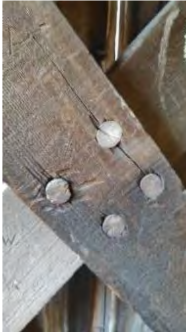
Figure 8-73: L3-4 is cracked at the dowels to the middle chord.
