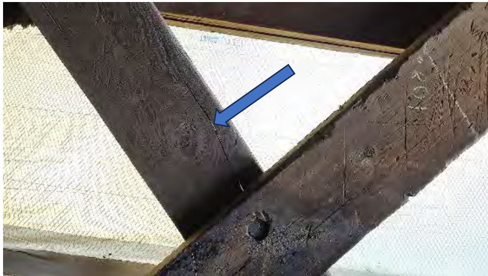
Figure 8-50: L1-4 is split through a dowel hole with a Lattice 2 member.
