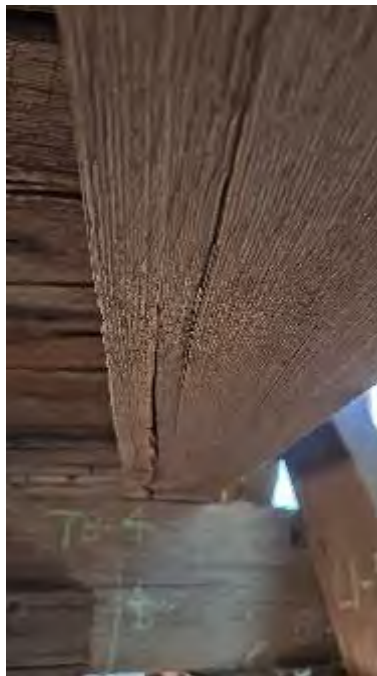
Figure 9-111: J3-1 has bottom face vertical splits.
