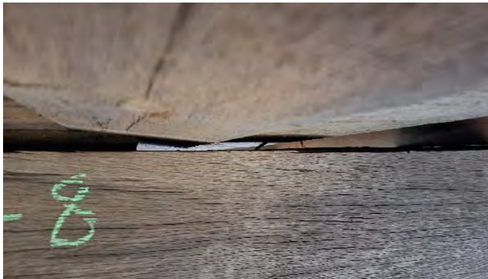
Figure 9-203: J8-5-S is not bearing on TB8.
