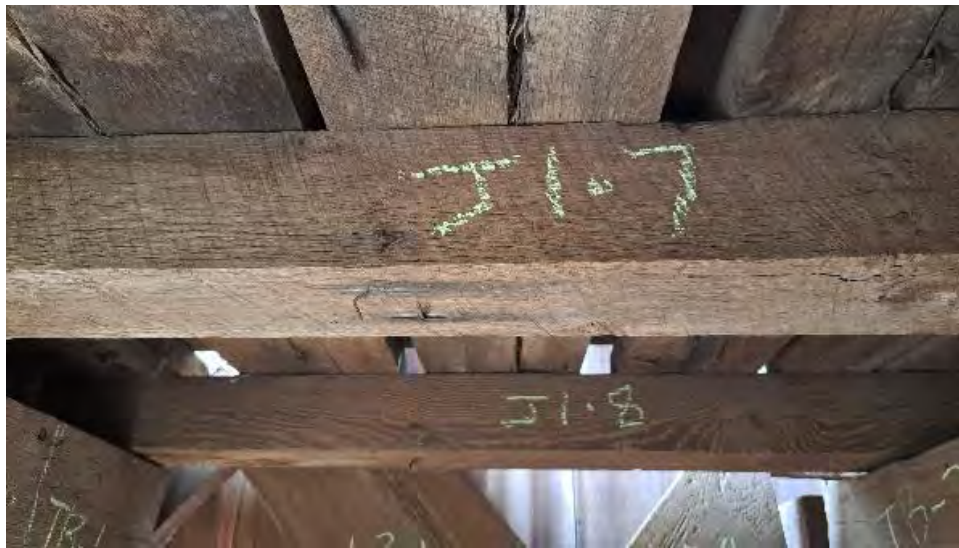
Figure 9-85: J1-7 is in fair condition and is continuous with J2-7.
