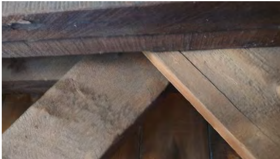
Figure 8-74: L3-6 is split from the dowel connection at the top chord.
