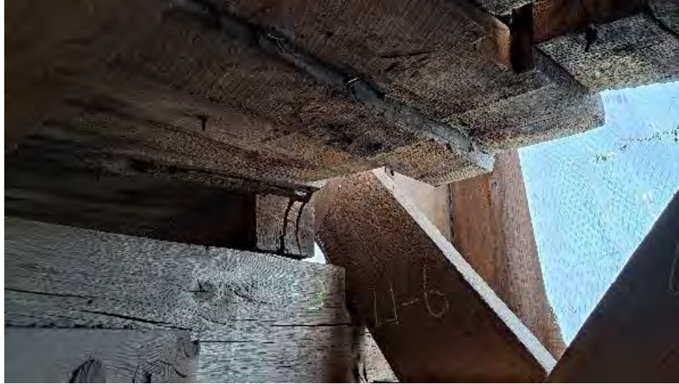
Figure 9-90: J2-1 is missing.
