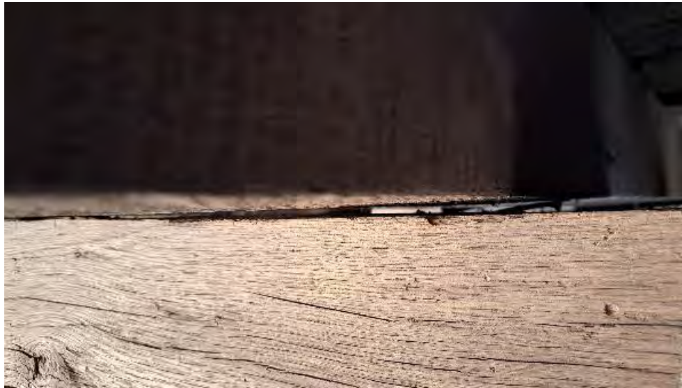
Figure 9-152: J5-3 is not bearing on TB6.
