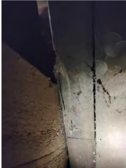
Figure 8-10: Small crack on bottom face of TC1B.
