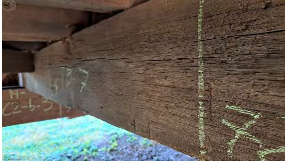
Figure 9-48: TB7 has planer skips, chisel scars and a large knot on the AB2 side, to the lower edge at 1/3 span location from the North end.
