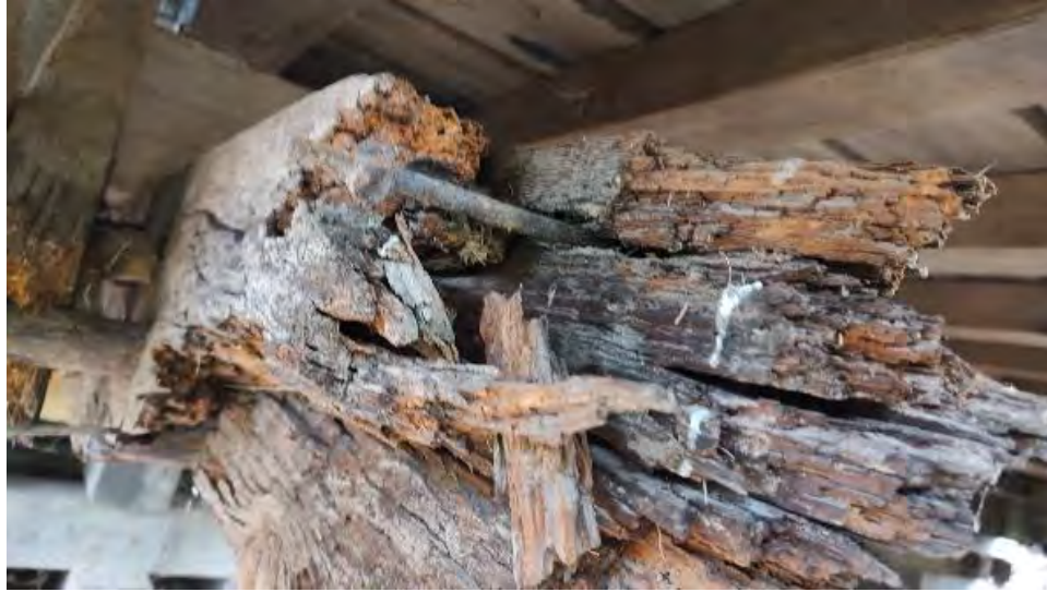
Figure 8-32: Significant decay and section loss to the AB2 ends of BC1 and BC2.
