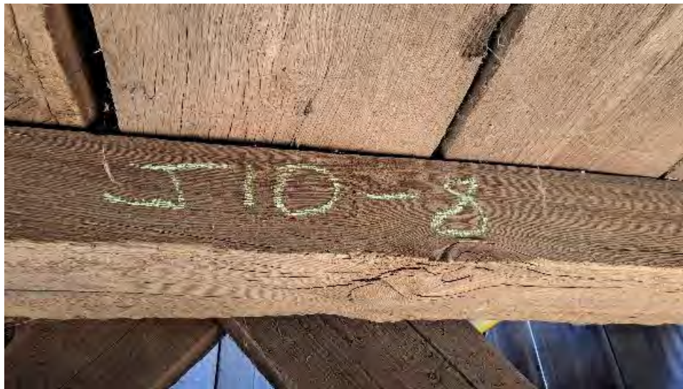
Figure 9-245: J10-8 has a large knot and cracks on its bottom and North side face at mid span.
