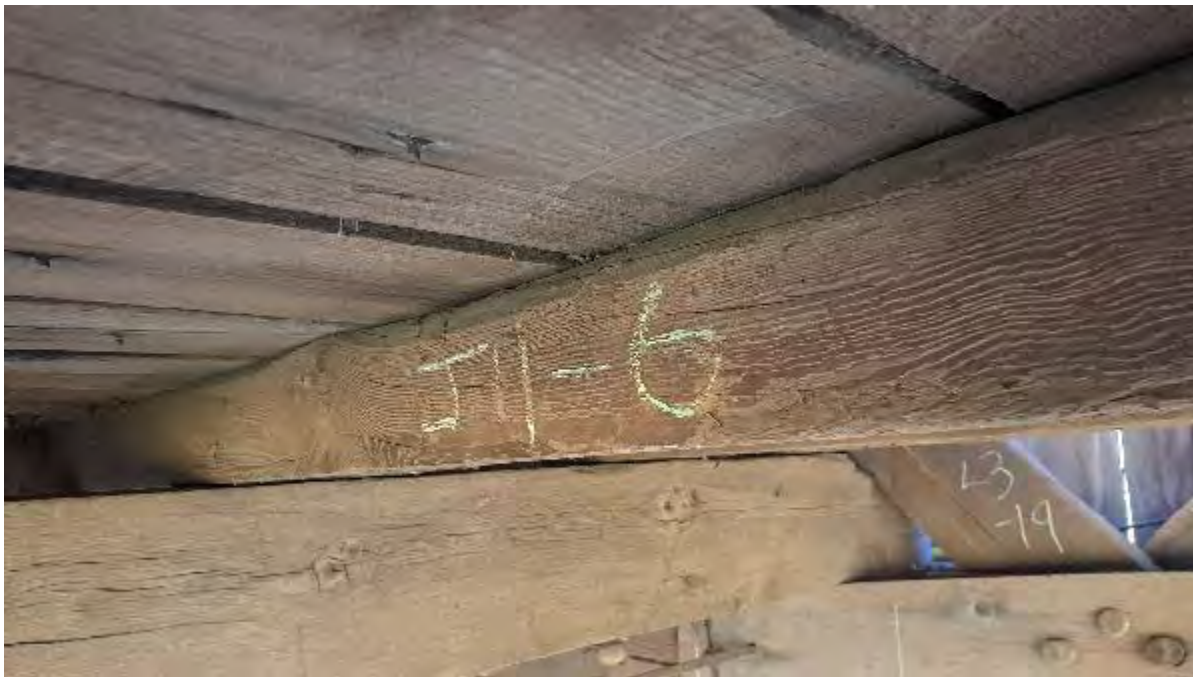
Figure 9-257: J11-6 has wane on the top North edge from TB11 to midspan.
