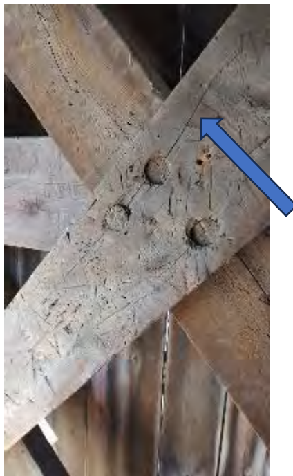
Figure 8-66: L2-20 has shrinkage checks through the dowelled connection to the middle chord and Lattice 1 member.
