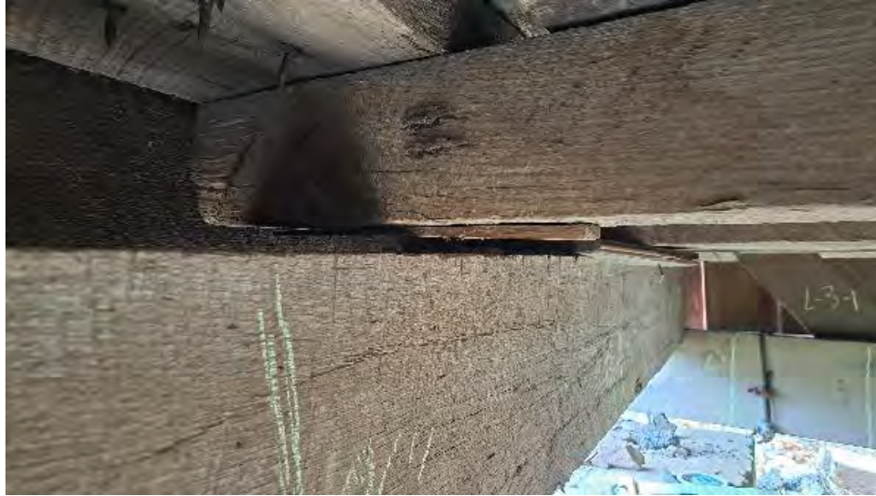
Figure 9-80: J1-5-N is wedged above TB1 but is not in contact with TB1 or TB2.
