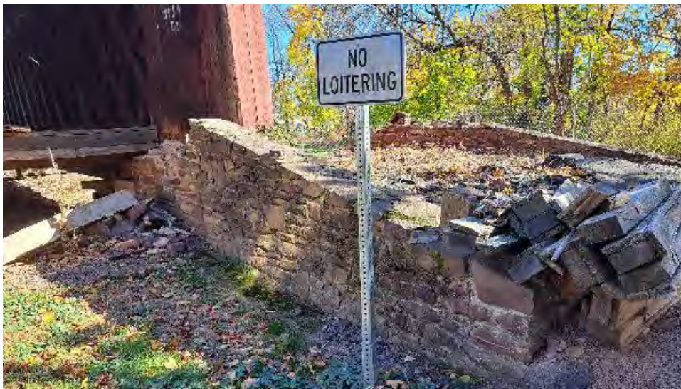
Figure 10-20: The stone wall on the North side of AB2 is in generally good condition away from the original wing wall position. Loose timber elements are stockpiled at AB2.
