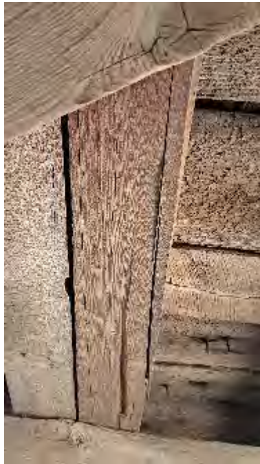
Figure 9-119: J3-4-S has a large split at the TB3 end on its South edge for 3-feet length.
