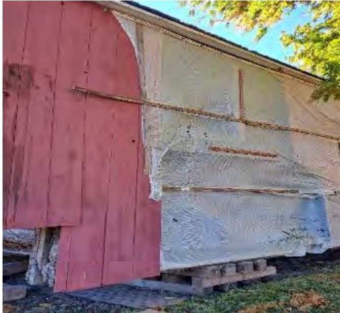
Figure 6-8: Siding on Northeast side showing missing boards in multiple locations behind the temporary plastic wrapping.
