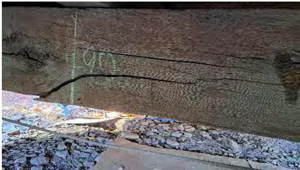
Figure 9-28: TB2 is broken, extending from the bottom face at mid span and caused by extreme slope of grain around a large knot on the side face.
