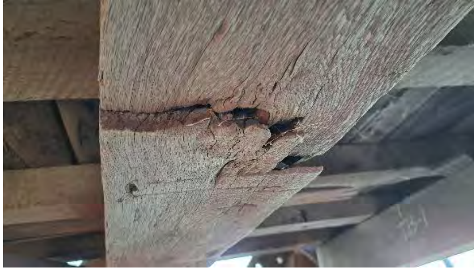
Figure 9-29: TB2 is broken, extending from the bottom face at mid span and caused by extreme slope of grain around a large knot on the side face.
