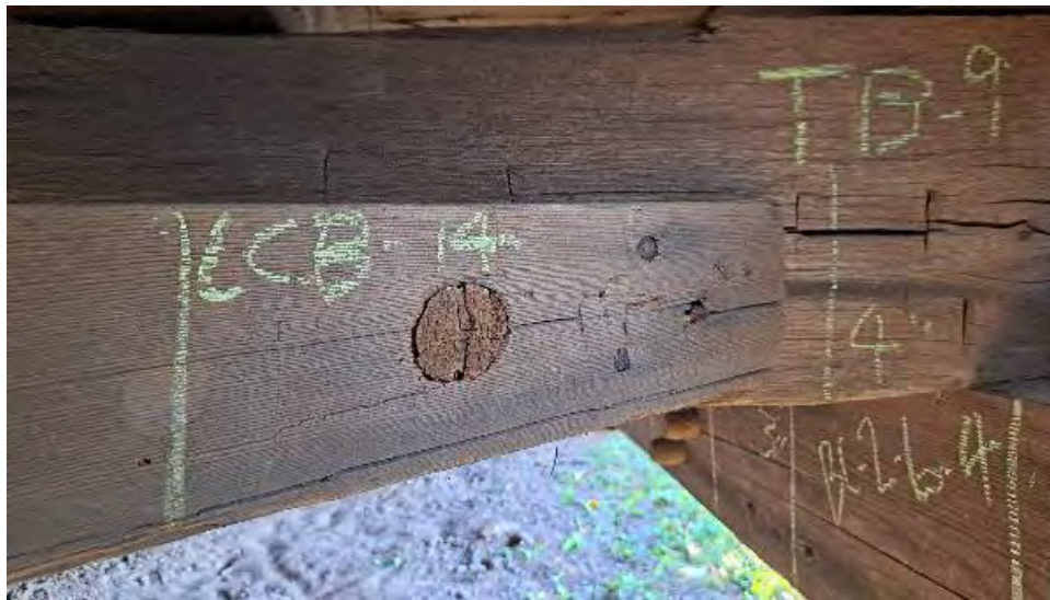
Figure 9-286: LCB-14 has minor cleaving of the dowel and spikes to TB9.
