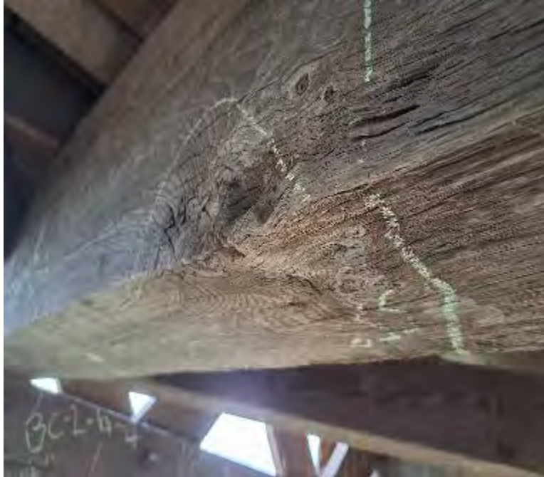
Figure 4-3: Knot on bottom face of a transverse beam
