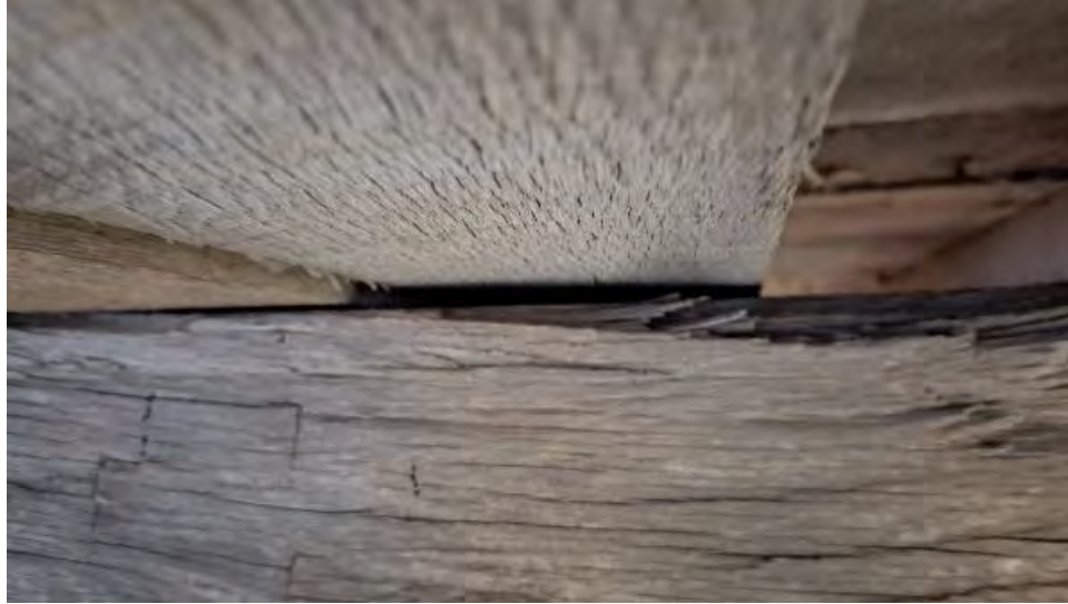
Figure 9-202: J8-4-N is not bearing on TB9.
