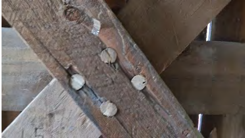
Figure 8-77: L3-9 is cracked through 1 row of dowels to the middle chord.
