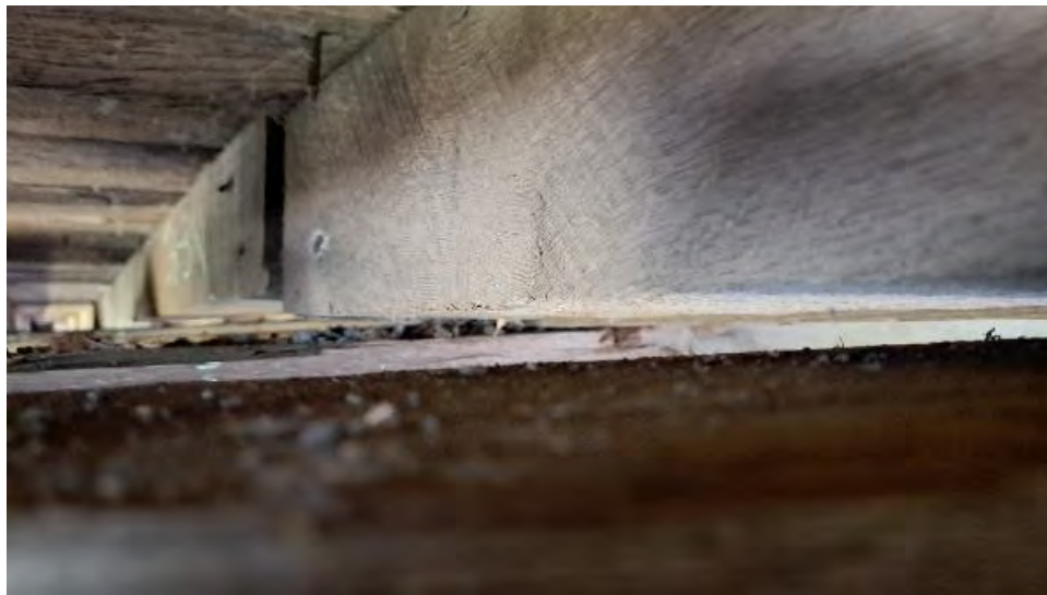
Figure 9-181: J7-3-N is not bearing on TB7.
