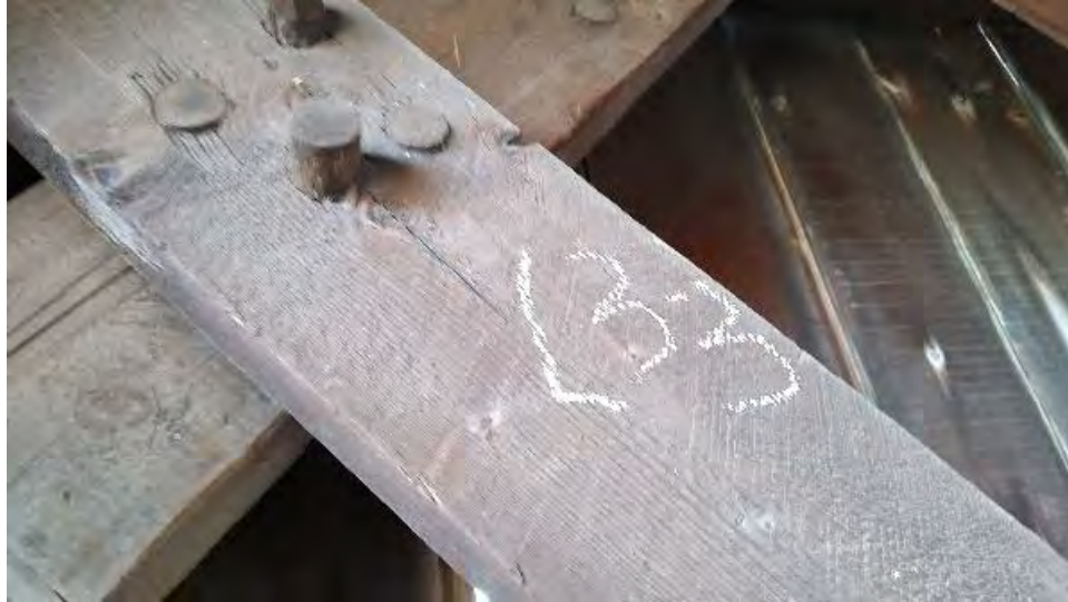
Figure 8-71: L3-3 is cracked at the dowels with L4-1 (note protruding dowels).
