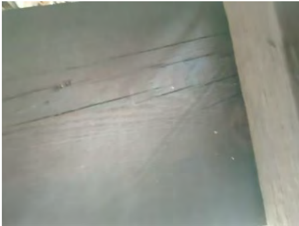
Figure 8-72: L3-3 is cracked at the dowels with L4-1.
