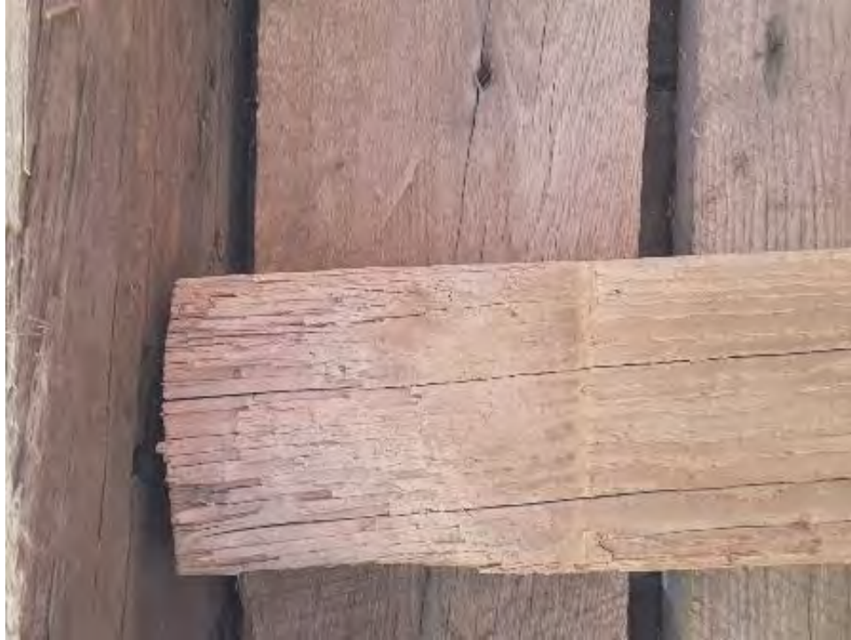
Figure 9-250: J11-3 has feathering at the bottom face at AB2 end.
