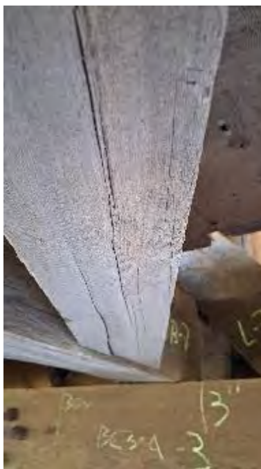
Figure 9-283: LCB-12 has an end split on its bottom face at TB7 end.
