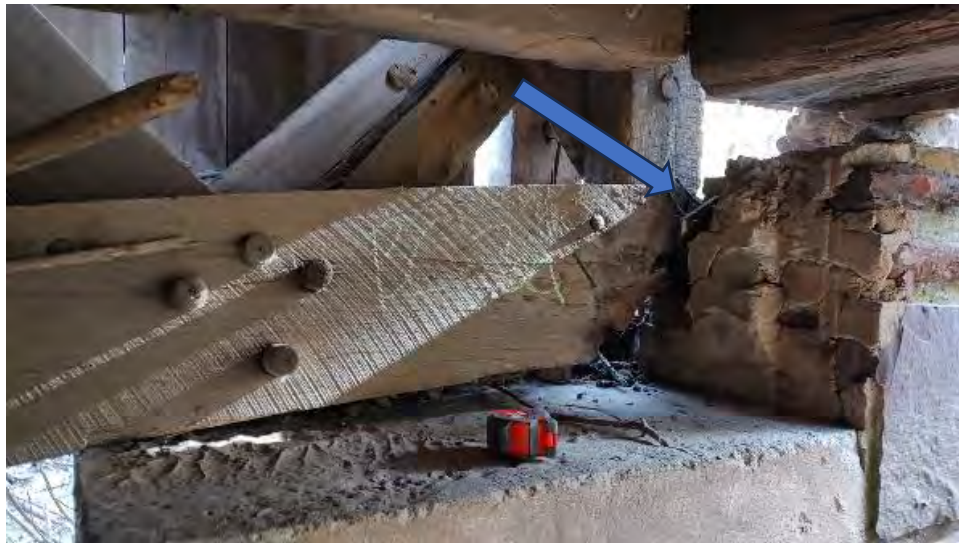
Figure 8-33: Approximately 80% of section loss exists for the first 10-inches of BC3A from P5. Segment 2 is cleaved with a split at 54-inches next to a lattice dowel joint.
