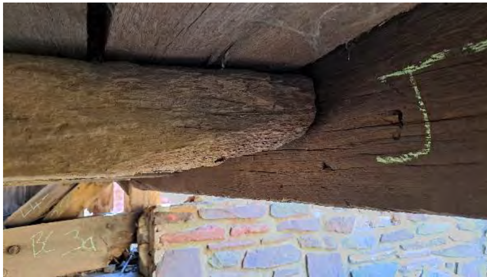
Figure 9-255: J11-5 has some termite damage and some section loss at bottom and South faces at the AB2 end.
