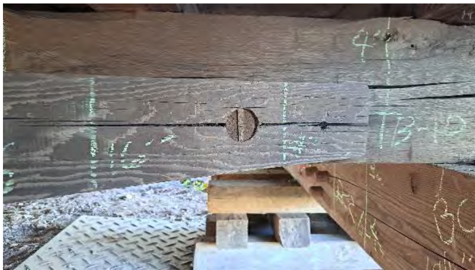
Figure 9-290: LCB-16 has cleaved on the dowel to TB10, resulting in a 2-foot long crack.
