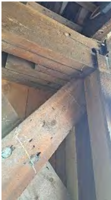
Figure 8-11: TC2B is cleaved through a peg hole (no peg) above post P2 and at a peg hole located 10-inches from P2.
