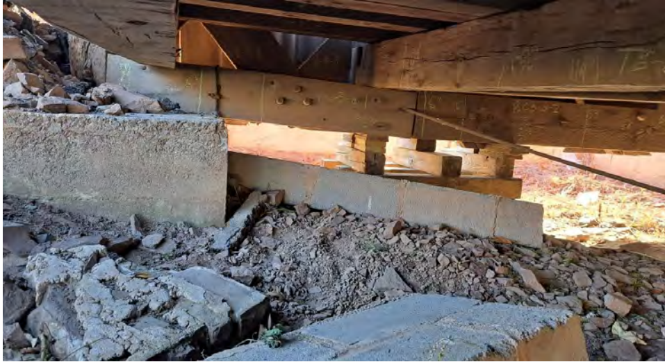
Figure 10-5: Concrete masonry wall segments have been dislodged at AB1. These may have formed the breastwall between the backfill and the timber deck.
