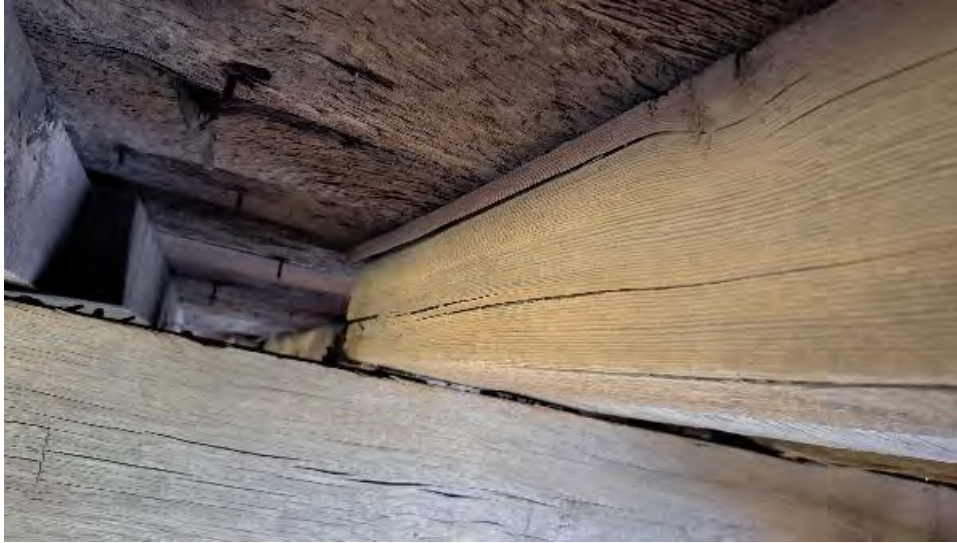
Figure 9-190: J7-6-S has some cracking on the South side near TB7 and is not bearing on TB7.
