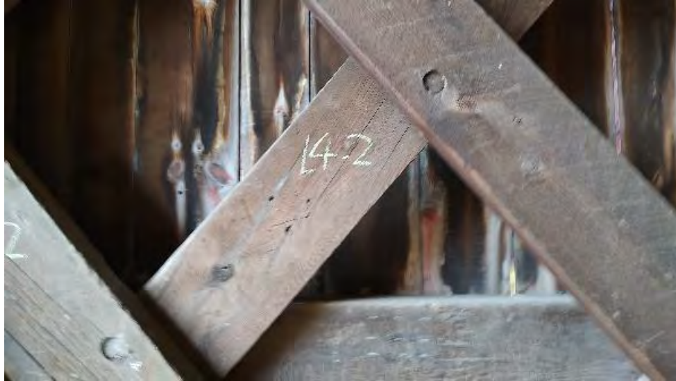
Figure 8-91: L4-2 is cracked either side of the connection to L3-2 and with shrinkage checks through 1 row of dowels.
