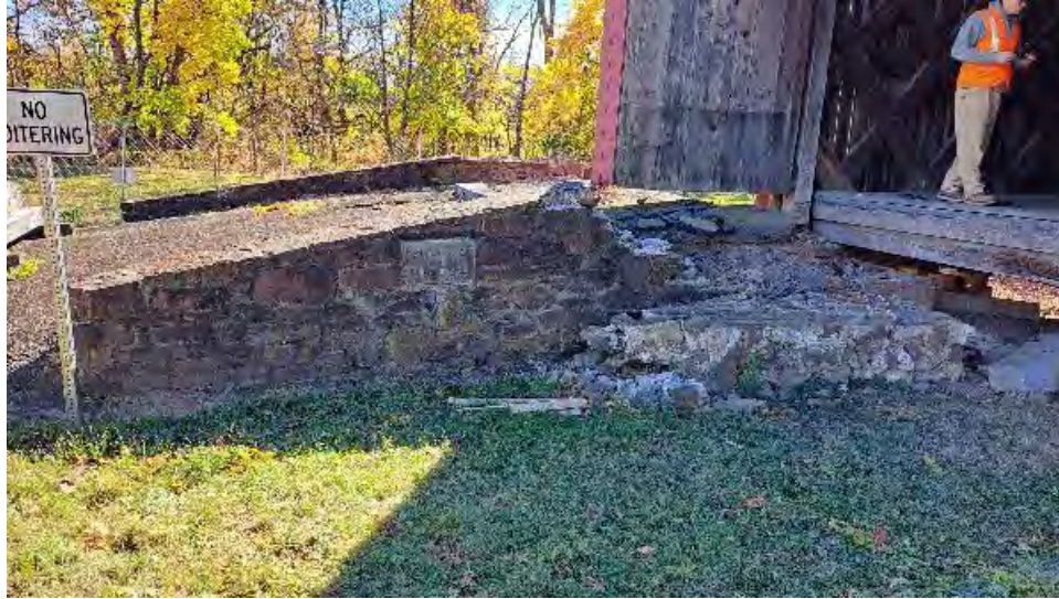
Figure 10-1: The North side of AB1 has an approximately 10-foot length of stone wall dislodged. Backfilling has receded and the asphalt surface is damaged.
