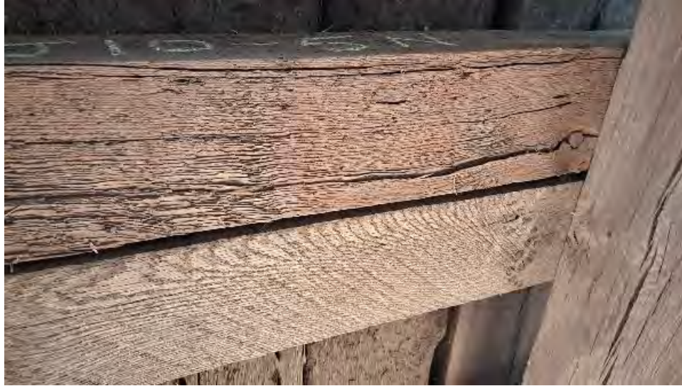
Figure 9-240: J10-5-N has heavy abrasion/section loss to bottom face with significant discontinuity of fiber.
