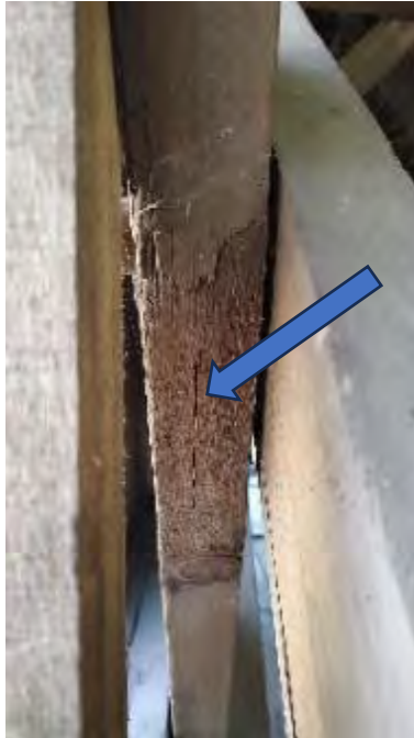
Figure 8-55: L1-18 is cracked on its side and lower edge above the intersection with L2-19.
