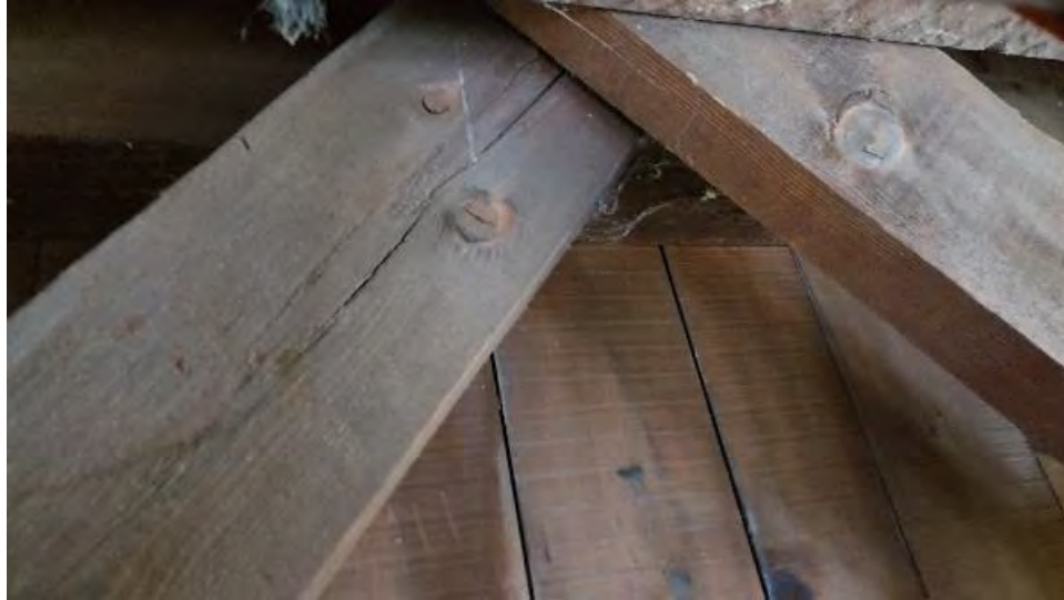
Figure 8-103: L4-16 has split extending from the dowels at the top chord.
