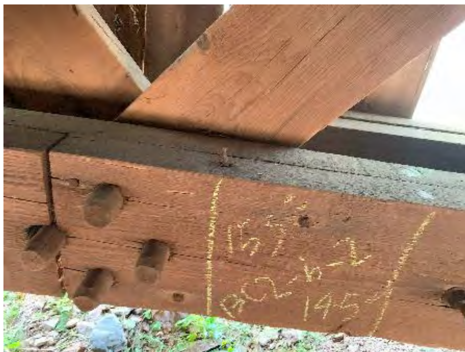
Figure 8-42: Shrinkage checks exist through BC2B splices.
