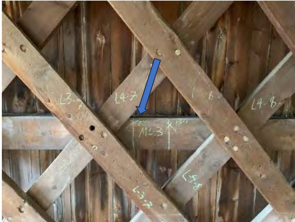
Figure 8-19: MC3 & MC4 has decay 2-inches from lattice member L4-7.
