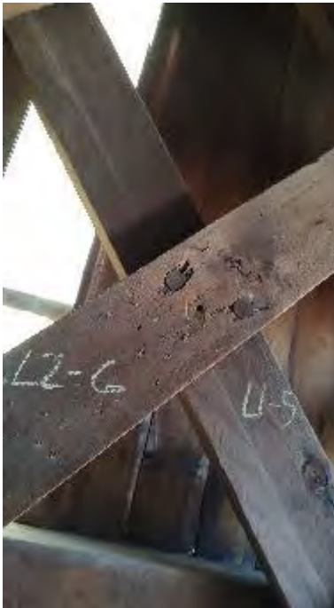
Figure 8-60: L2-6 has some damage at the dowel connection to L1-5.
