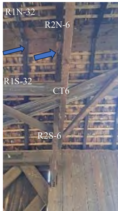
Figure 7-22: R2S-6 and R1N-32 are showing some deterioration on bottom surface.
