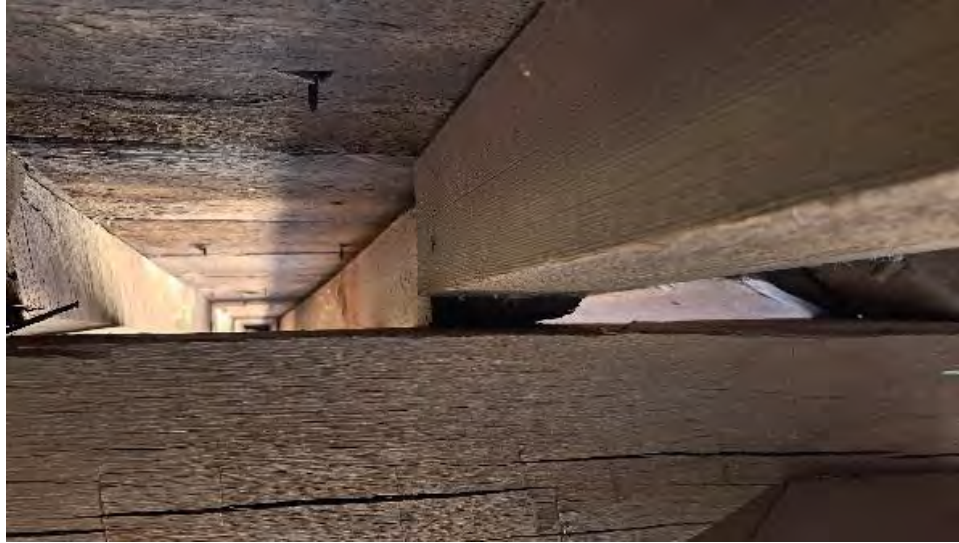
Figure 9-161: J5-7 is not bearing on TB5.
