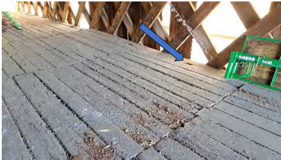
Figure 9-8: Floor decking Span 3, North side, with hole in Plank 2.
