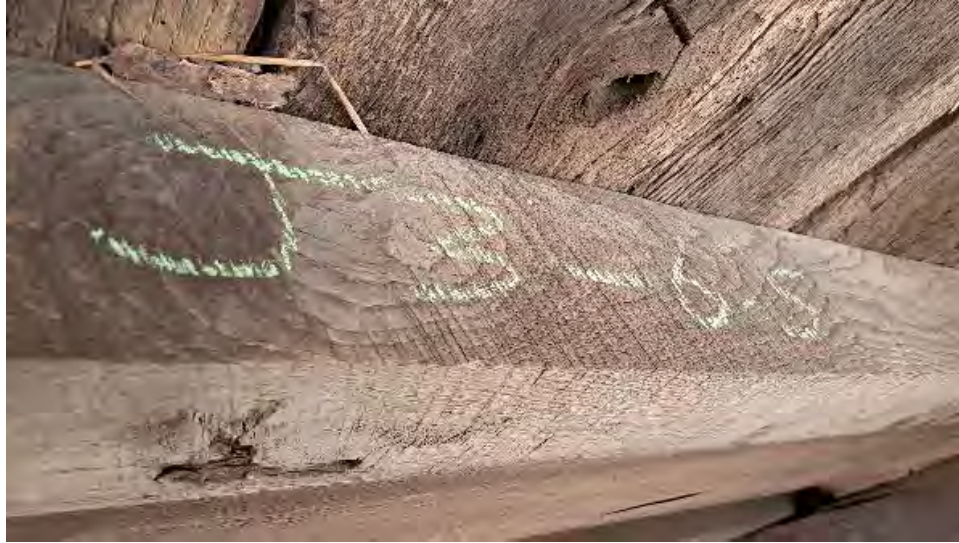
Figure 9-122: J3-6-S has knot holes to bottom face at mid span.
