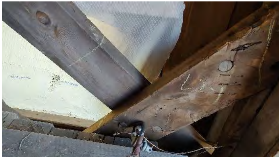
Figure 8-58: L2-1 has some deterioration and abrasion on the outer surface.
