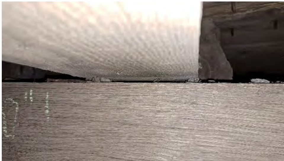
Figure 9-93: J2-2 is not bearing on TB3.
