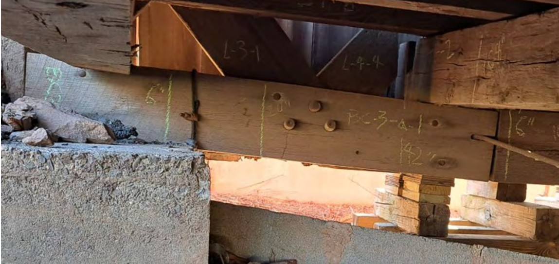
Figure 8-25: BC3A is broken at a dowelled connection to the lattice members L3-1 and L4-4 and is spliced at 61-inches from the end.
