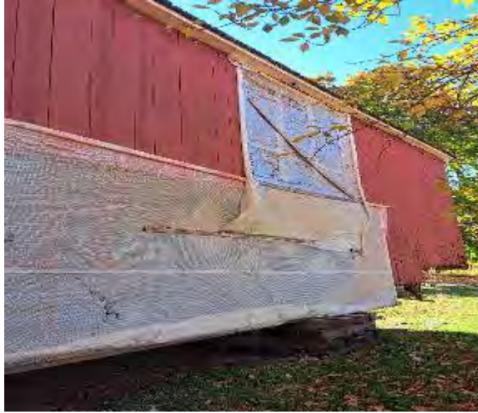
Figure 6-12: Siding on the Northwest side showing missing boards in multiple locations behind the temporary plastic wrapping.
