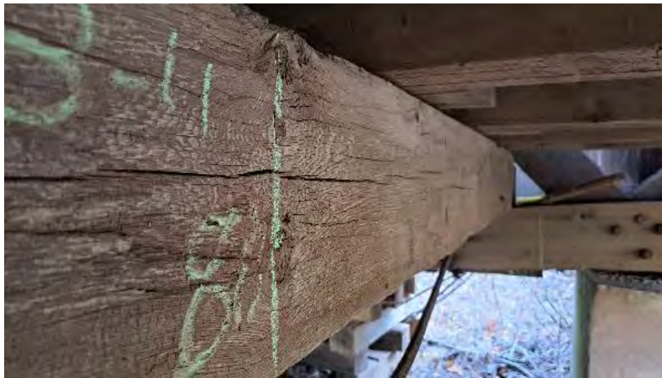
Figure 9-64: TB11 has full length shrinkage checks on the AB1 side that are 1 inch deep.
