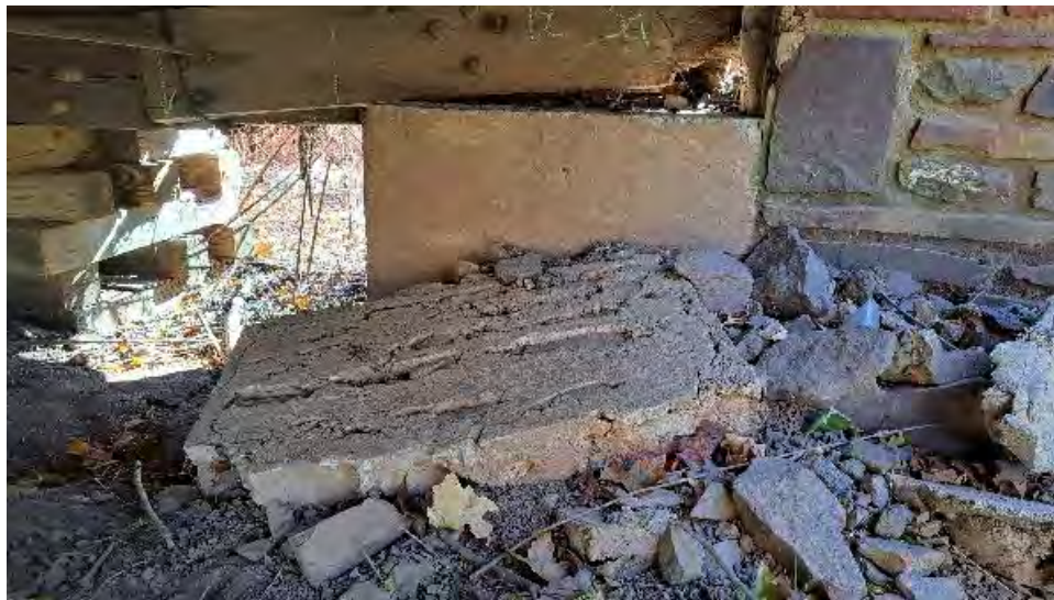
Figure 10-24: Concrete masonry wall segments have been dislodged at AB1. These may have formed the breastwall between the backfill and the timber deck.
