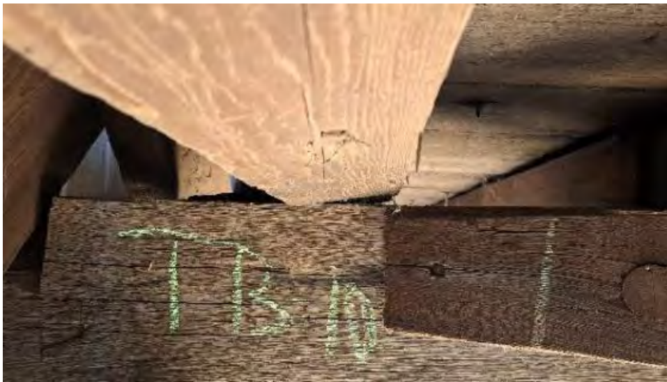
Figure 9-232: J9-8 has end splitting showing its South side only at TB10 end that is 4-feet long. J9-8 is likely cracked on its top surface. There is an end split 8-inches long on its North face from TB10.
