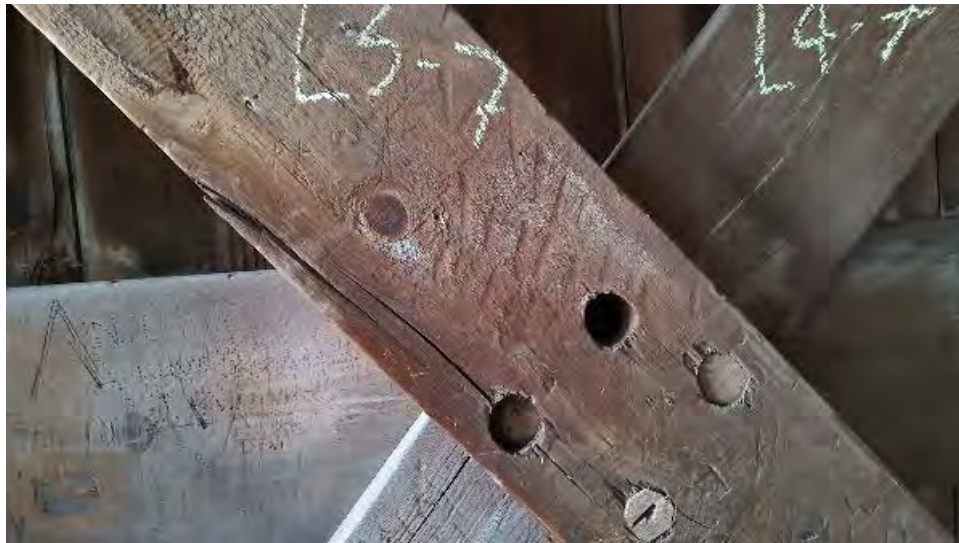
Figure 8-76: L3-7 is cracked at a dowel to L4-7 and the middle chord. The top dowel of this connection does not penetrate through L3-7.
