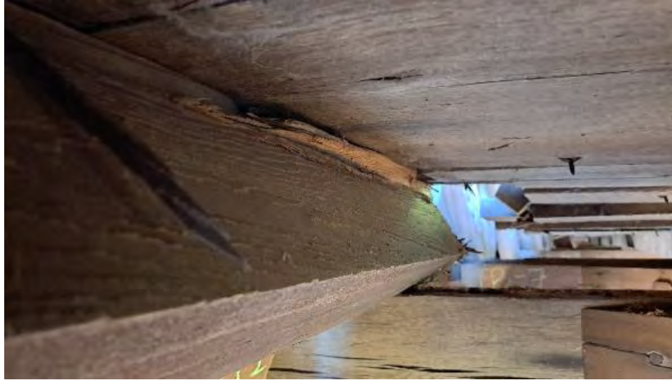
Figure 9-165: J5-8 is crushed on its top North edge for 2-feet from TB6.
