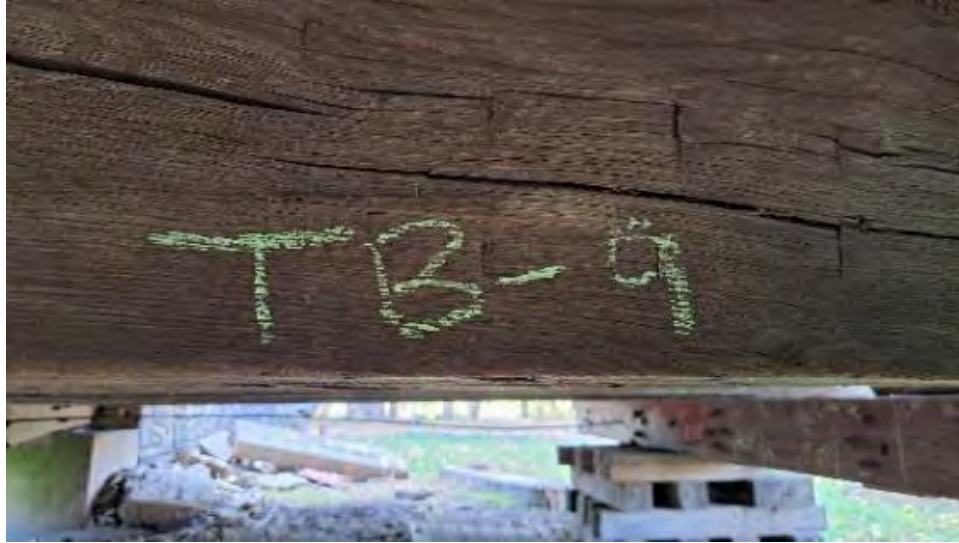
Figure 9-54: TB9 has shrinkage checks 2-inches deep and 3/8-inches wide on the AB1 side at the North end.
