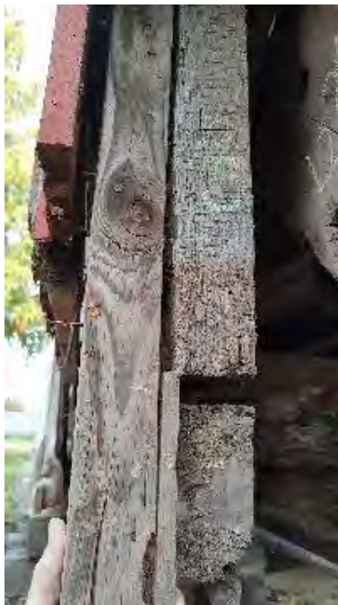
Figure 8-114: P5 has a 2x2 1/2" notch on the BC1A alignment. The bottom 12-inches are missing and the next 16-18- inches are decayed.
