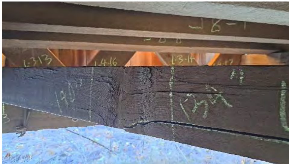
Figure 9-288: LCB-14 has a large knot on the AB1 side that has led to slope of grain cracking.
