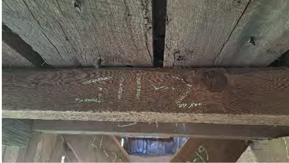
Figure 9-248: J11-2 has a large knot on the South face at mid span, likely extending to the top face with some section loss from slope of grain cracking and wane.
