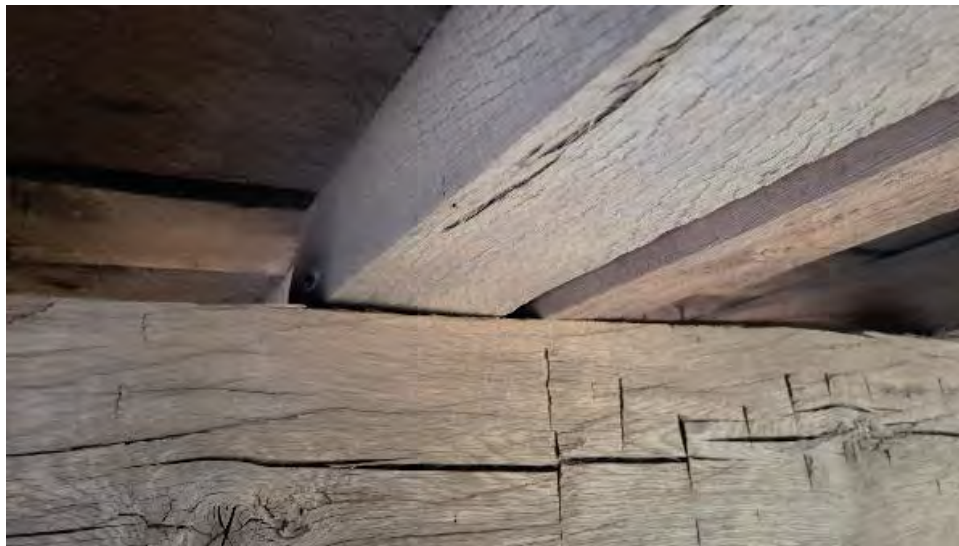
Figure 9-207: J8-5-S is twisted 5 degrees over TB9 and bearing on its North edge only.
