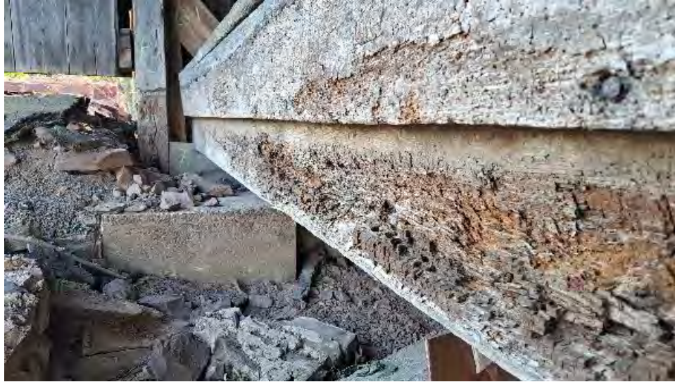
Figure 9-24: TB1 on Abutment 1 side is decayed and section loss up to 2-inches deep.
