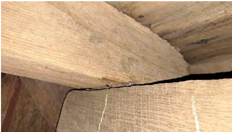
Figure 9-71: J1-1 is decayed on the bottom face at the bearing over TB1.
