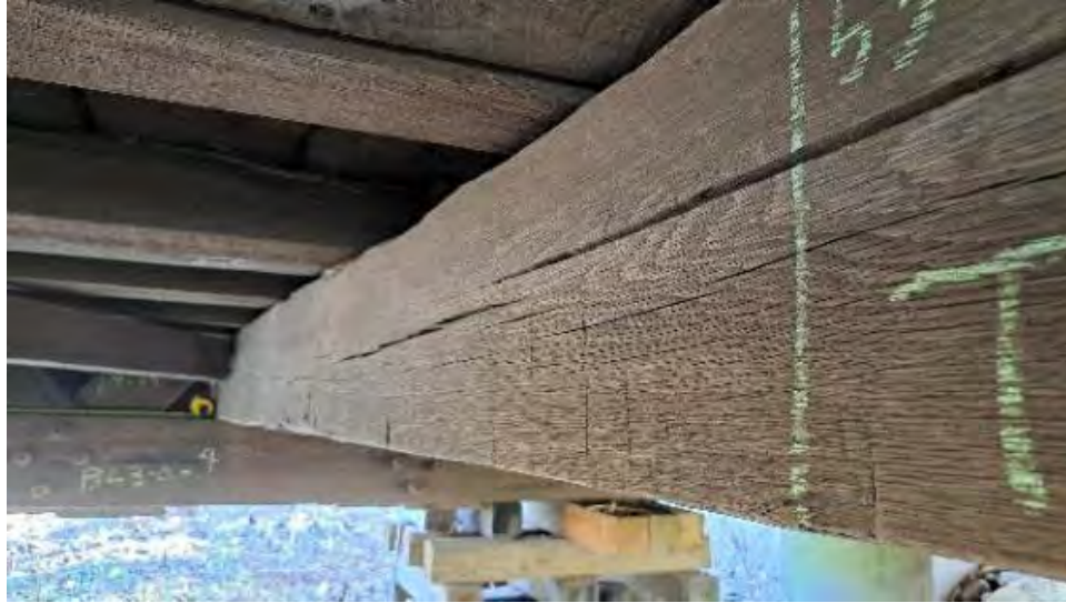
Figure 9-60: TB10 has shrinkage checks 2-inches deep and 3/8-inches wide on the AB1 side, North end.
