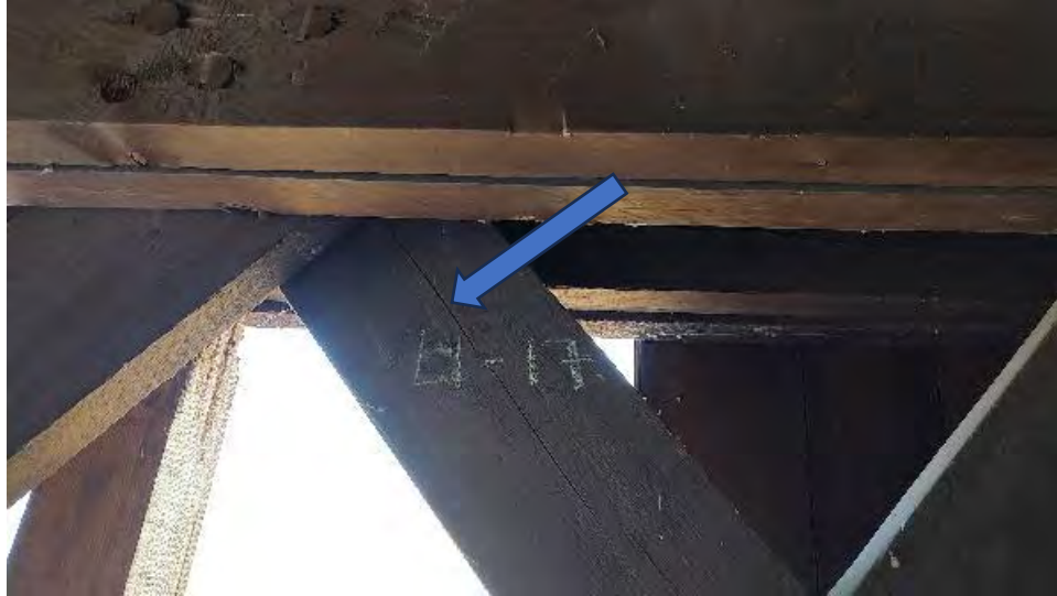
Figure 8-53: Shrinkage checks exist to L1-17 which extend from the dowelled connection with the top chord.
