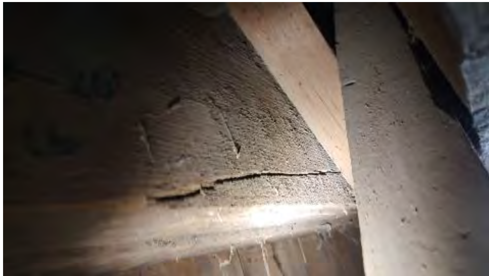
Figure 8-9: Small crack on bottom face of TC1B.
