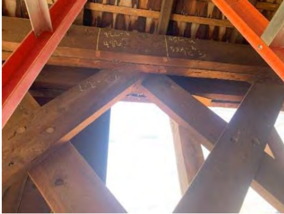
Figure 8-12: TC3A exhibits some shrinkage checks.
