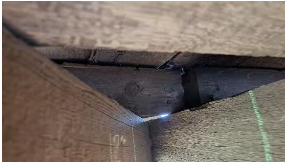
Figure 9-197: J8-2 has more bearing on (LCB13 than on TB8.
