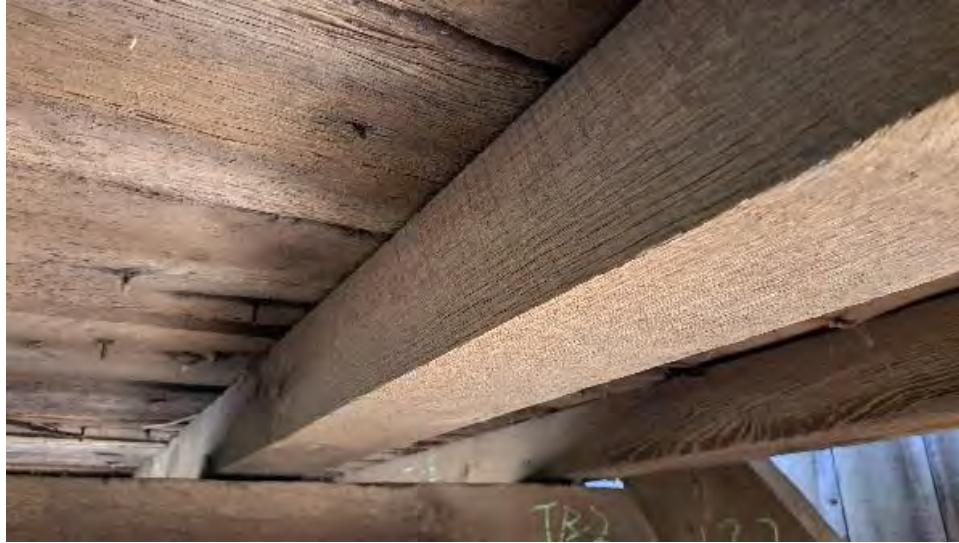
Figure 9-106: J2-7 is not bearing on TB2.
