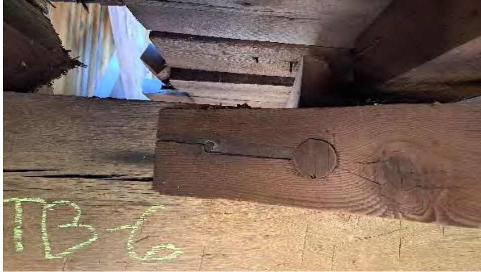
Figure 9-277: LCB-7 has cleaved on the dowel to TB6.
