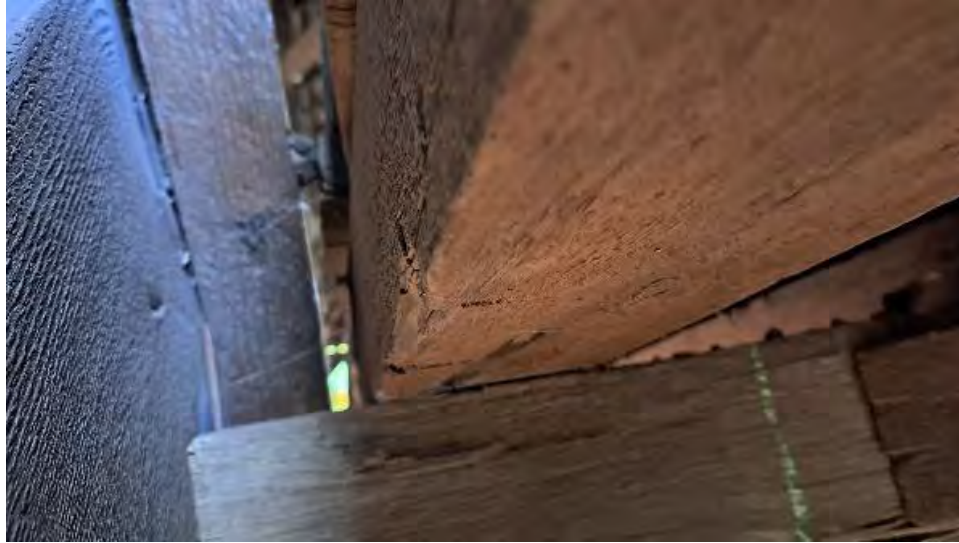
Figure 9-110: J2-8 has section loss and is split on the bottom South edge for 24-inches from TB3.
