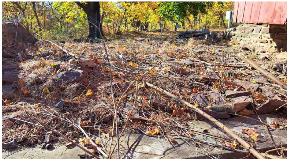
Figure 10-14: The backfilling at AB2 has receded and the asphalt surface is damaged for the full width of AB2. Significant debris exists over the approach.
