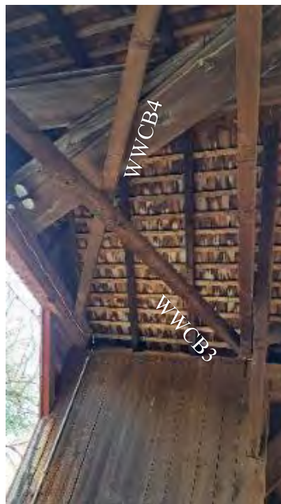
Figure 7-14: Wing wall upper cross braces WWCB3 and WWCB4 are in fair condition.
