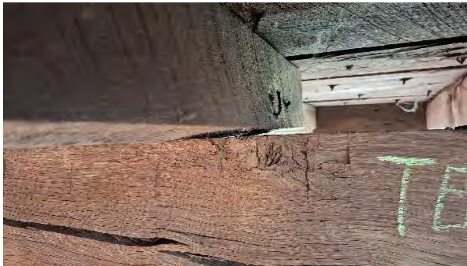
Figure 9-237: J10-3-N is twisted at the TB11 end, with a cupped bottom face and bearing on its South edge only.
