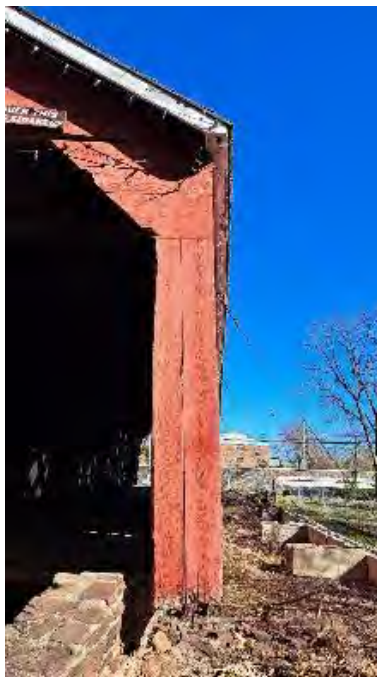
Figure 6-23: Abutment 2 South side front view of siding with some section loss and decay at the bottom.
