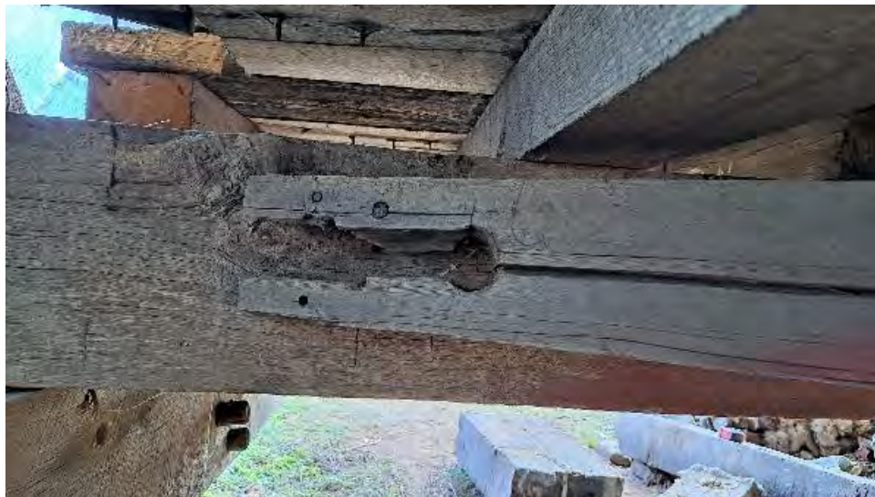
Figure 9-266: The LCB-1 dowel connection to TB2 is destroyed with end split extending to mid span.
