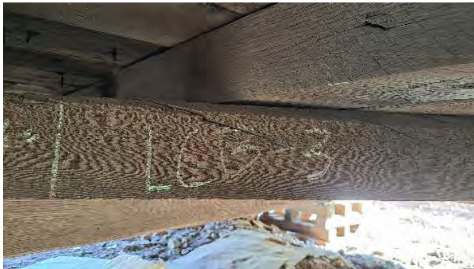
Figure 9-270: LCB-3 has some wane on its top edge facing AB2 with some slope of grain cracking.
