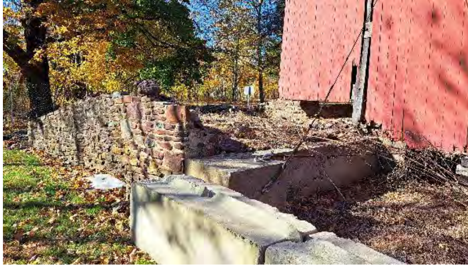
Figure 10-13: The top course of stone is missing for the length of the wing wall at the South side of AB2.
