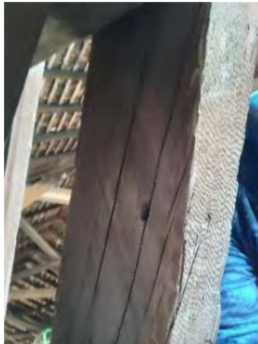
Figure 8-70: L3-2 has several cracks propagating from the dowelled connections to L4-2 & L4-3.
