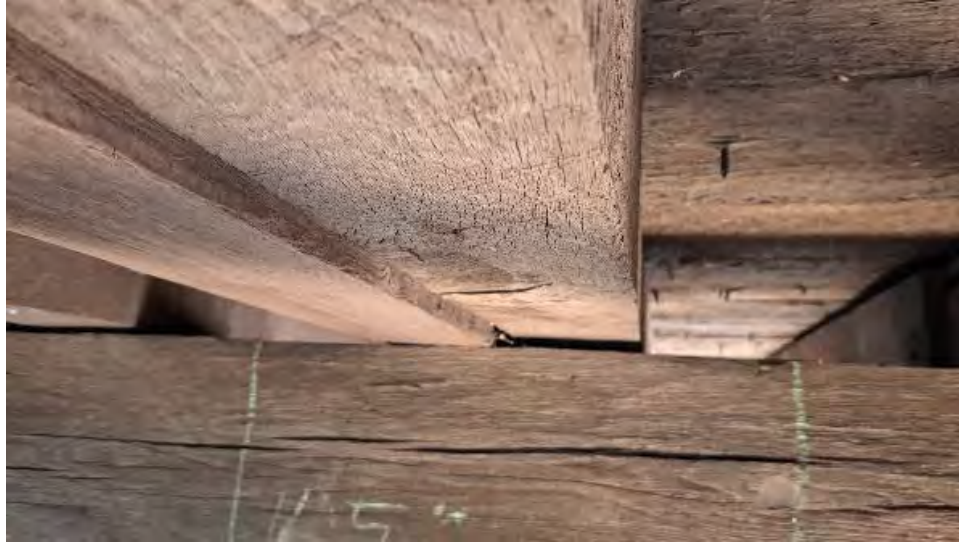
Figure 9-242: J10-6-N has a knot on its bottom face at mid span that is split and is bearing on its South edge only at TB10.
