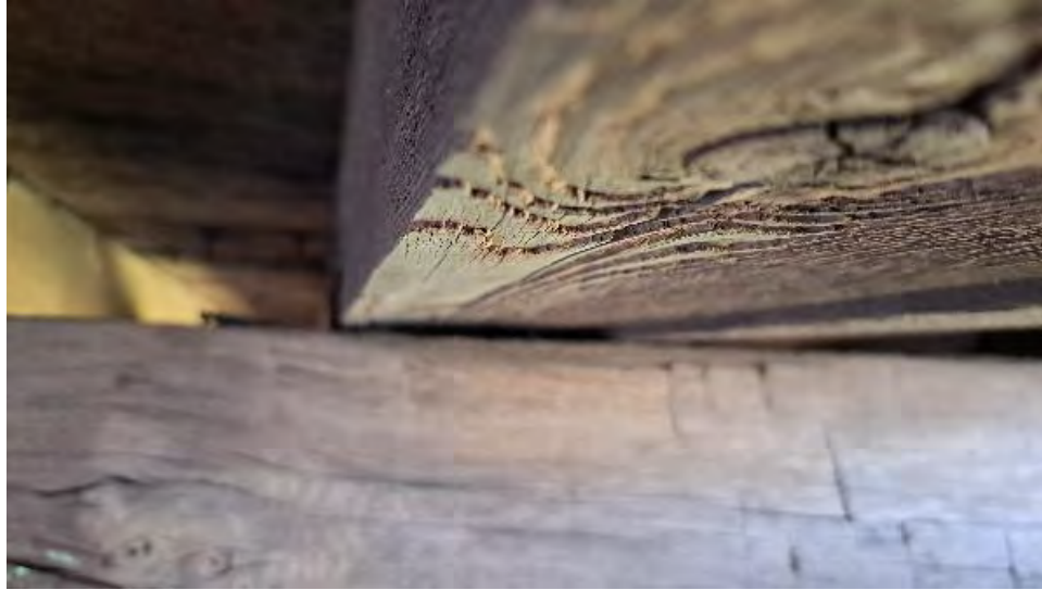
Figure 9-182: J7-3-N is only bearing on the South edge over TB8. J7-3-S is not bearing on TB8.
