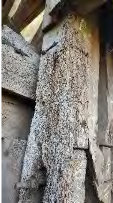
Figure 8-111: P2 is decayed with insect damage and section loss for bottom 3-feet.
