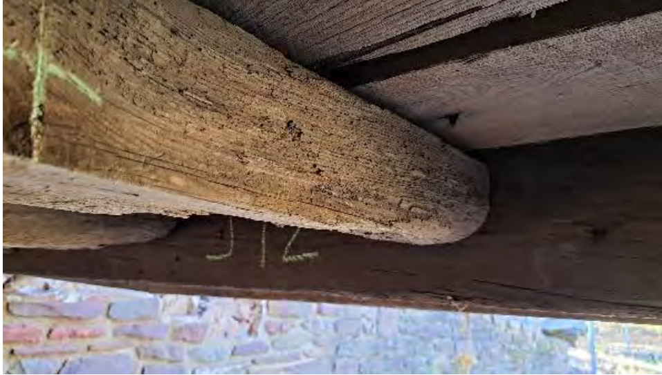
Figure 9-252: J11-4 has some termite damage with major section loss at the bottom face at the AB2 end.
