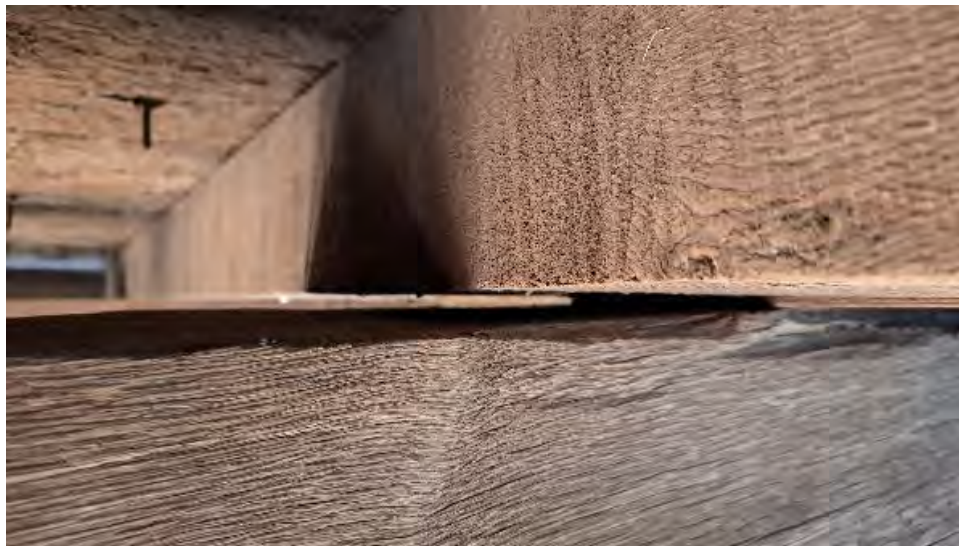
Figure 9-226: J9-5-S is not bearing on TB10.
