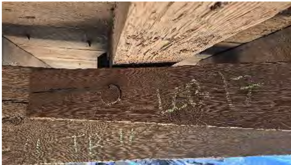
Figure 9-292: LCB-17 has minor cleaving on a spike to TB-11.
