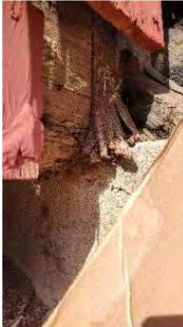
Figure 8-113: P4 is crushed for 6-inches from bottom.
