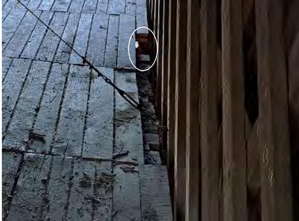
Figure 9-11: Floor decking Span 5, South side. Half of Plank 18 is missing.
