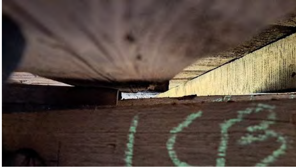
Figure 9-168: J6-2 has partial bearing on a packer at TB6.
