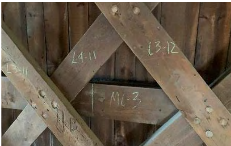
Figure 8-20: MC3 & MC4 splice location.
