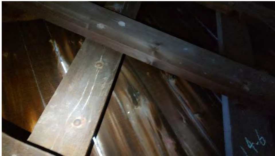
Figure 8-96: 5 is cracked through a dowel at the connection to L3-3.
