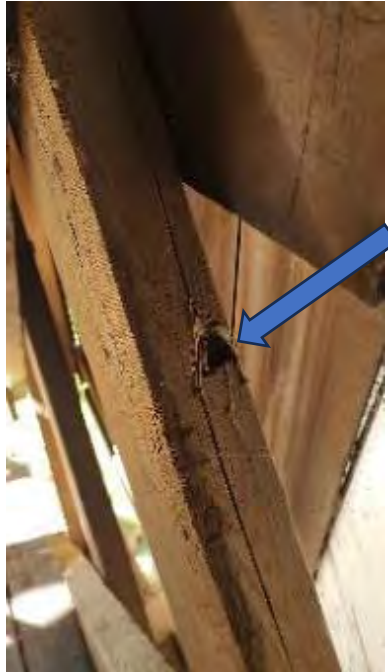
Figure 8-57: A tension crack (24-inches long) has propagated from at a knot on the top face of L1-20 below the middle chord.
