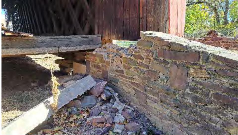
Figure 10-21: The North side of AB2 has approximate 10-foot length of stone wall destroyed for approximately half of its height.
