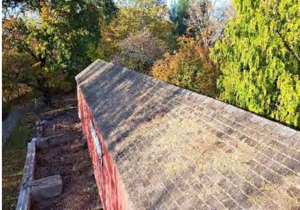
Figure 6-1: South side roof top of the Bridge with significant areas of fungal colonies present and shrinkage of the shakes.
