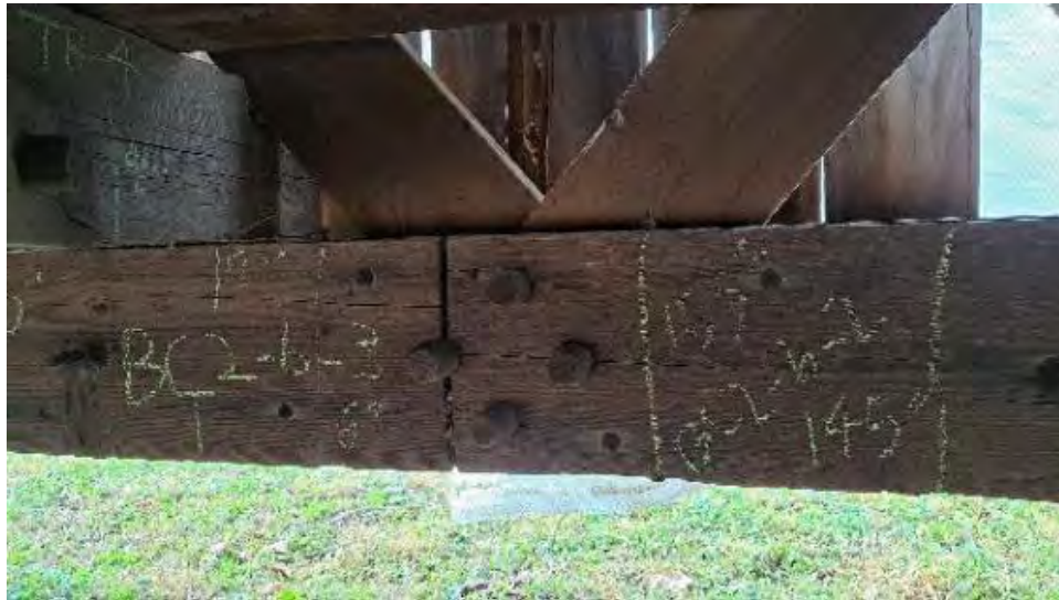
Figure 8-38 Some shrinkage checks exist to Bottom Chord 2 Ply B (BC2B) through the dowel holes at lattice connection, which is also the splice between chord segment 2 & 3 (BC2B-2 and BC2B-3).
