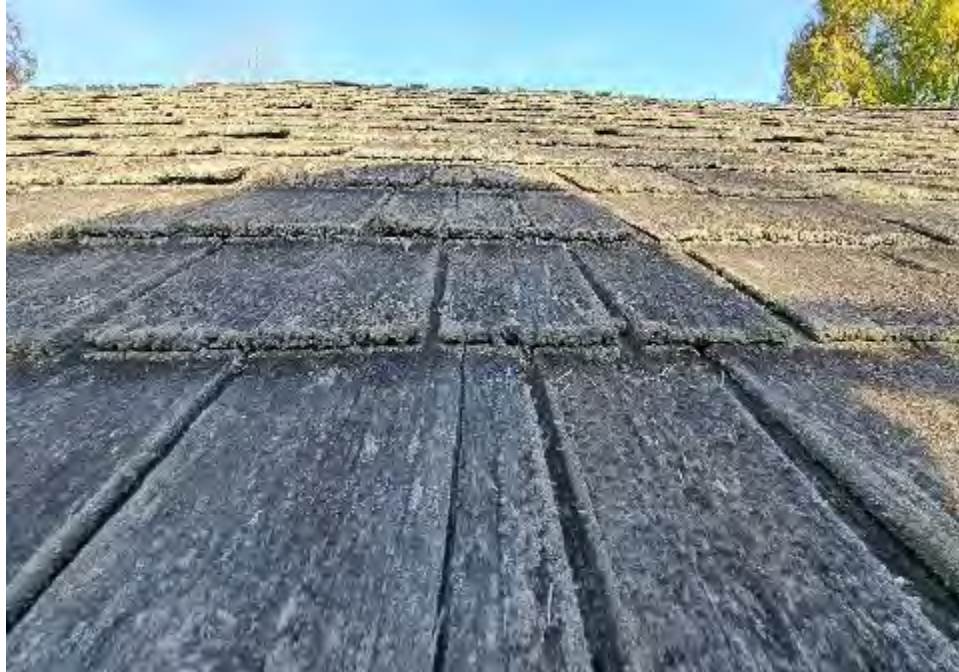
Figure 6-5: Severe weathering, shrinkage and fungal colonies across the roof.
