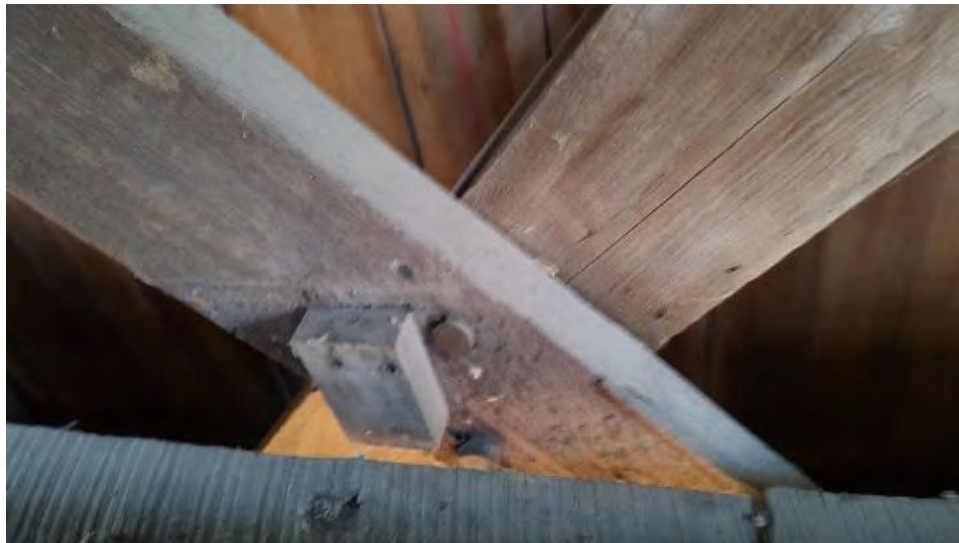
Figure 8-108: L4-20 has split extending from the dowels at the bottom chord.
