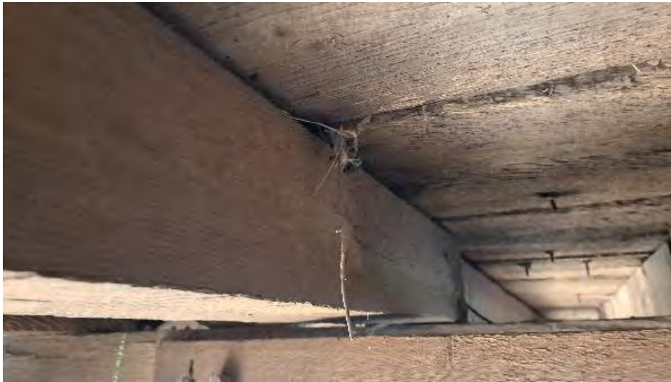
Figure 9-105: J2-7 is in fair condition.
