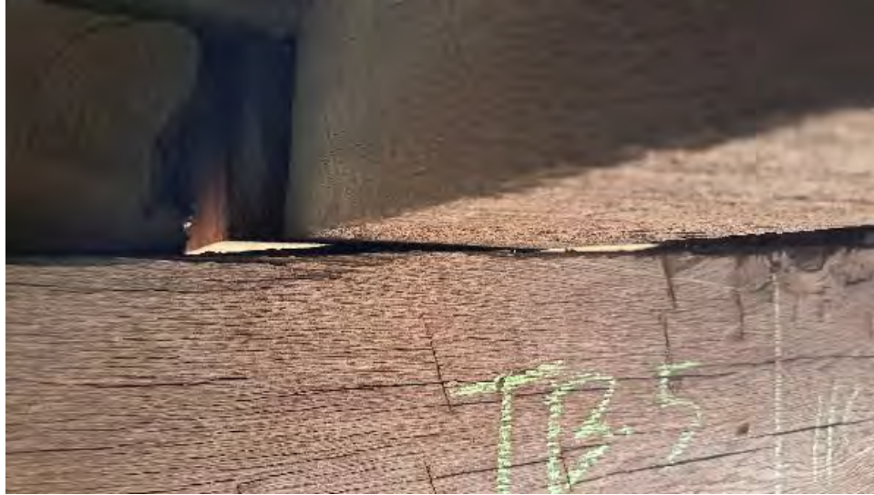
Figure 9-157: J5-5 is only bearing on the South edge over TB5.
