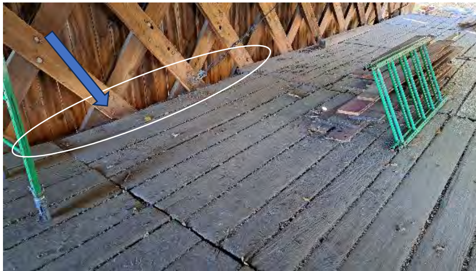
Figure 9-14: Floor decking Span 6, South side, where Plank 18 is missing.
