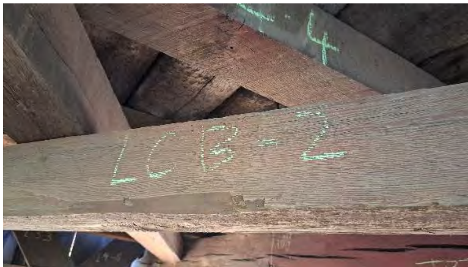
Figure 9-268: LCB-2 has some wane on the North side at midspan.
