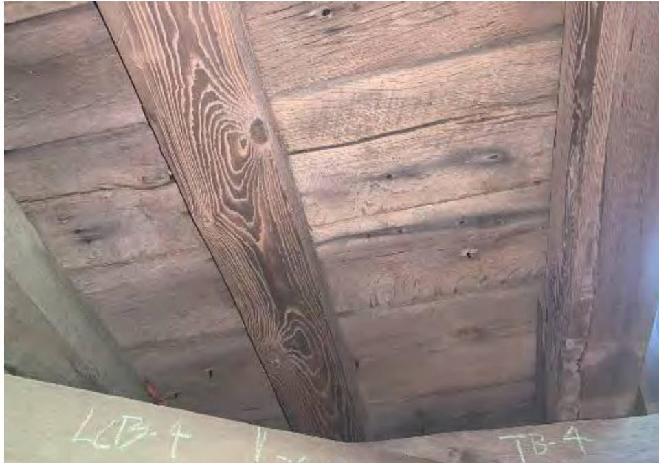
Figure 9-7: Lower layer of decking of Span 3 with termite damage.
