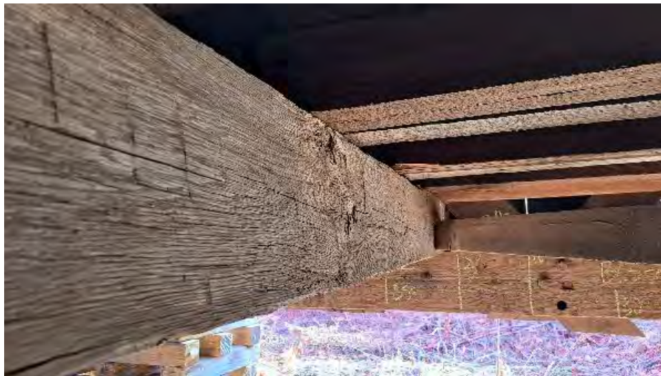
Figure 9-35: TB3 is twisted up to 3 degrees and is on a skew 18-inches out of perpendicular alignment with the bottom chords.
