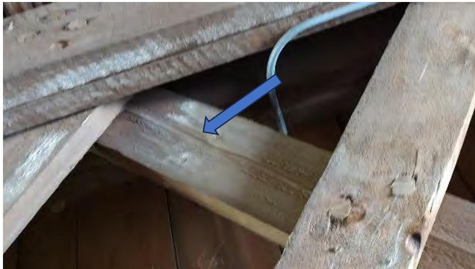
Figure 8-52: Large shrinkage checks exist through L1-10 and extend to the dowelled connection with the top chord.
