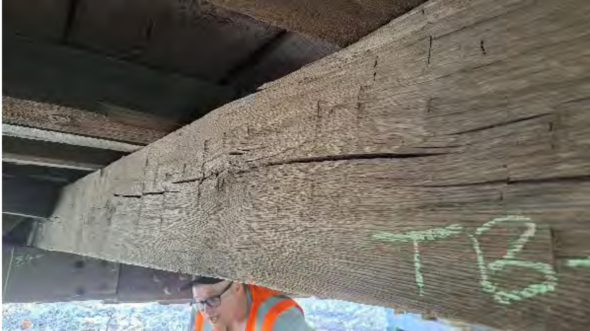
Figure 9-56: TB9 has shrinkage checks 2-inches deep and 3/8-inches wide on the AB1 side at the North end.
