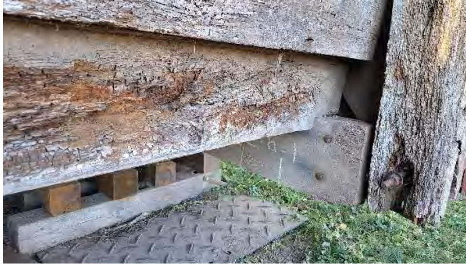
Figure 9-26: TB1 is on a skew as per original bridge site and has rotated or twisted up to 7 degrees on North end.
