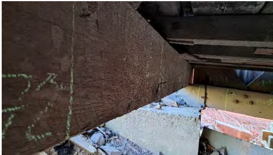
Figure 9-23: TB1 has some section loss (old split) on Abutment 2 side, North end on bottom corner for 12-inches.
