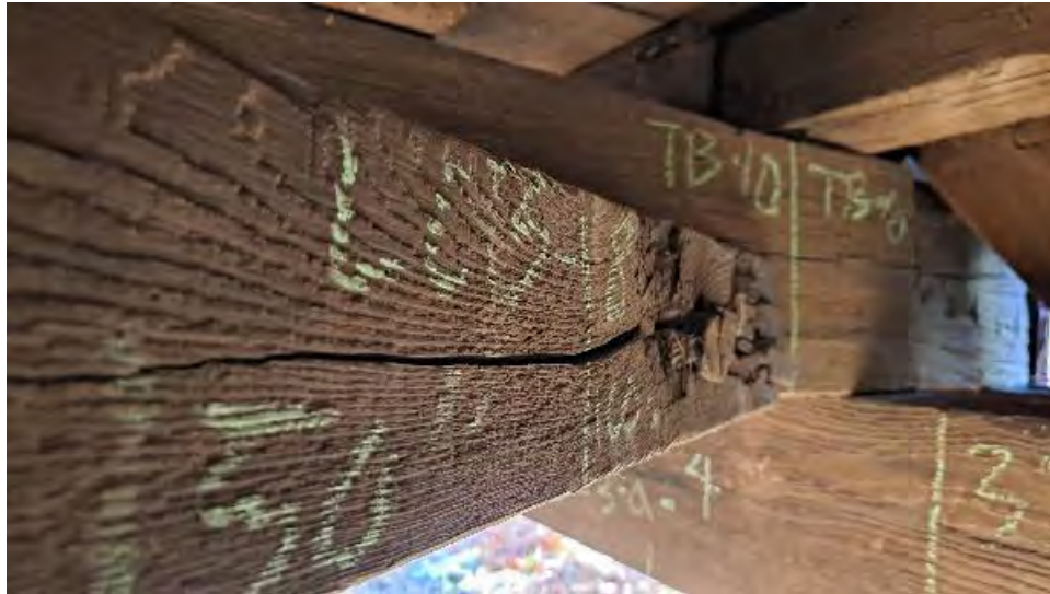
Figure 9-295: LCB-18 has major cracking and cleaving of dowel to TB10. The crack is 2-foot long and is on the AB2 face and meets vertical end crack seen on the bottom face.
