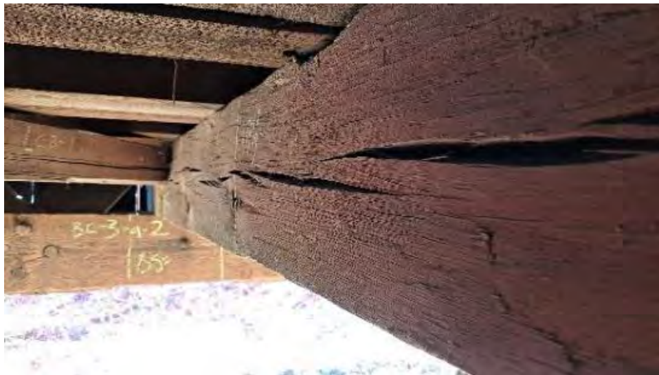
Figure 9-33: TB3 has large shrinkage checks on AB1 side that are up to 5/8-inches wide, for its full length.
