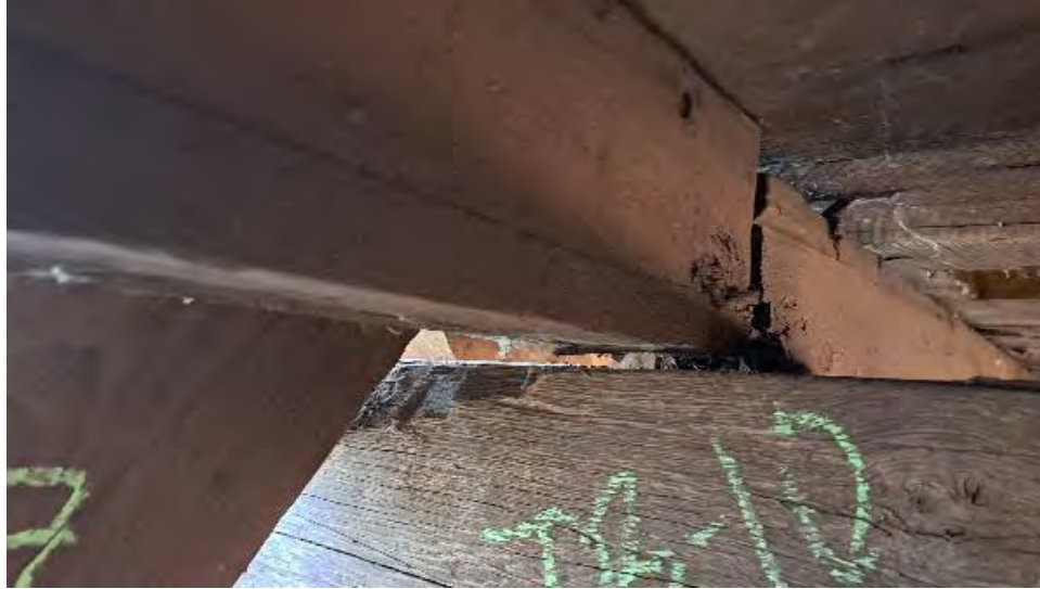
Figure 9-234: J10-1 is not bearing on TB10. Wane exists on its North bottom edge for 3-feet from TB11.
