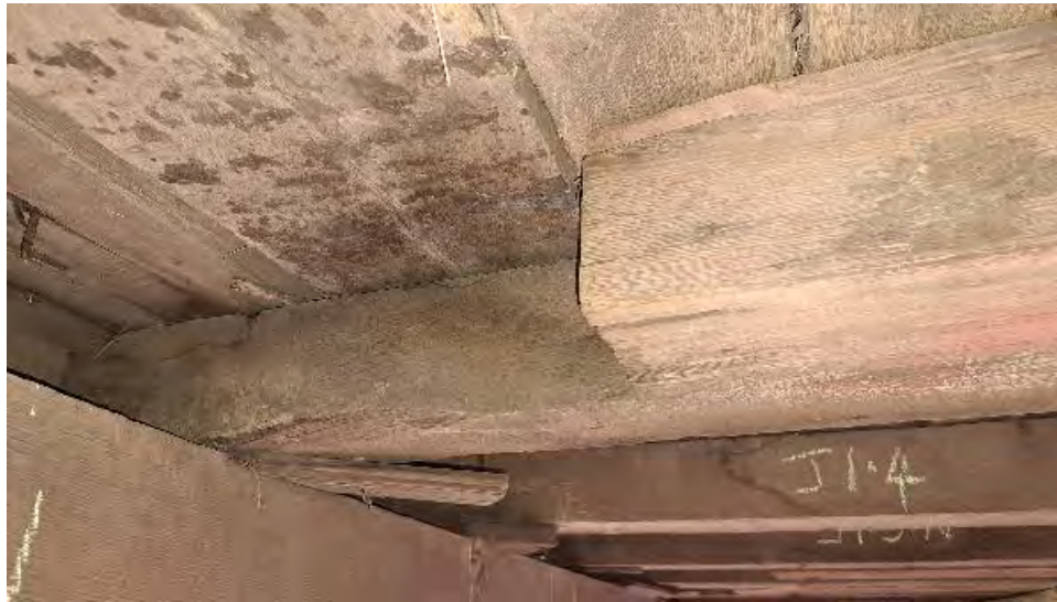
Figure 9-75: J1-3-N does not extend to TB1. J1-3-S is packed over TB1.
