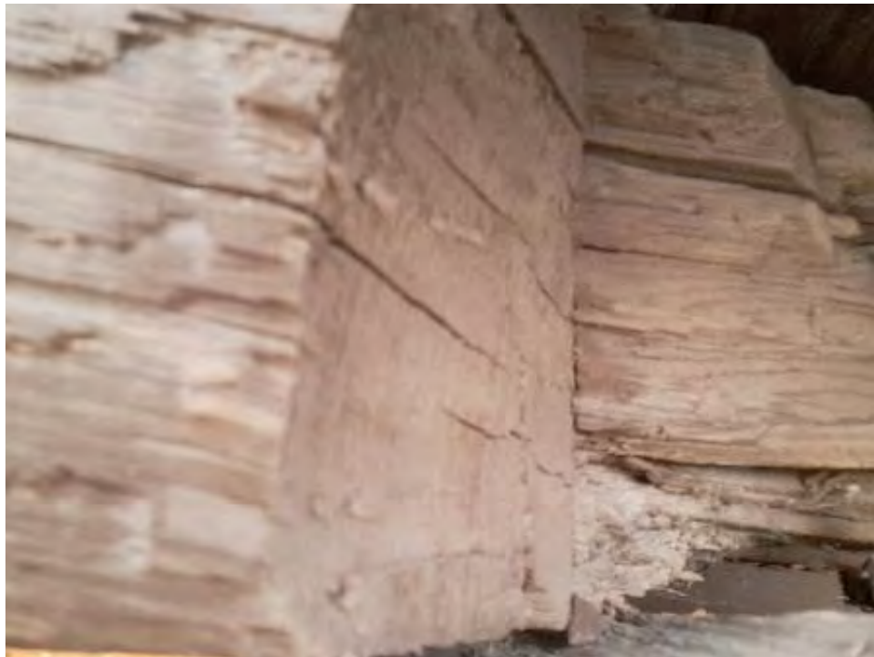
Figure 9-218: J9-1 has section loss at the bearing surface of TB10 end.
