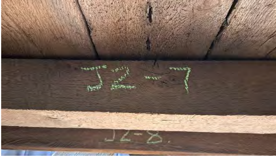
Figure 9-104: J2-7 is in fair condition.
